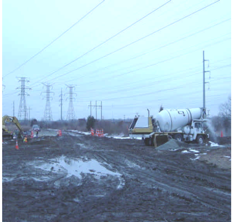
Trenching activities near sta. #1063. Concrete truck was observed washing out in a contained area.
