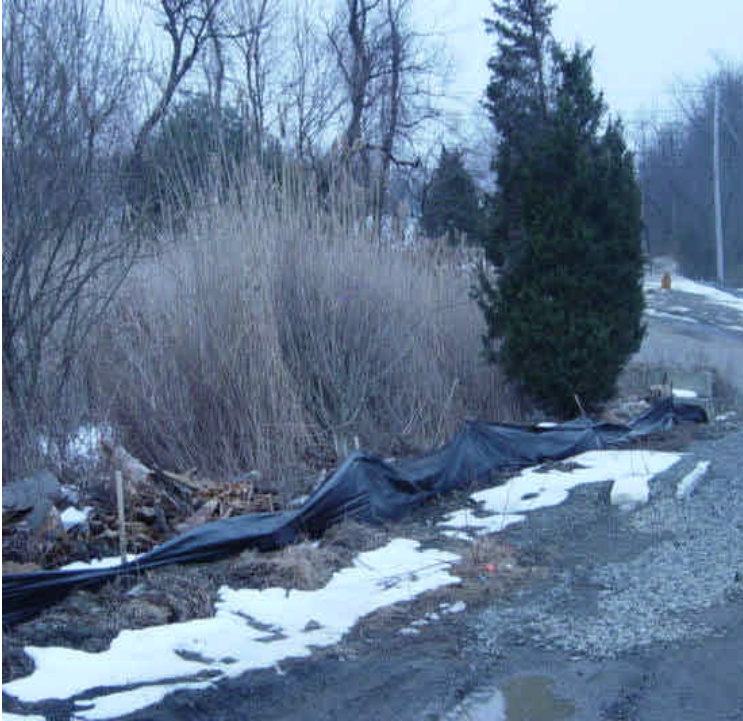
Brush and stumps have been piled in a resource area beyond the silt fence. The gate at Naugatuck Ave has been removed and also remains stored in the adjacent resource area. Erosion controls are degraded here and need repair.
