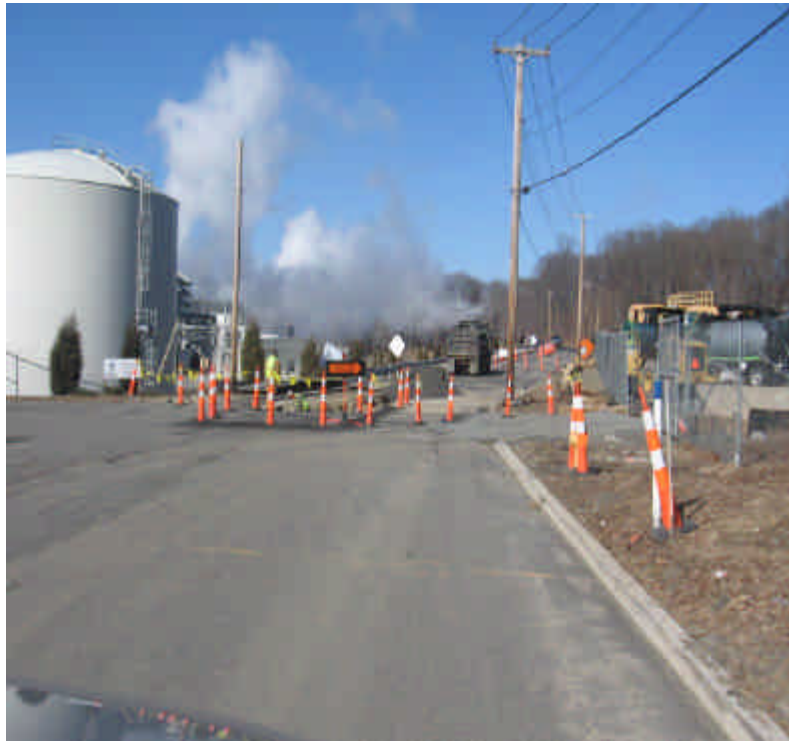
View of trenching activities on Shelland St. adjacent to the entrance to Milford lay-down yard. No sediment tracking was observed from the yard onto Shelland St.
