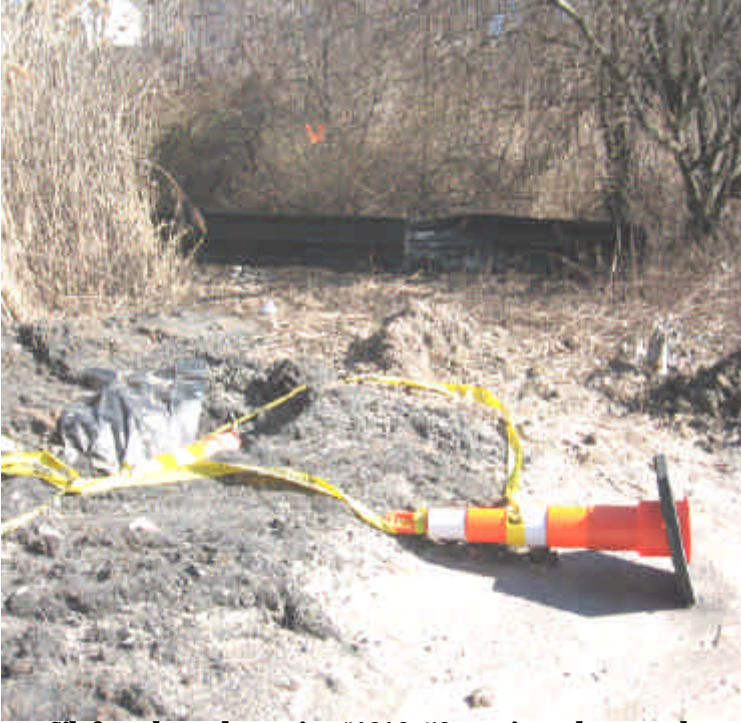
Silt fence located at station #1016+50 remains to be properly installed (toed-in). A resource area is adjacent so maintenance is necessary.
