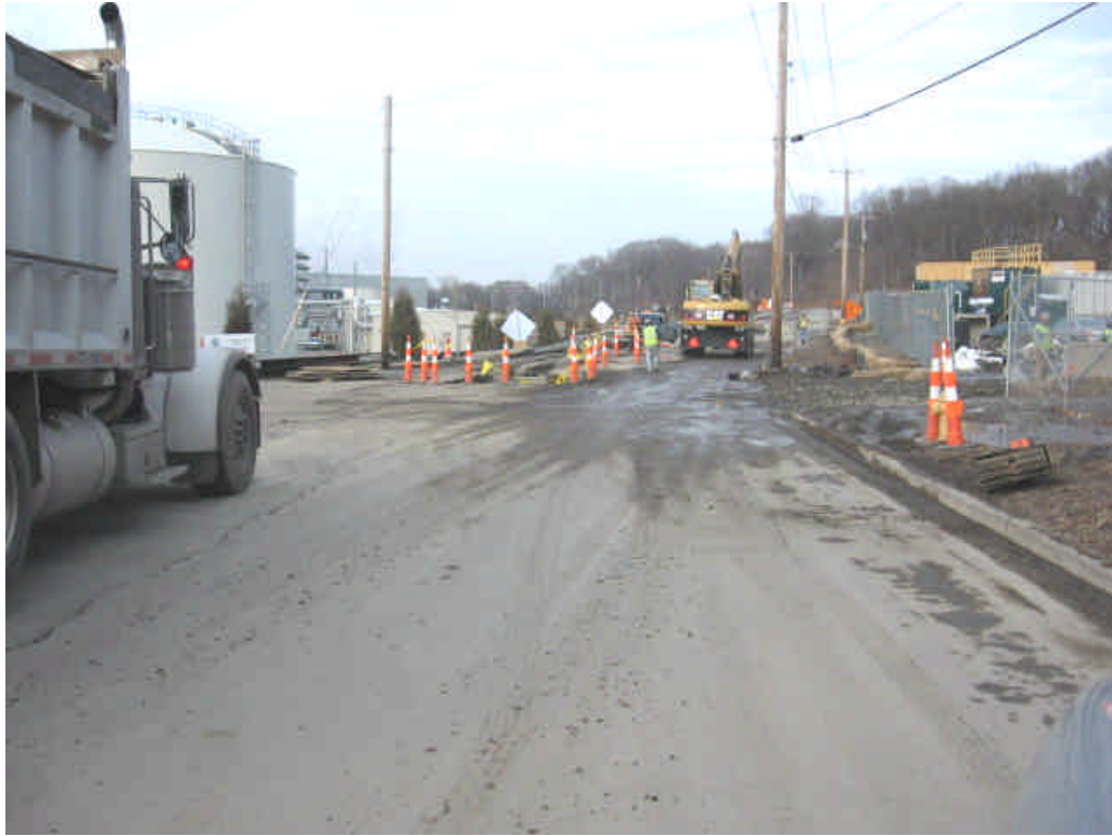
Photo of trenching activities on Shelland St. near the entrance to the Milford lay-down yard. Minimal tracking from the yard was noted.
