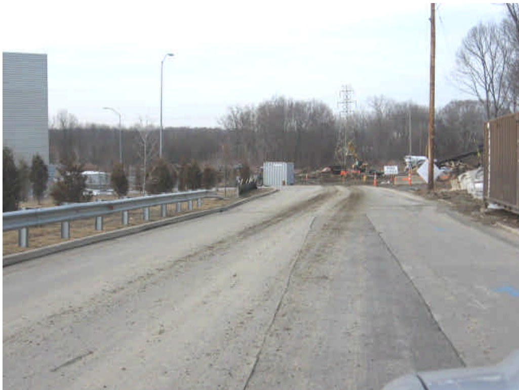
Sediment tracking from the unpaved portion of Shelland St. was apparent on the remainder of the roadway. A stone construction entrance may be necessary to reduce sediment tracking in this area. Sweep the roadway on a regular basis.
