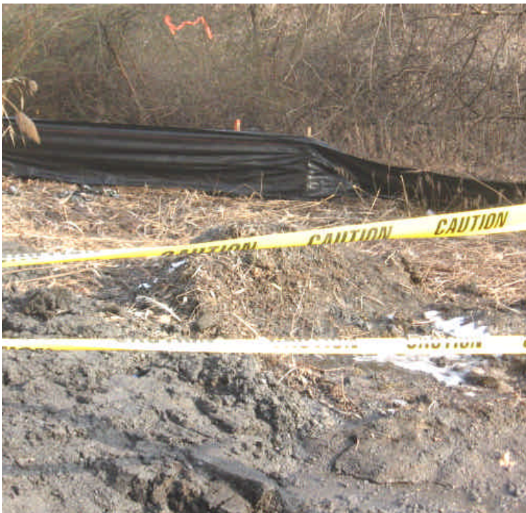
Silt fence was in place between trenching activities and the adjacent resource area at #1016+50, but it needs to be properly installed (toed-in).
