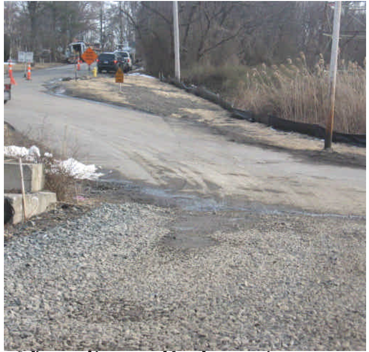
Sediment tracking was noted from the construction entrance at station #1053 onto Naugatuck Ave. The construction entrance appears clean but the roadway should be swept.
