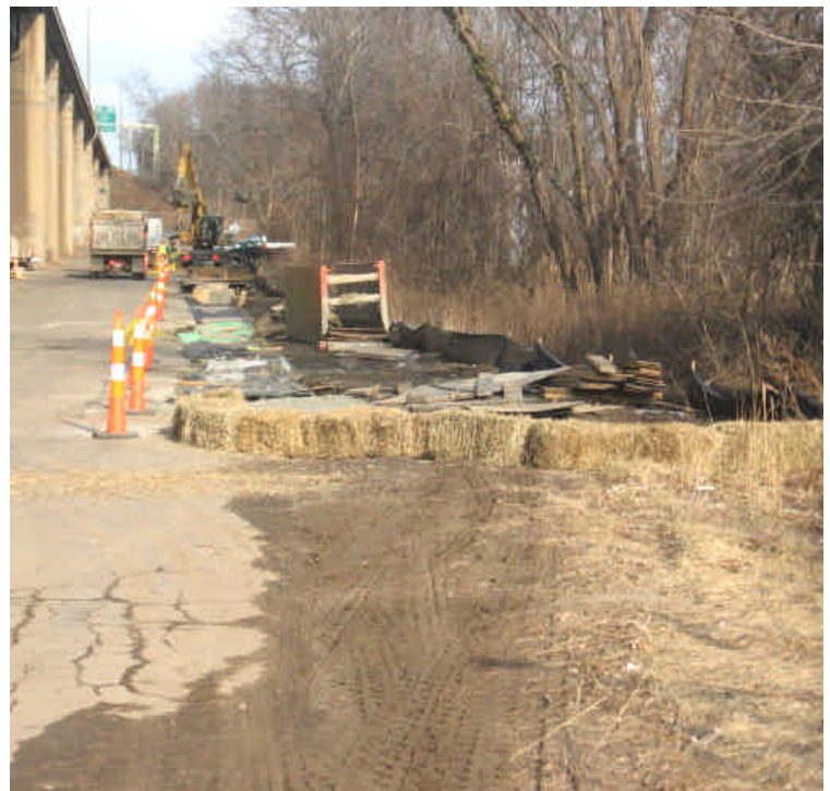
Haybales have been proactively installed to control sediment migration at station #1017. The sediment seen in the foreground of the photo was present prior to the construction activities.
