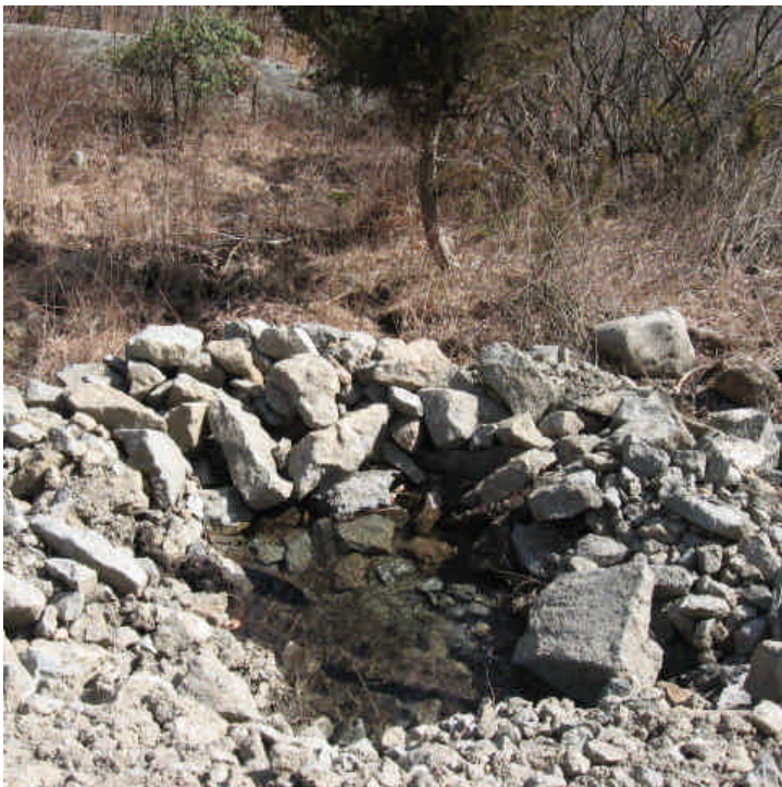
Cow Path Lane: Additional stone sediment traps were installed along the access road.
