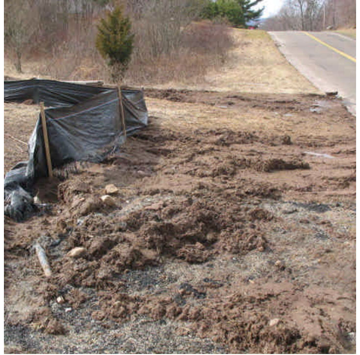
Old Lane Rd: Silt fence was installed to protect the area downgradient of the access road, but it does not protect the catch basin from the adjacent, exposed soil and run-off.
