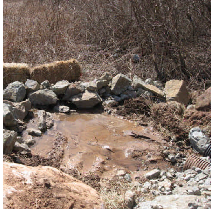
Tom Swamp/Arrow Rd: Sediment was present within the sediment trap at the outlet of the smaller culvert during the inspection. Water exiting the stone trap was clean. Restore capacity if necessary.
