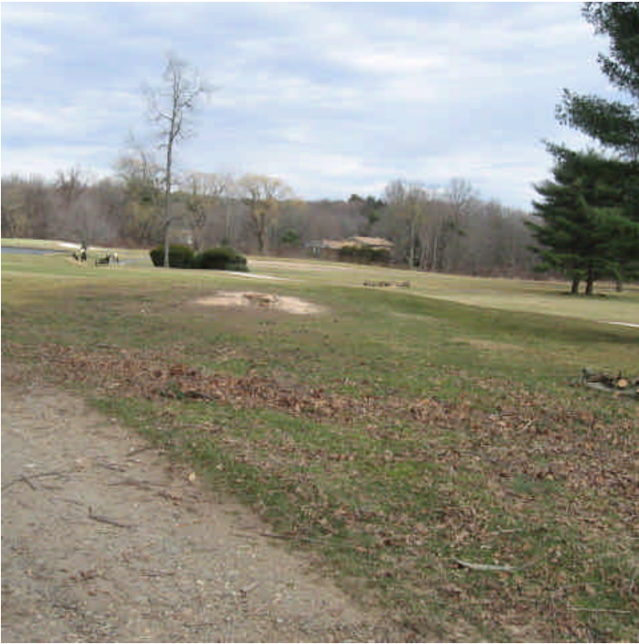
Oak Lane Country Club (Woodbridge): Large trees were cut and removed carefully from the golf course area.
