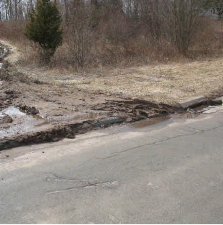
Old Lane Rd (Hamden): The entrance to the overhead ROW access was still very muddy this week. There is still no drop inlet protection here and turbid water was observed entering the catch basin.
