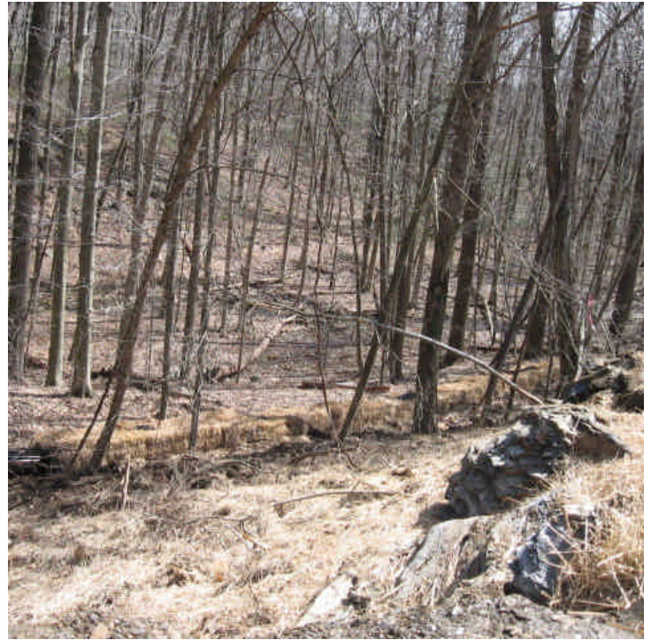
Cowpath Lane: A double line of haybales and silt fence were installed upgradient of the wetland system located off the ROW, and below a recently graded pad.
