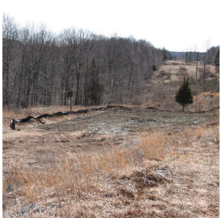
Cow Path Lane: Additional silt fence was added along the new crane pads and throughout the ROW.
