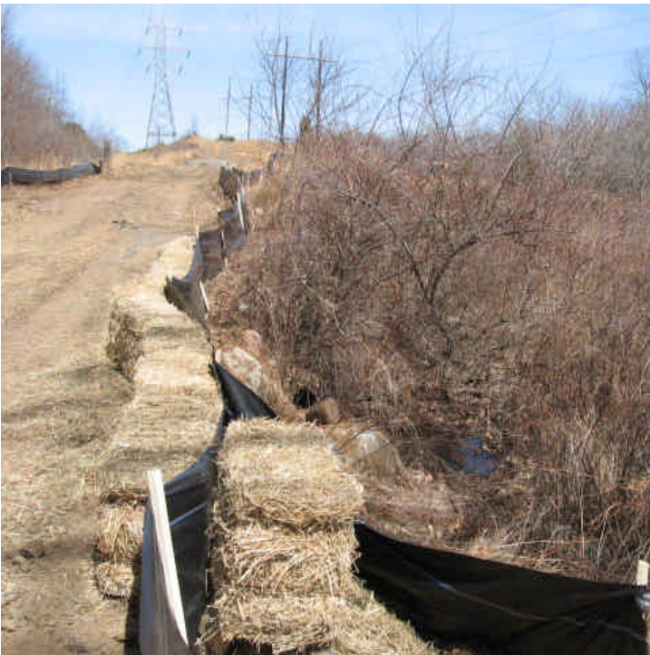
SCCRWA (Glen Dam): View of the haybales and silt fence installed at the wetland area located along the access road.
