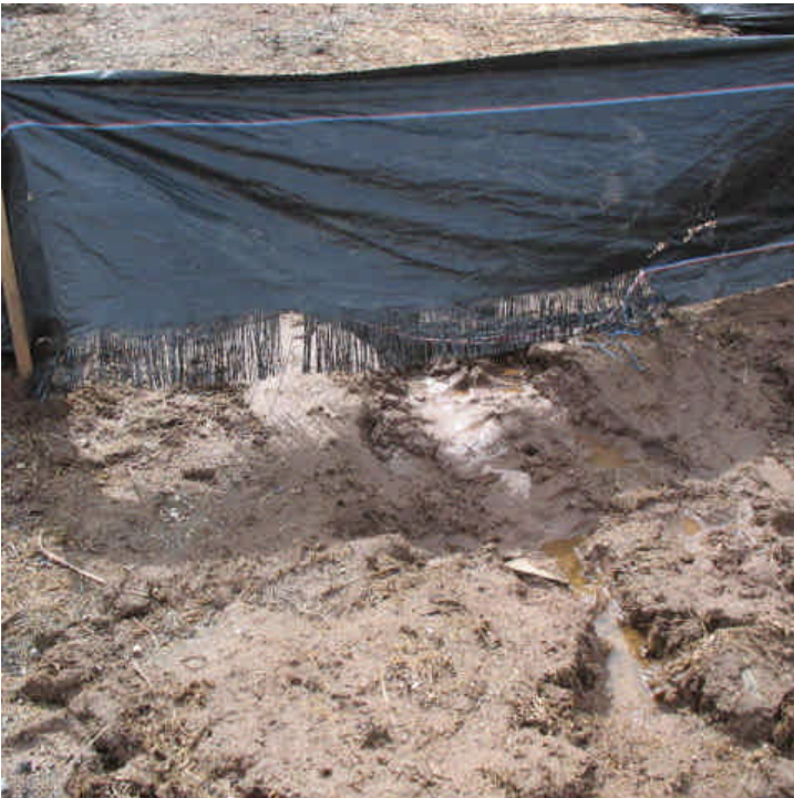
Old Lane Rd: Some areas of silt fence were ripped and not toed in. A small gully has formed and turbid water is flowing toward the road.
