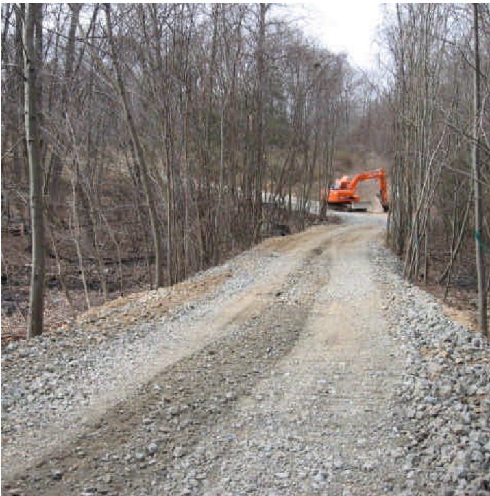
East Rutland Rd. (Milford): View of the constructed access road. Road building was actively occurring during the inspection.
