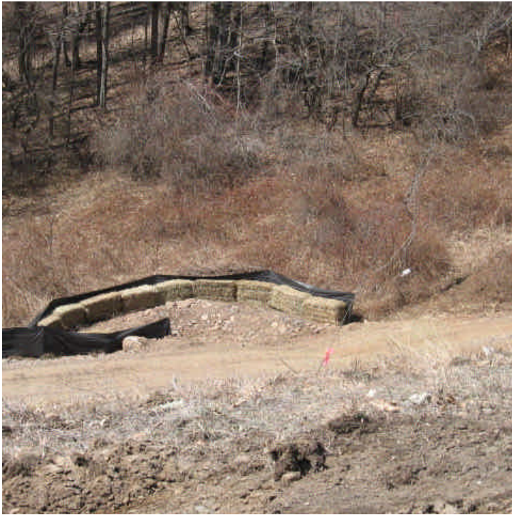
SCCRWA (Glen Dam): Additional water bars were added along the access road. Haybales and silt fence were installed at the outlets.
