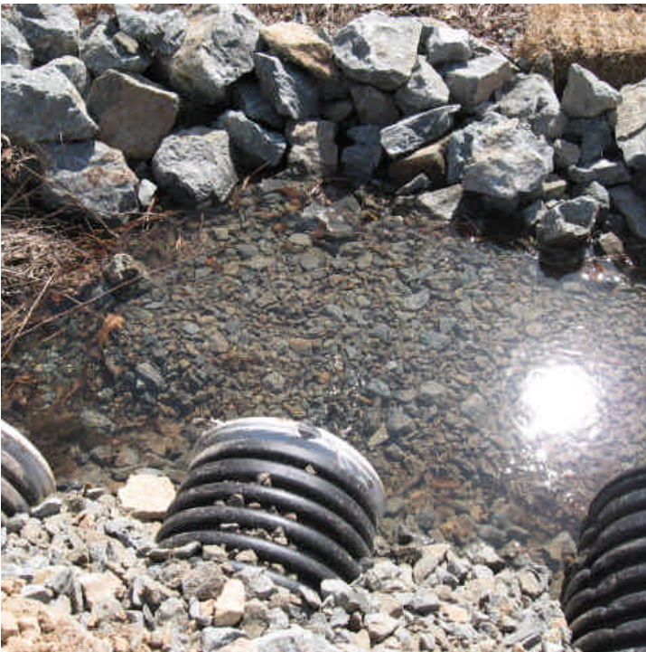
Tom Swamp/Arrow Rd: A triple culvert crossing was constructed within the access road at the stream crossing. Water at the outlet was clear.
