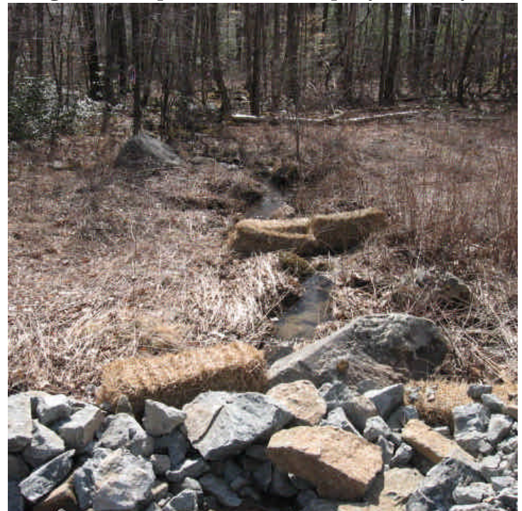
Tom Swamp Rd/Arrow Rd: Haybale check dams were installed down-gradient of the crossing. Although some sediment was present within the channel, it had not migrated beyond the check dams.
