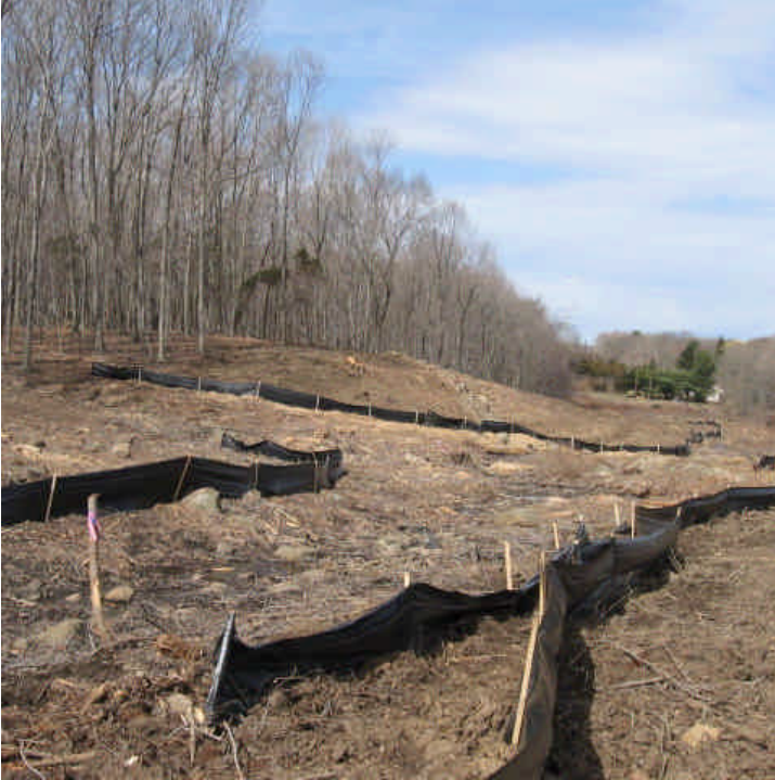
JCC (Woodbridge): Additional silt fence was installed along the wetland area here. All other silt fence remains intact.
