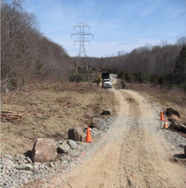
Tom Swamp/Arrow Rd (Hamden): View of the constructed access road and clearing within the ROW.
