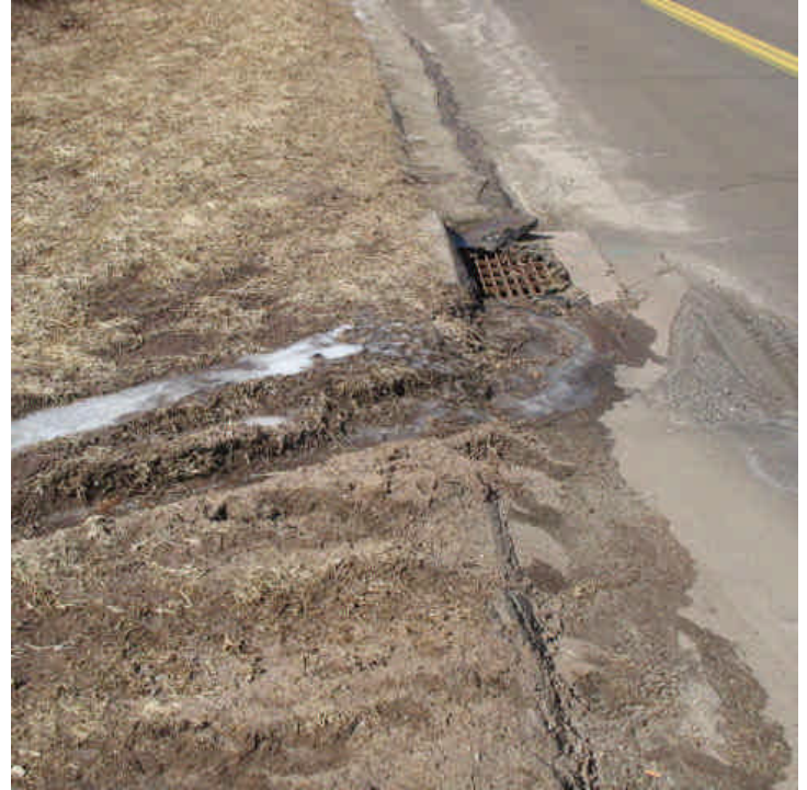
Old Lane Rd: The catch basin at the entrance of the overhead ROW did not have curb drop inlet protection and run-off has a direct path to it.
