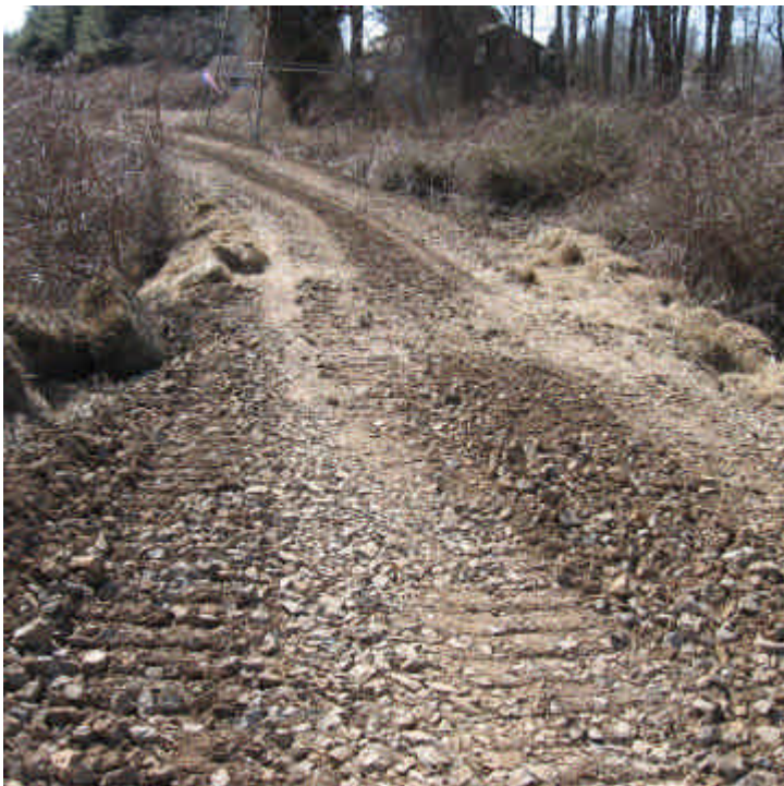
Treat Lane (Orange): Stone was added as a stabilization measure along the access road at the wetland/stream crossing.
