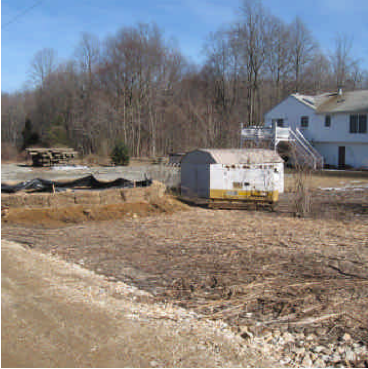
Dogwood Rd (Orange): Controls were breached at the secondary dewatering basin here last week, but sedimentation is not an issue.
