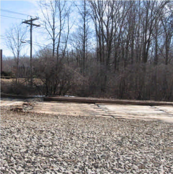
Rimmon Rd (Woodbridge): A stone and timber mat crane pad was installed near the wetland/stream in this location.
