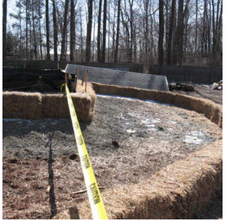
Whealers Farm Rd (Milford): Foundation drilling/poring has begun at this location. A dewatering basin and secondary line of haybales was installed proactively.
