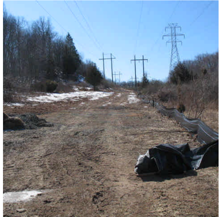
Old Lane Rd: Work within this section of overhead ROW appears to be complete at this time. Silt fence remains intact.
