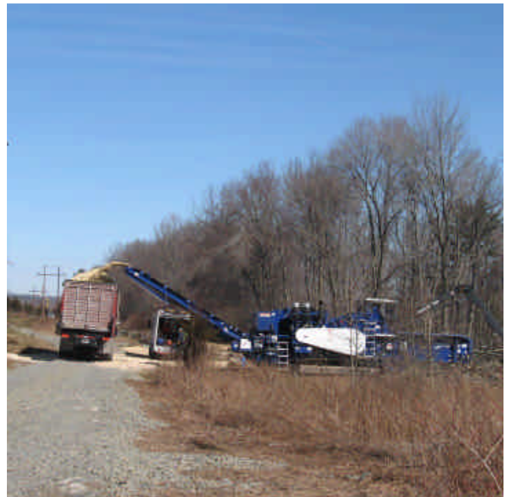
Pease Rd/JCC (Woodbridge): Chipping and stockpiling of timber continued in the ROW this week.
