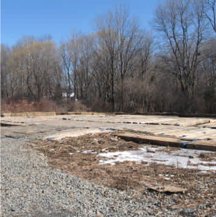
Manville Rd (Woodbridge): The stone access road was extended to the second proposed structure within the wetland here. A timber mat crane pad with haybale perimeter controls was also in place.
