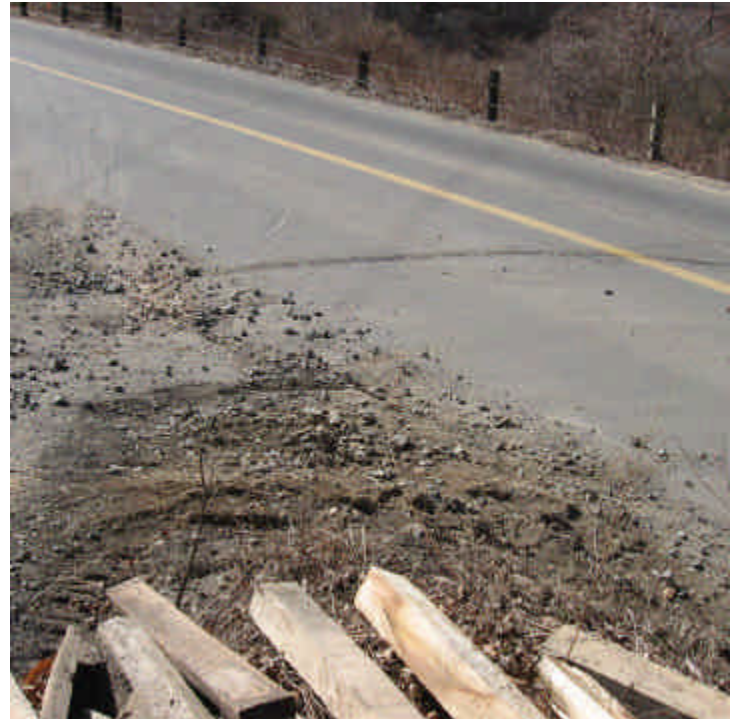
Pease Rd (Woodbridge): Due to heavy vehicle traffic and the sharp turn at the access road, sediment tracking continues to be an issue here.
