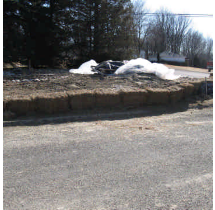
Saddle Ridge Rd/Harborview Rd (Orange): Foundation work has begun here. Haybales were added to control sediment at this roadway intersection.
