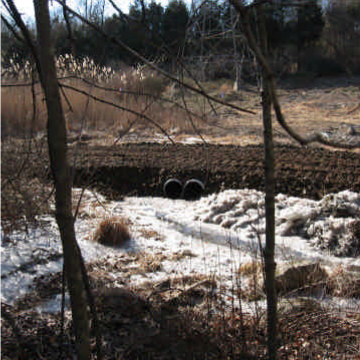
Cowpath Lane (Woodbridge): Clearing and road building has begun within the portion of ROW accessed from Cow Path Lane. Due to high water levels within the wetland and intermittent stream flow here, temporary culverts were installed along the access road.
