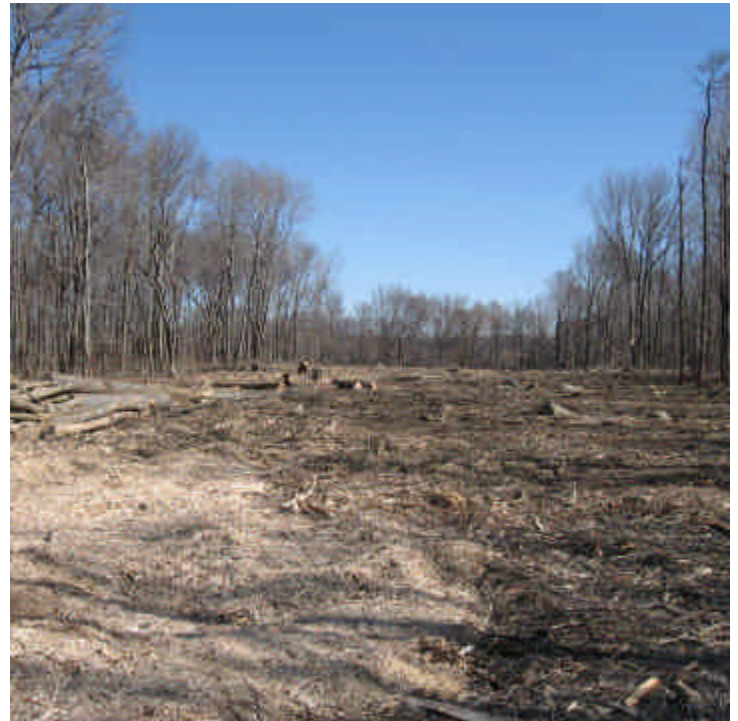
Pease Rd/JCC (Woodbridge): The majority of the clearing necessary for the new section of ROW (JCC bypass) is complete.
