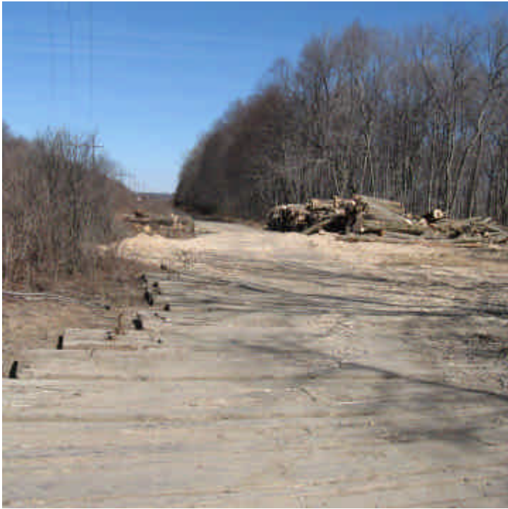
Pease Rd (Woodbridge): Timber mats have been extended along the access road here to prevent rutting.
