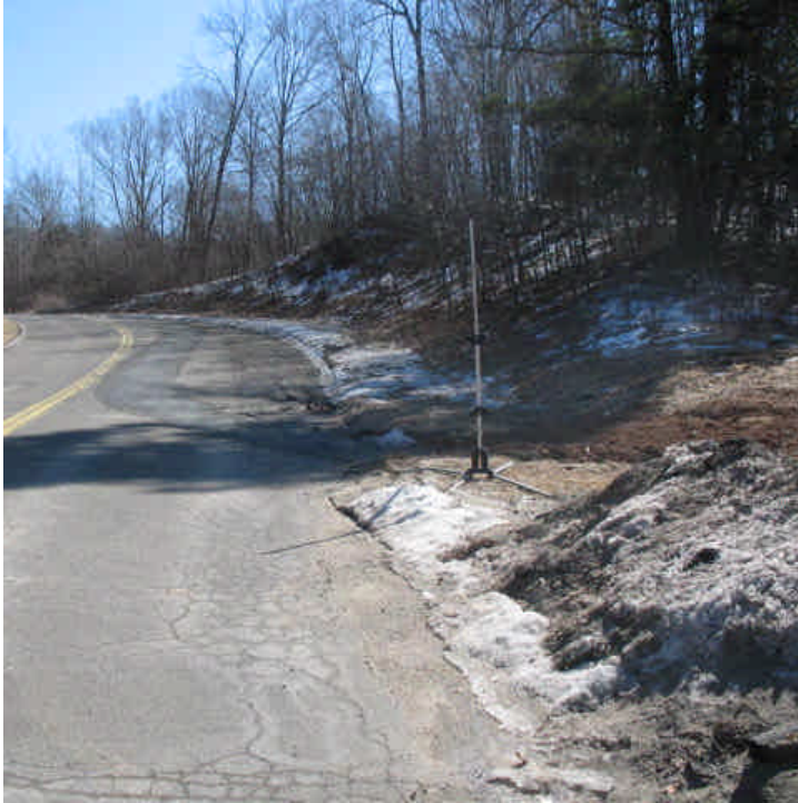
Old Lane Rd: View of the underground line transitioning from the roadway into the overhead ROW. The underground conduit is in place.
