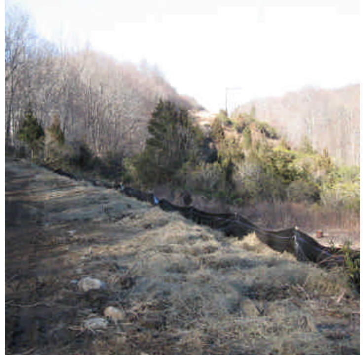
Cowpath Lane (Woodbridge): Silt fence was installed along the access roads and mulch was in place on disturbed slopes.
