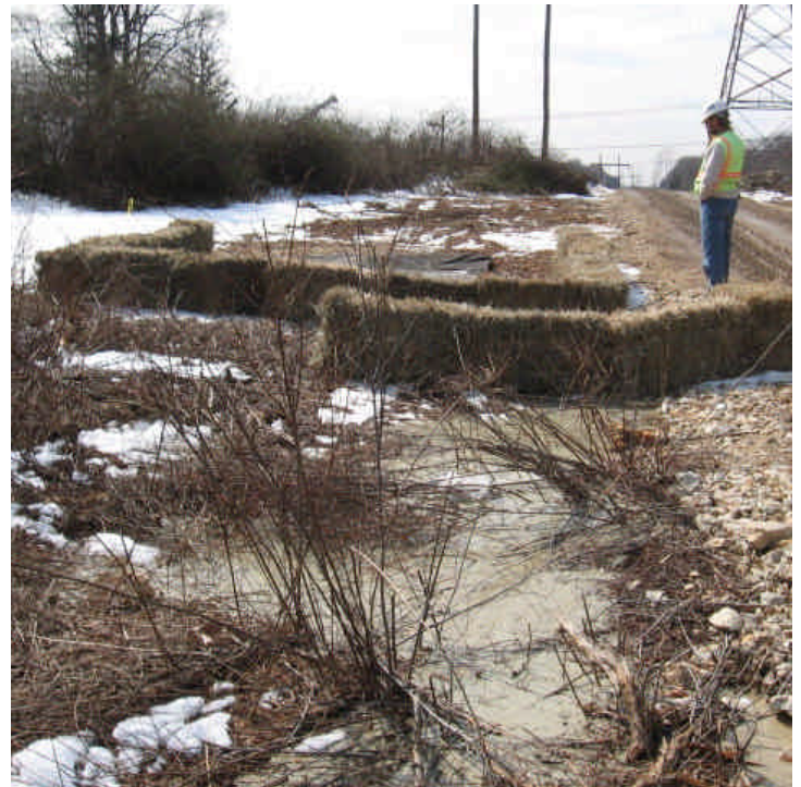
A second dewatering area, consisting of a filter bag and two lines of haybales, was used as an alternative to the primary basin. Slurry/sediment had breached the controls here but did not reach the wetland area. Solutions and additional controls were being discussed.
