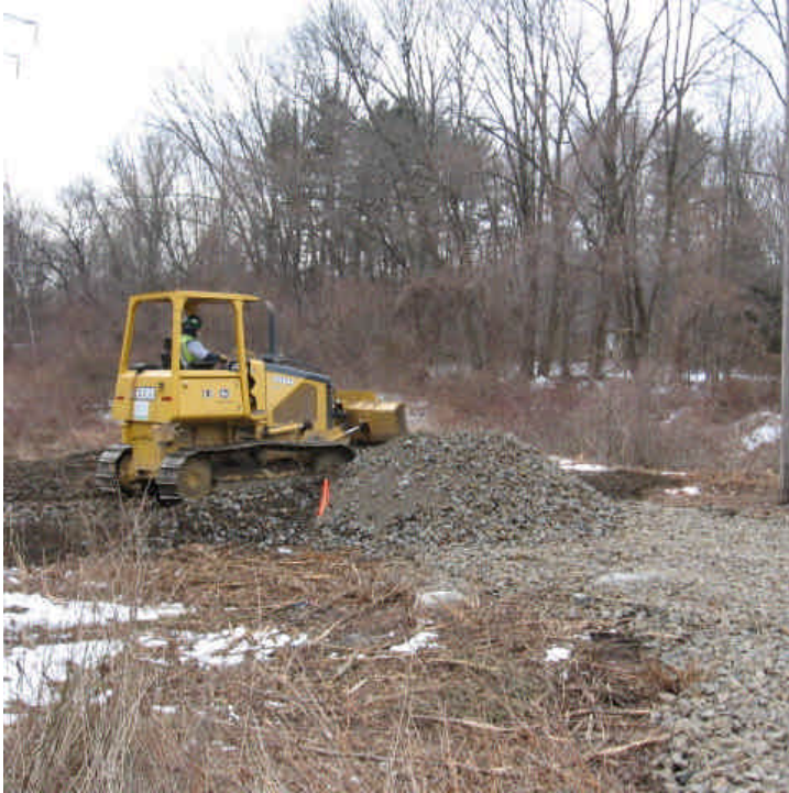
View of the clearing and access road construction off Rimmon Road in Woodbridge. Haybales had been delivered for installation near the wetland here.
