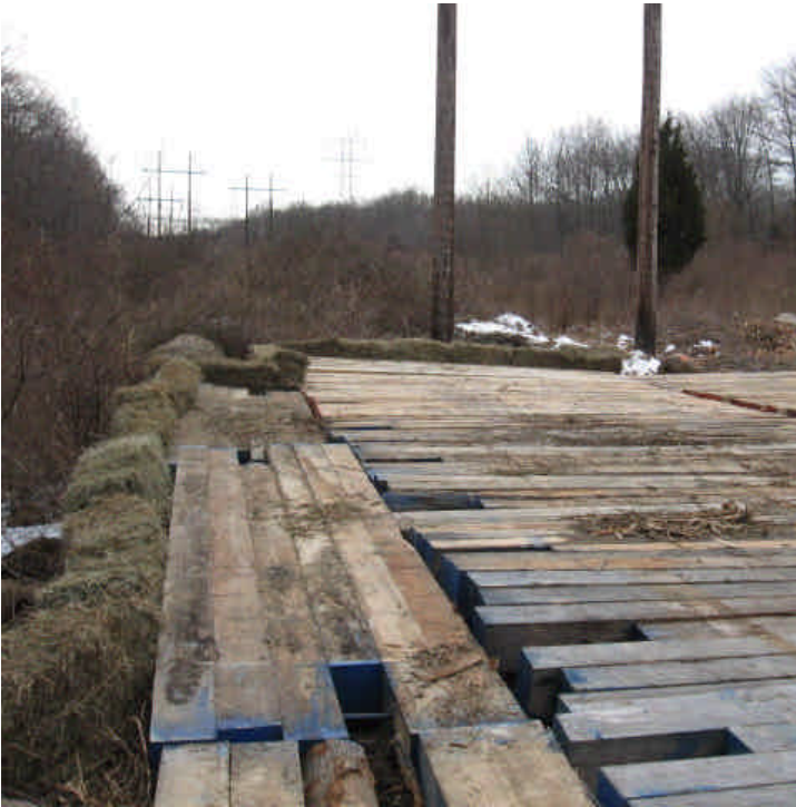
View of the crane pad and haybales installed within the wetland area off Marville Road (west).
