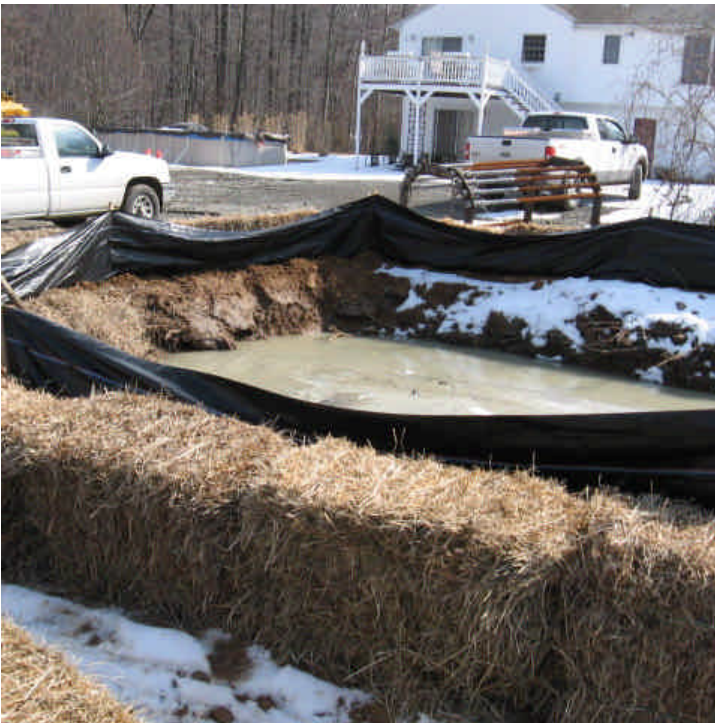
View of the primary dewatering basin within the ROW off Dogwood Rd (east). Active dewatering was occurring at the time of inspection.
