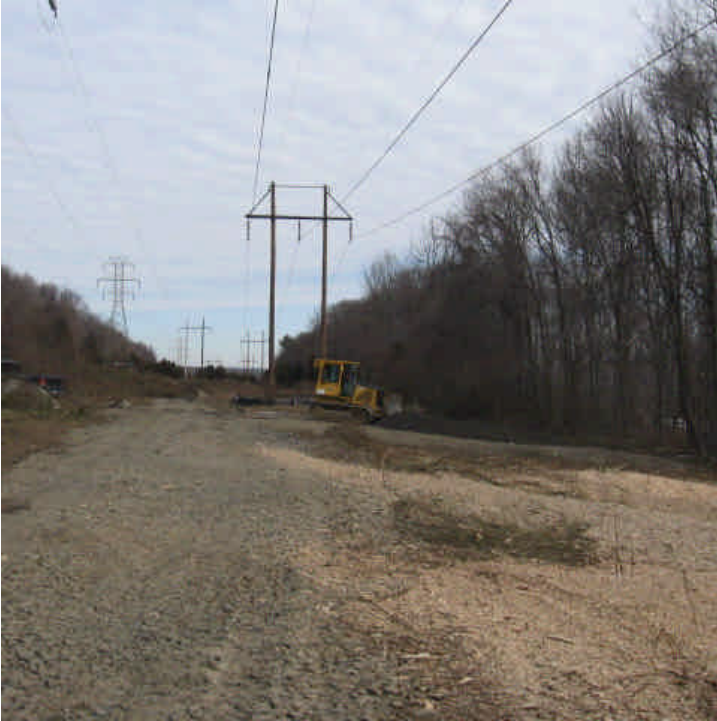
View of the new clearing and stone access roads constructed within from the the ROW accessed from Pease Road.
