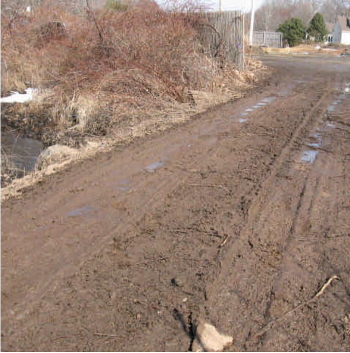
The access road crossing the wetland off Treat Lane was very muddy this week. Additional stabilization measures may be needed here.
