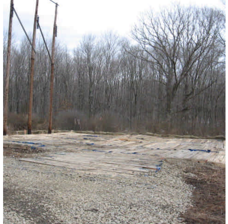
A timber mat and crane pad were installed within the wetland off Manville Road (east). Hay bales were placed along the crane pad, at the undisturbed wetland edge
