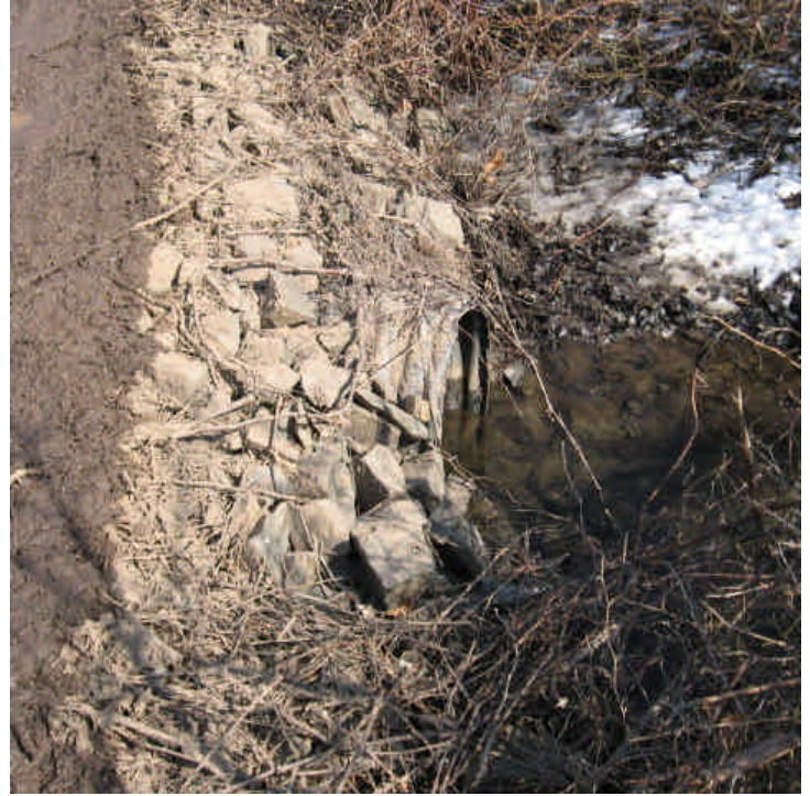
Some sediment from the muddy access road had migrated toward the stream channel here (Treat Lane). Erosion controls are required here per the D&M plan (especially with warming temperatures).
