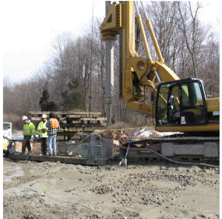
View of the foundation drilling/pouring near the wetland off Dogwood Rd (east).
