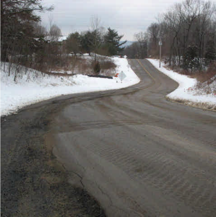
View of backfilling and trench patching/paving associated with the 115-kV underground work (Section 2b) in Old Lane Road.
