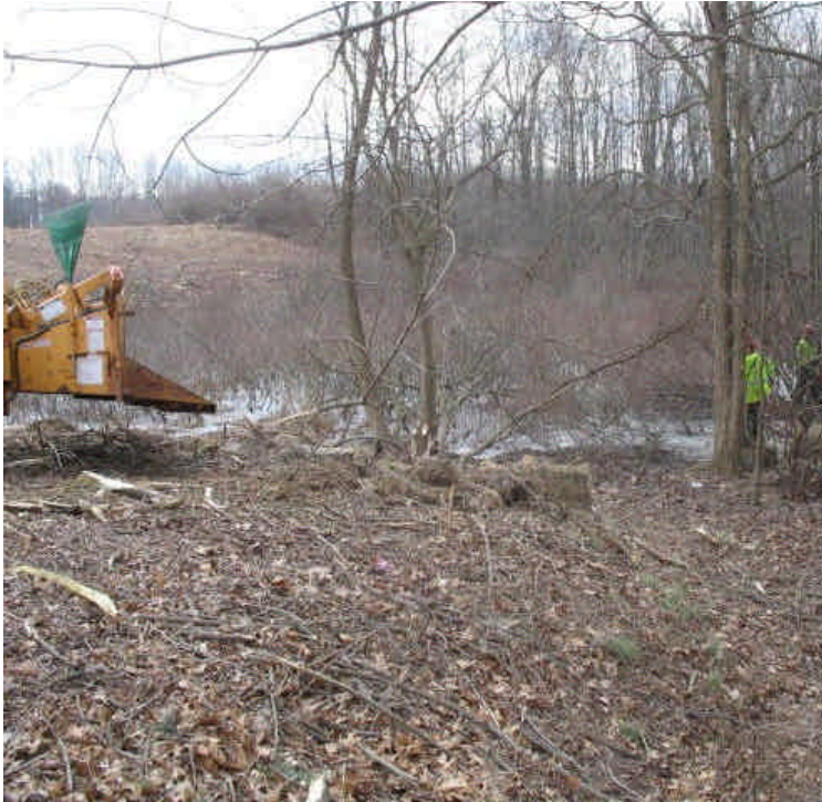
Clearing was occurring in wetlands within the ROW moving south from Carpenter Lane and Beseck SS.
