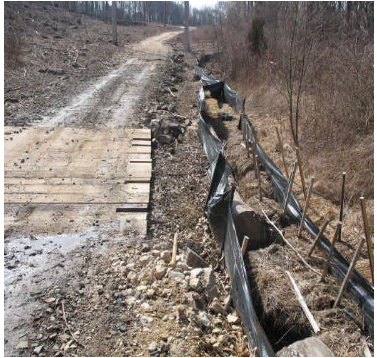
Silt fence and controls are degraded along the access road off High Hill Rd. Haybales were added to reinforce controls. Run-off issues were not observed.
