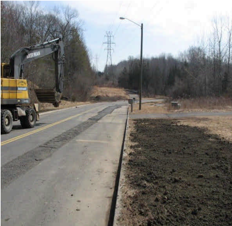
Topsoil is being applied and graded along Old Farms Rd. in an effort to repair ruts. Crews were also working to clean sediment from the gutters
