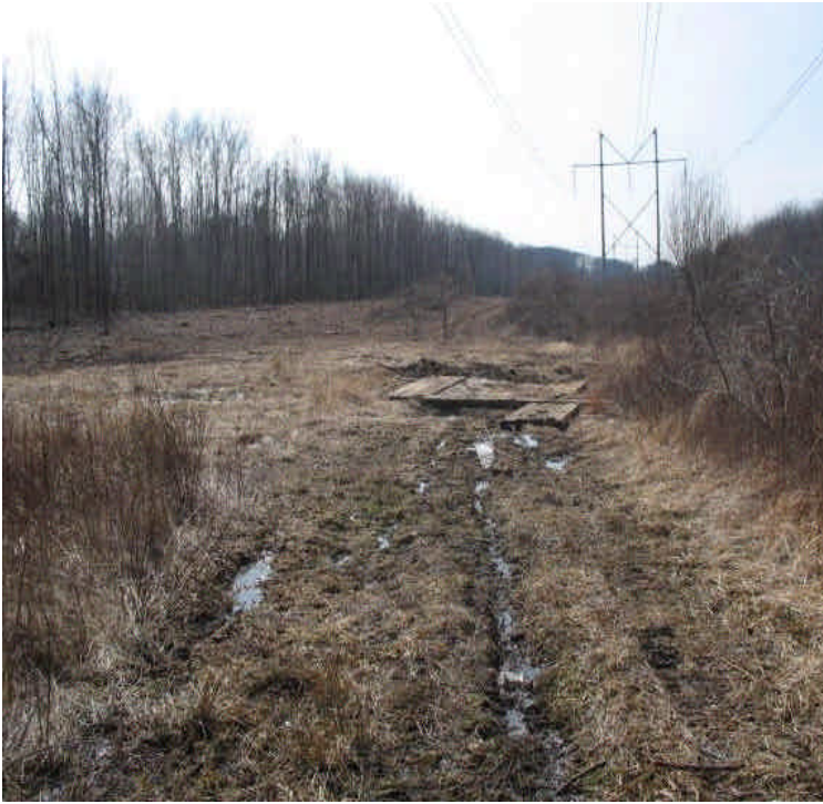
ROW clearing and timber mat installation south of Beseck SS off High Hill Rd. Low growth vegetation was retained within the wetlands here appropriately. Controls may be needed if soil becomes disturbed.
