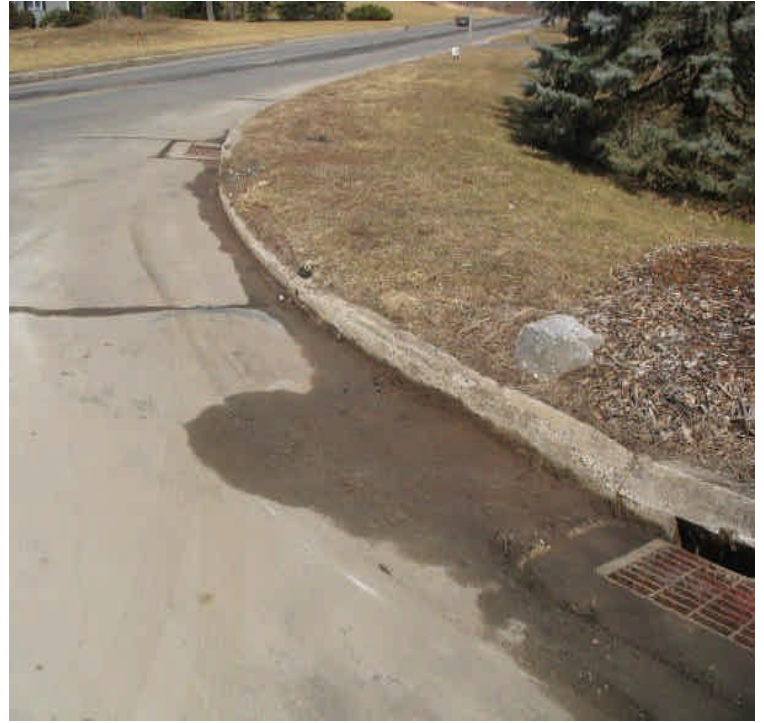
Efforts to sweep and remove sediment accumulation along Old Farms Rd. were noted.
