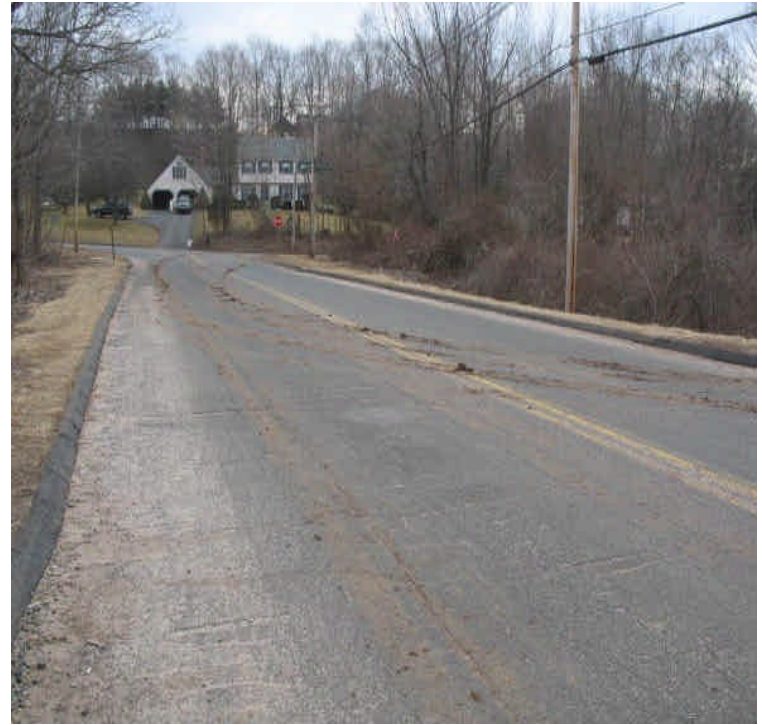
Sediment tracking was noted on Carpenter Ln. resulting from clearing crews accessing the ROW. Sweep the roadway on a regular basis and install a construction access pad as necessary.
