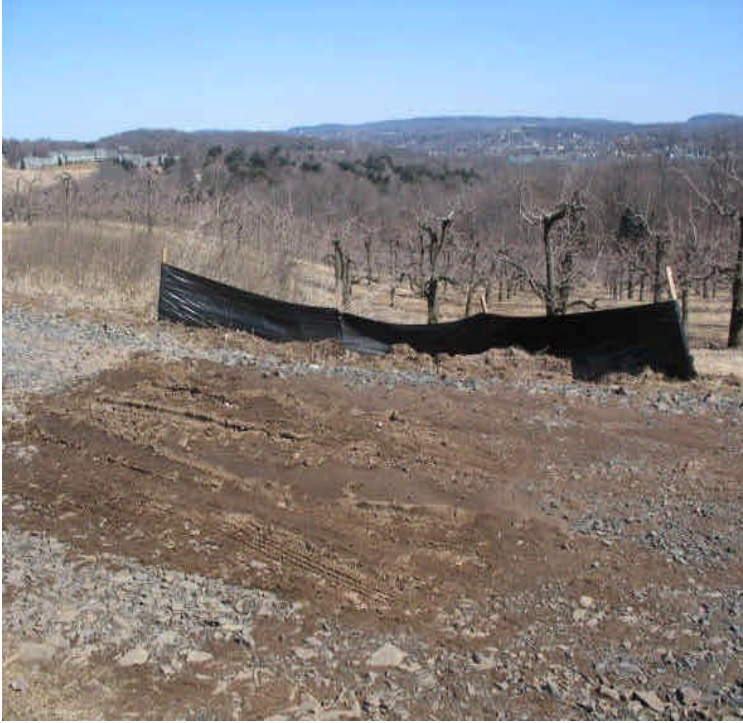
Sediment accumulation was noted near some of the controls within the apple orchard off Mansion Rd. Pull back sediment to remove stress on the controls when needed.
