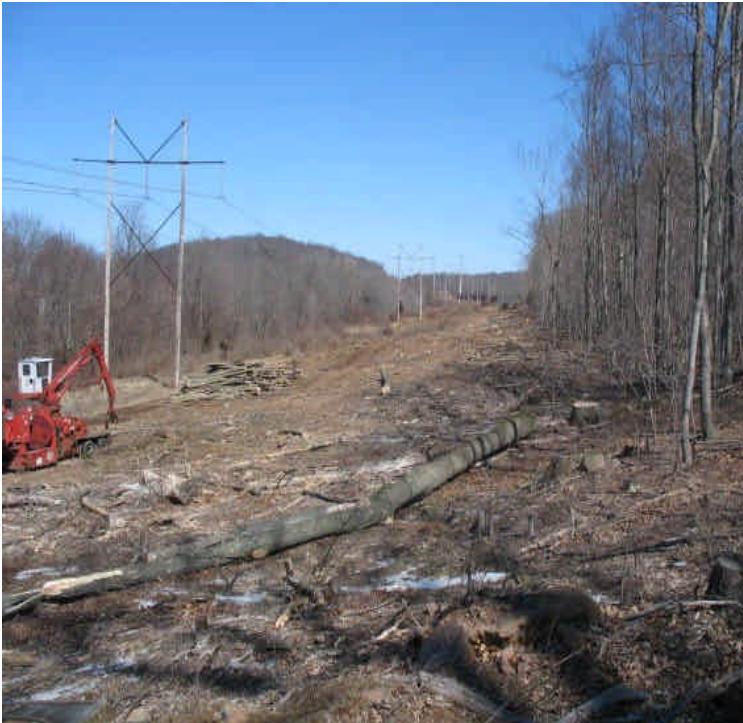
Clearing was occurring north of High Hill Rd. in the ROW moving toward Carpenter Lane and Beseck SS.
