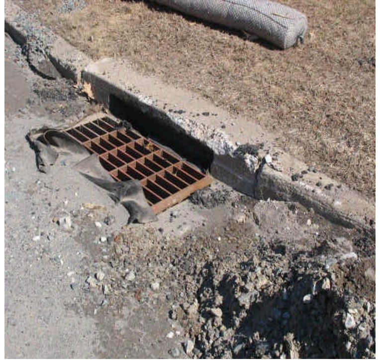
A sediment pile noted near a CB following dewatering activities along Old Farms Rd. The curb cut inlet is exposed and the silt liner is torn here. Replace controls and remove sediment along the roadway.
