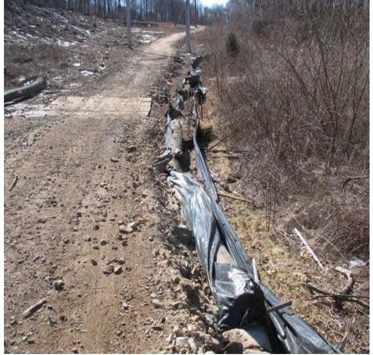
Silt fence and haybales are degraded along the access road off High Hill Rd. Replace/maintain controls when feasible.
