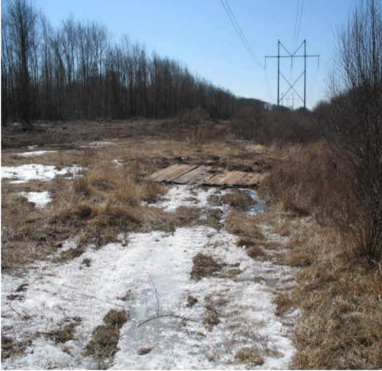
ROW clearing and timber mat installation south of Beseck SS off High Hill Rd. Low vegetation was retained within the wetlands here appropriately. Controls may be needed if soil becomes disturbed.
