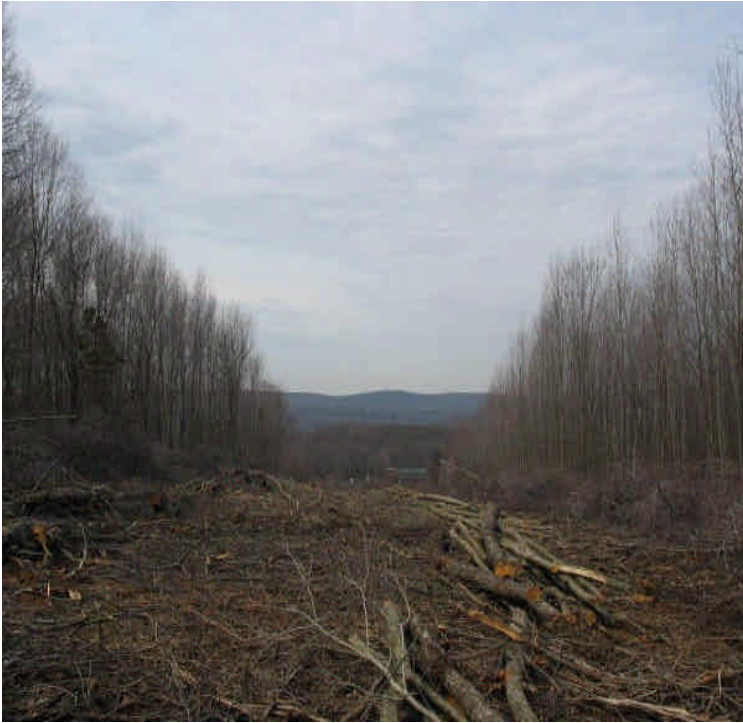
View of the recently cleared portion of ROW looking west toward Route 9.
