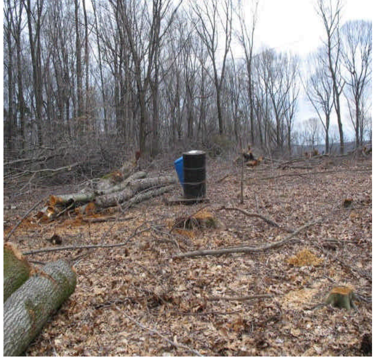
View of two 55-gallon drums stored along the ROW. Drums were located away from wetlands. Trees were being stockpiled, removed, and chipped.
