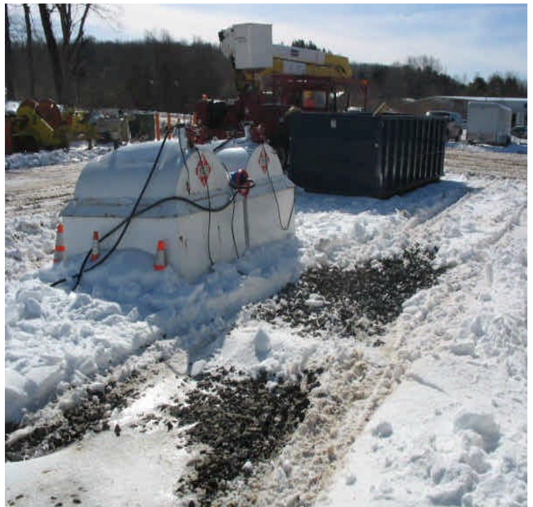
The fuel storage tanks remain in place on the stone spill pad and nozzles are contained. Larger drip stains were noted; spills contained to the stone.
