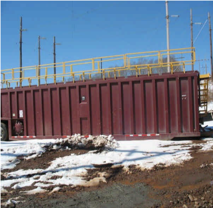
Dewatering tank along the ROW east of Beseck SS. Slurry was removed from the foundation and transported to a containment basin. Controls were in place along the wetland edge.
