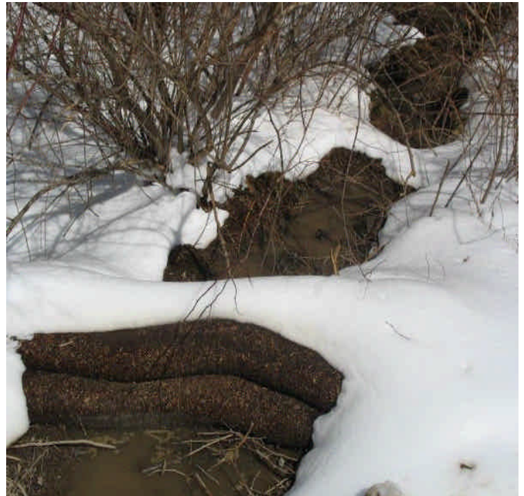
Turbid water and sediment is seeping through some of the controls in some areas located off Powder Hill Rd. Contractors were actively working to repair the problems during the inspection.
