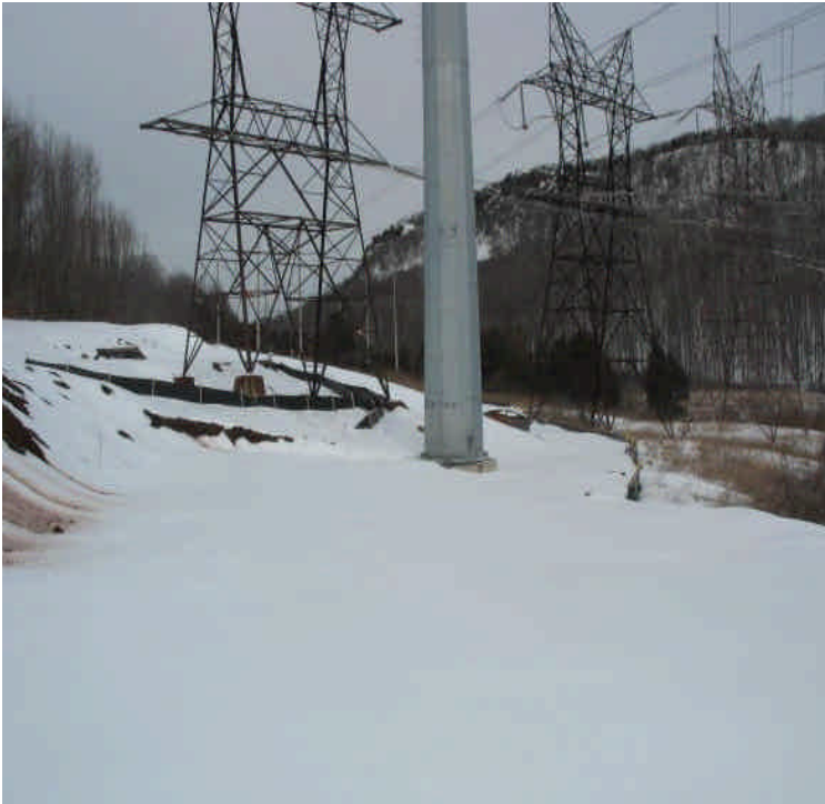
Controls remain stable off Black Pond following installation of the monopole. No active work in this area.
