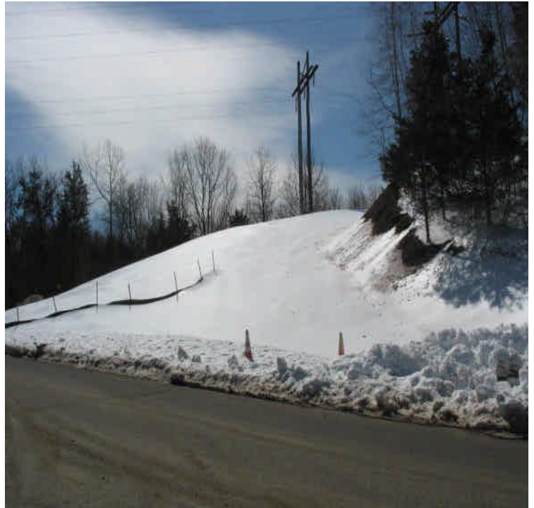
Filter socks were added along the pad and access road slope in the vicinity of the transfer station off Cherry Hill Rd. Ensure that controls are adequate to slow erosion.
