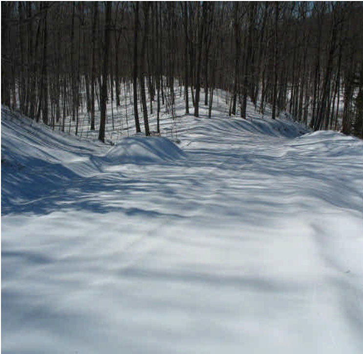
Haybales and water bars are in place along the access road off Black Walnut Dr., currently under snow cover. Continue to monitor the area as snow melts and ground thaws.
