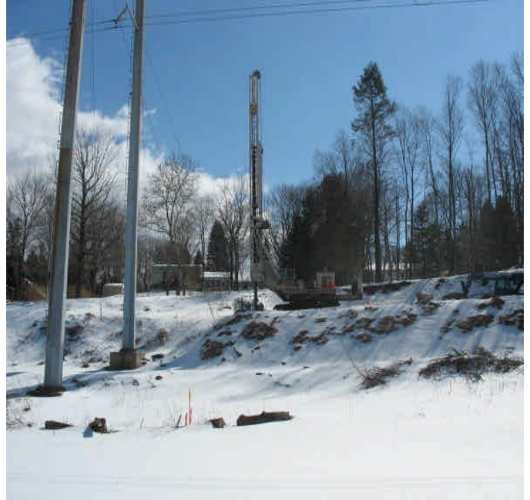
Foundation drilling just south of E. Meriden SS. Slurry pit has been established if needed.
