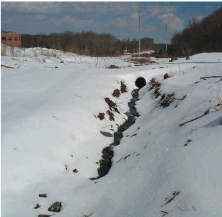
View of the stream flow diverted through the culvert and riprap channel in the ROW between E. Meriden SS to Black Pond. Water in the channel was clear.
