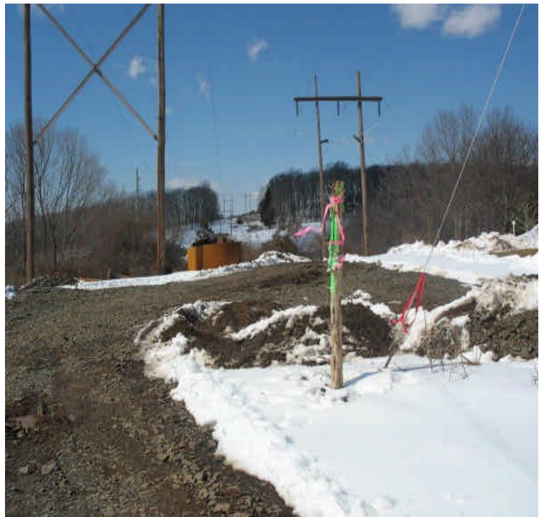
New pad site installed off of Valley View Drive and east of Beseck SS.
