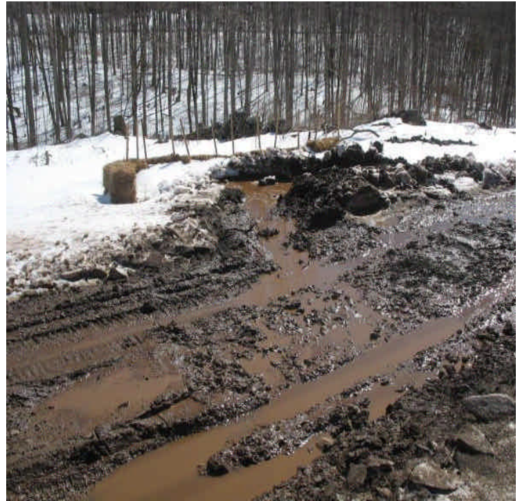
Turbid run-off and mud cover the surface of the access road north of Beseck SS. Consider stabilizing the access road with stone. Remove sediment accumulation from controls as needed.
