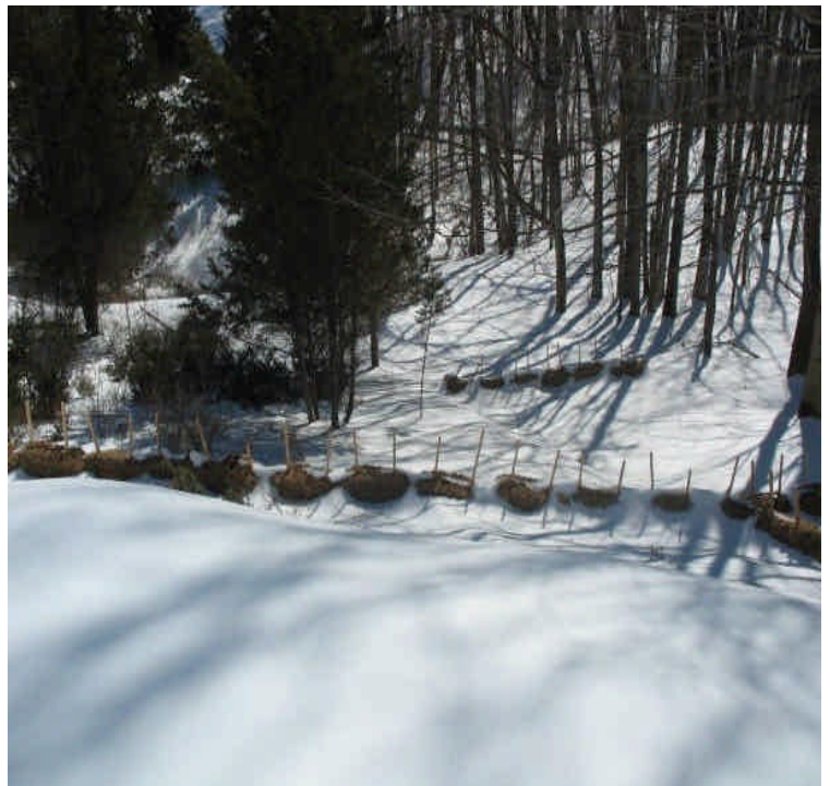
Pad site installed off Black Walnut Dr. upgradient of Ball Brook. Additional mulch, haybales, and a filter sock were placed along the slope in an effort to reduce erosion prior to snow cover.
