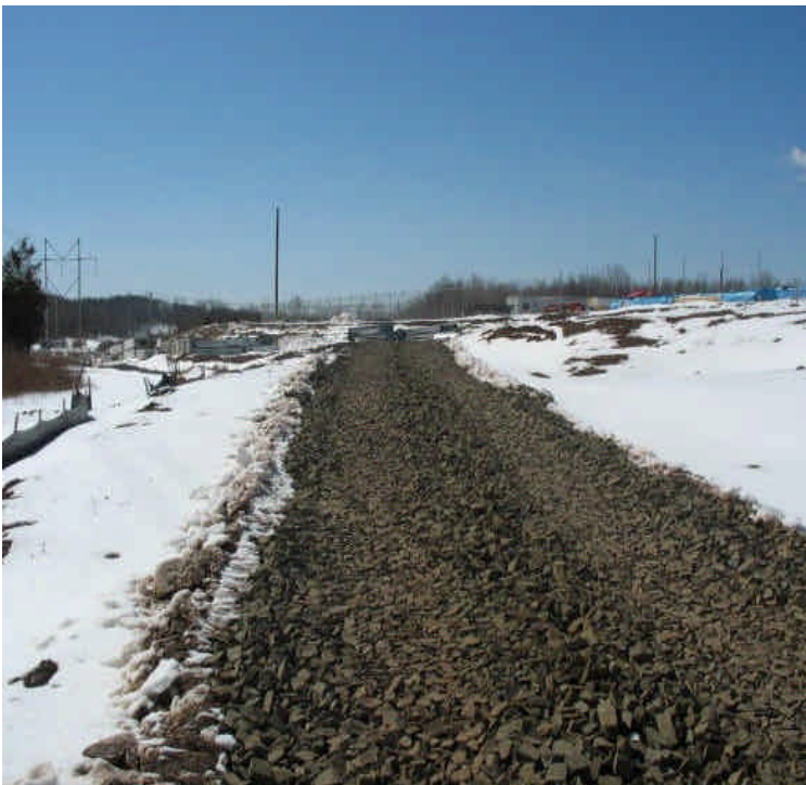
Tracking pad installed along the ROW and connecting to the Beseck SS stone entrance pad to reduce sediment tracking from the ROW.
