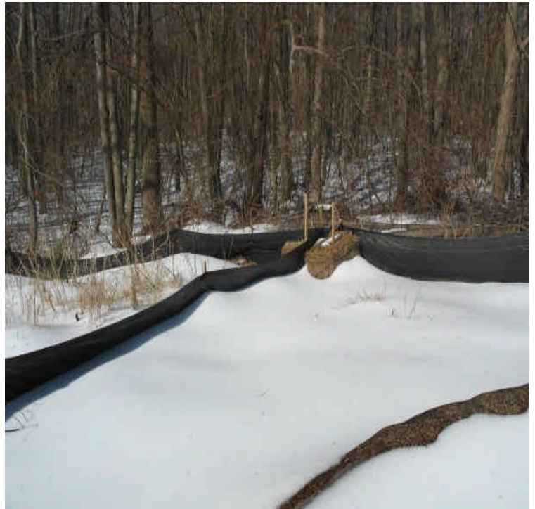
Silt fence, fiber rolls, and hay mulch are in place as a buffer for wetlands around the perimeter of the contractor receiving yard. Fallen sections of silt fence were supported with haybales.
