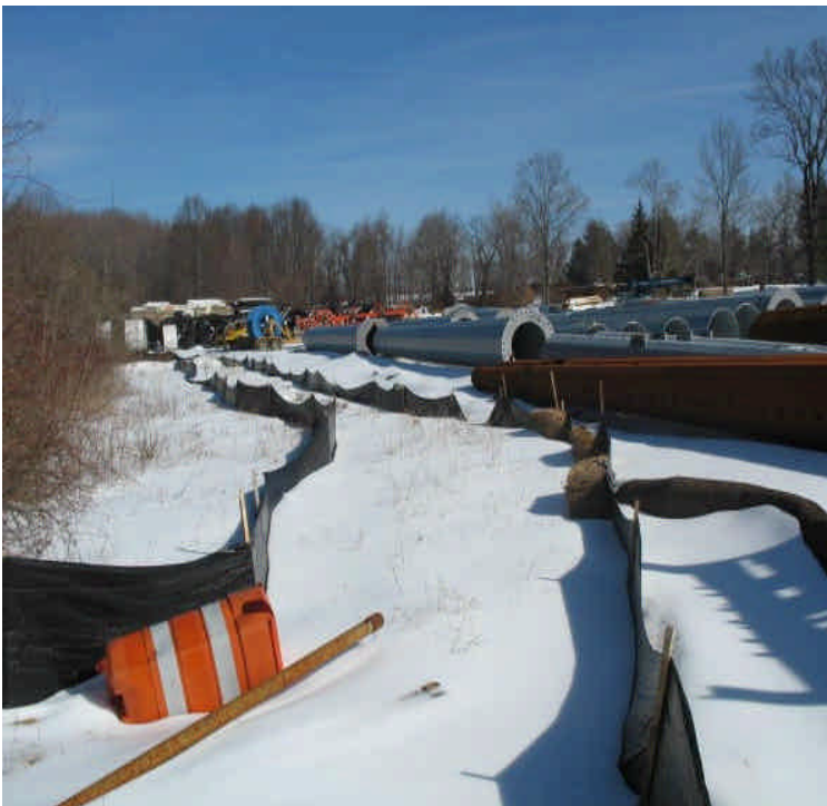
Additional controls remain in place adjacent to wetlands to filter/contain turbid run-off leaving the site.
