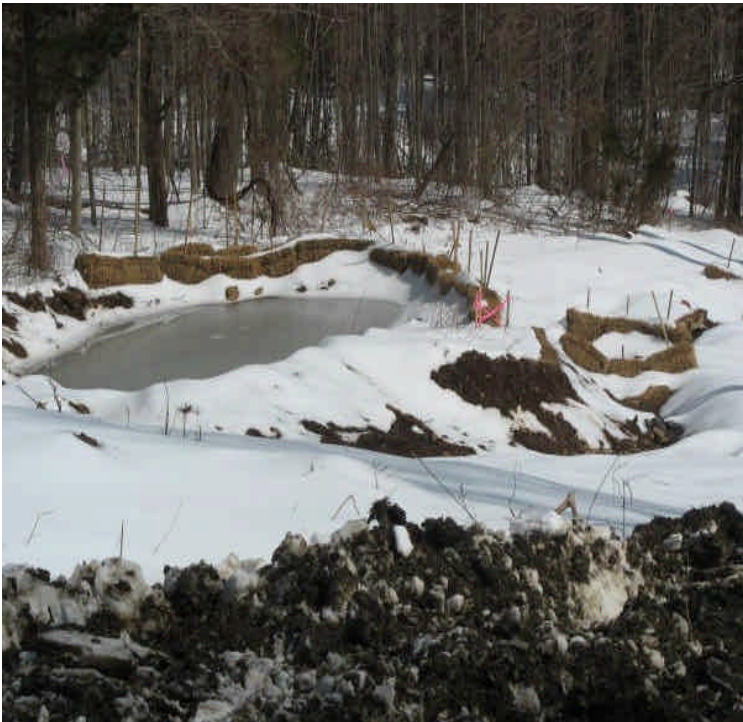
View of water and slurry from dewatering the foundation excavations off Powder Hill Rd. This appears contained to the basin.
