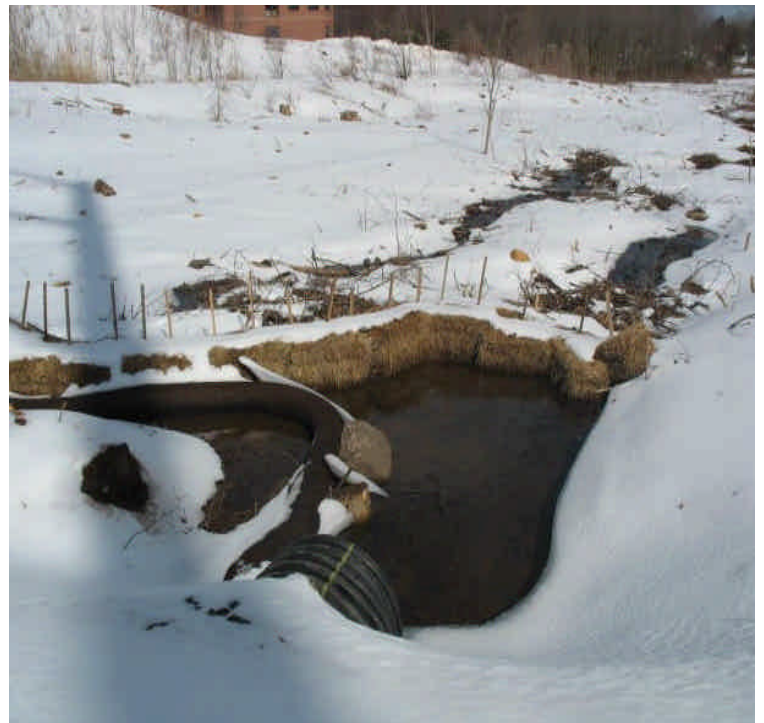
New controls remain downgradient along the diverted stream channel. Controls appear to be filtering all sediment before it leaves the construction area.
