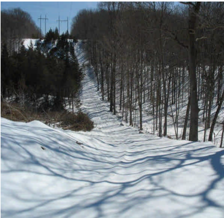
View of access road leading to the culvert area off Black Walnut Dr. Check dams (haybales and stone) were in place along the access road. Drainage ditches/waterbars leading to haybales were installed to direct and filter turbid run-off along the access road.
