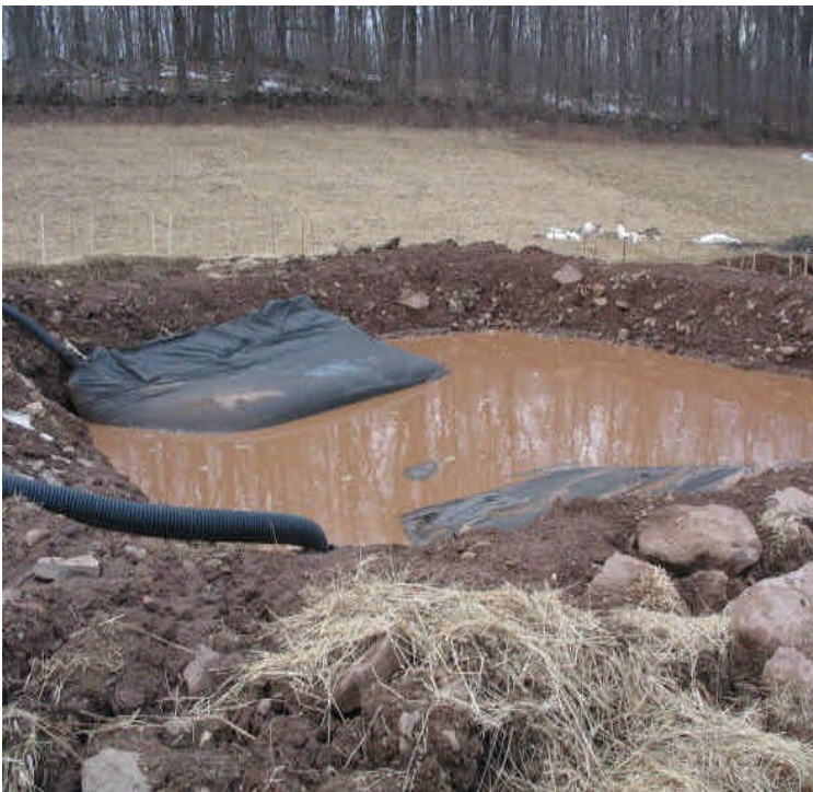
A dewatering basin with filter bags were in place north of Beseck SS.
