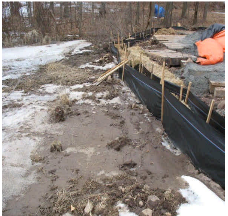
North of Beseck SS: Controls remain in place after the foundation adjacent to the pond was drilled. Ensure that sediment is adequately contained.
