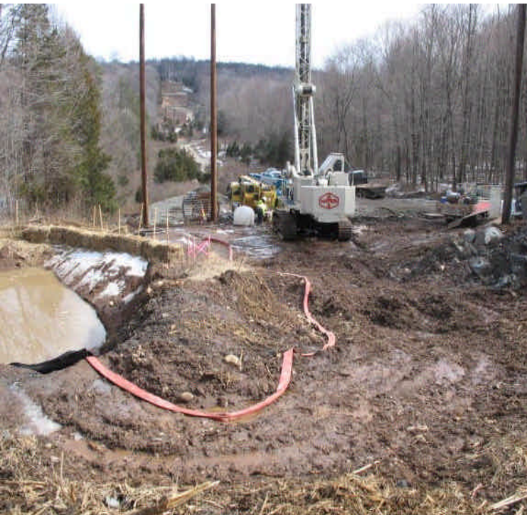
Dewatering and foundation installation off Powder Hill Rd. Water appears to be well contained in a basin at this time.
