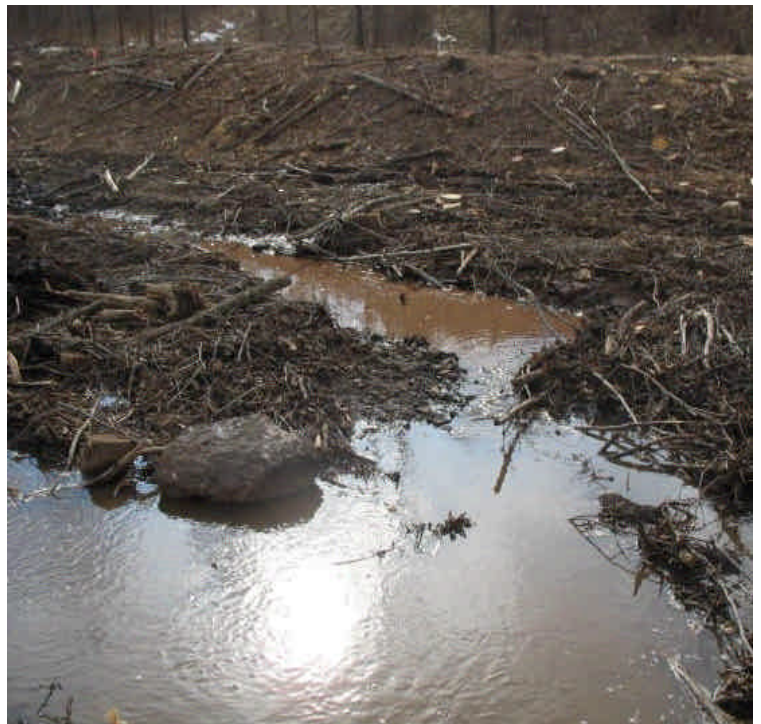
The stream flow was picking up sediment and becoming turbid down-gradient of the diversion. Additional controls are needed (i.e. filter sock across the channel and temporary soil stabilization measures on the adjacent exposed soil and banks).
