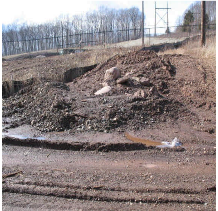
Slurry from foundation drilling in the wetland was being trucked and placed on a slope upgradient. Stabilize soils or install controls as necessary to prevent sedimentation from migrating.
