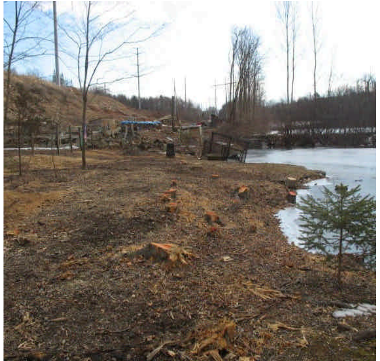
Stumps were left along the bank of a pond to maintain soil stability during clearing along the ROW from E. Meriden SS to Black Pond.
