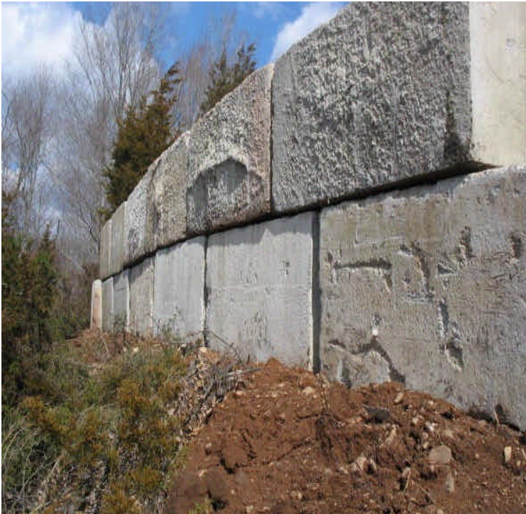
Retaining wall installed along a steep slope at a new pad site in the vicinity of the transfer station land off Cherry Hill Rd.
