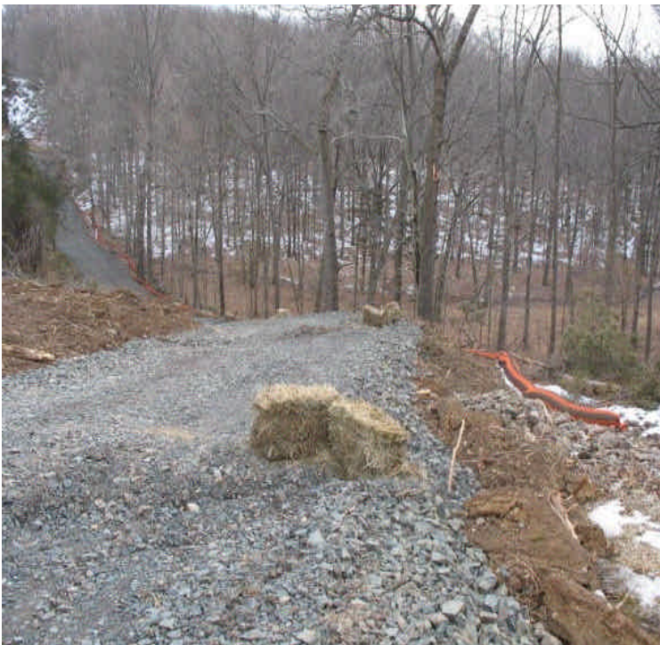
View of access road leading to the culvert area off Black Walnut Dr. Filter socks were in place along the base of slope of the access road. Drainage ditches/waterbars leading to haybales were installed to direct and filter turbid run-off along the access road.
