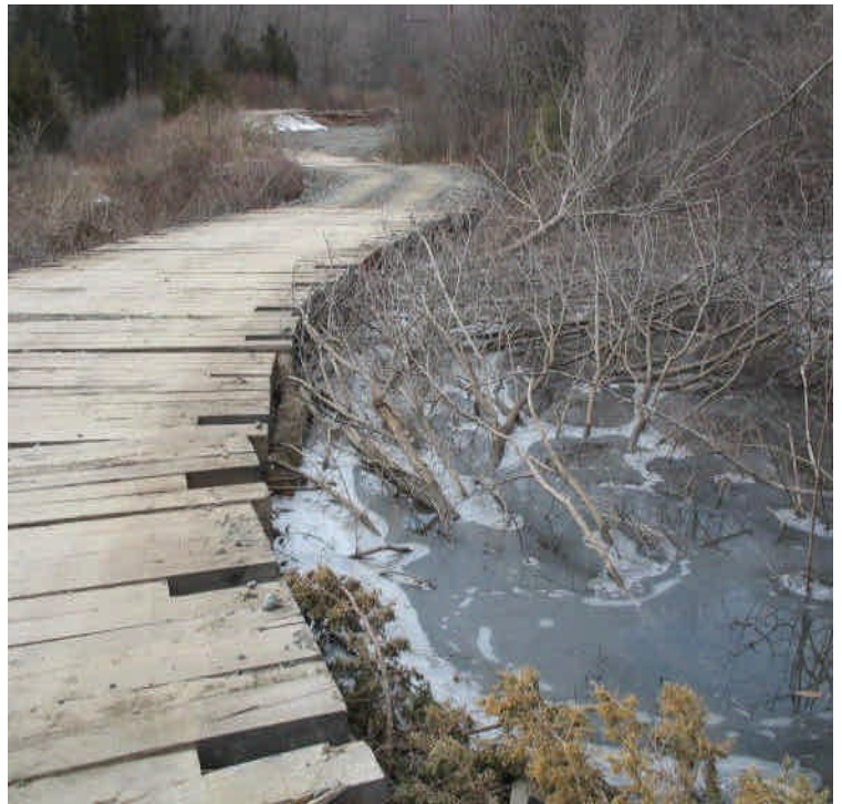
Wetland crossing off Powder Hill Road. No sediment or turbidity was observed coming from the stone crossing
