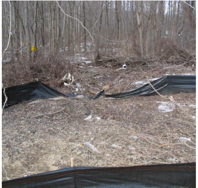
View of some of the erosion controls in place around the perimeter of the contractor receiving yard. Repair the individual sections of silt fence that require maintenance and replace the filter sock that was run over at the entrance.
