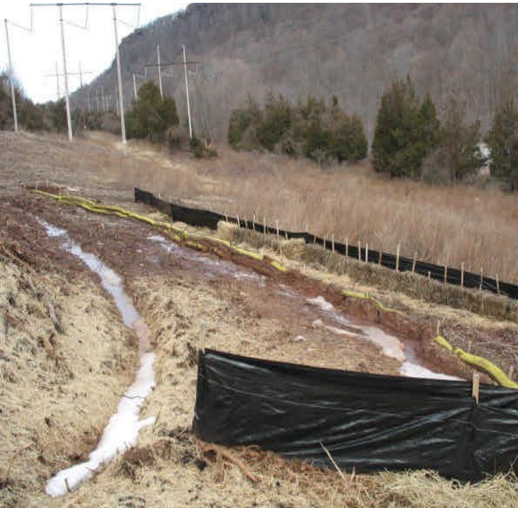
Controls are stable off Black Pond following the installation of the monopole.
