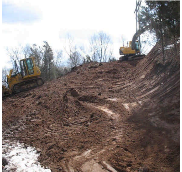
Access road and pad grading in the vicinity of the transfer station land off Cherry Hill Rd. (and vicinity of proposed structures #24523-24)
