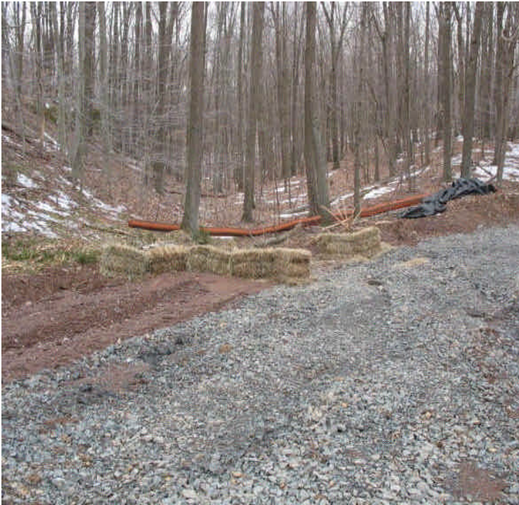
New haybales along the access road off Black Walnut Dr. Access is being installed in this section to reach structure locations to the east. This avoids crossing Ball Brook and associated habitat.
