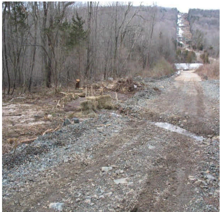
Drainage ditch/water bar and haybales installed along the slope off Powder Hill Rd. Adjust controls as necessary.
