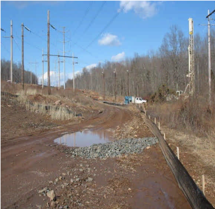
Foundation drilling along the ROW east of Beseck SS. Controls were in place to prevent sediment from entering the wetlands.
