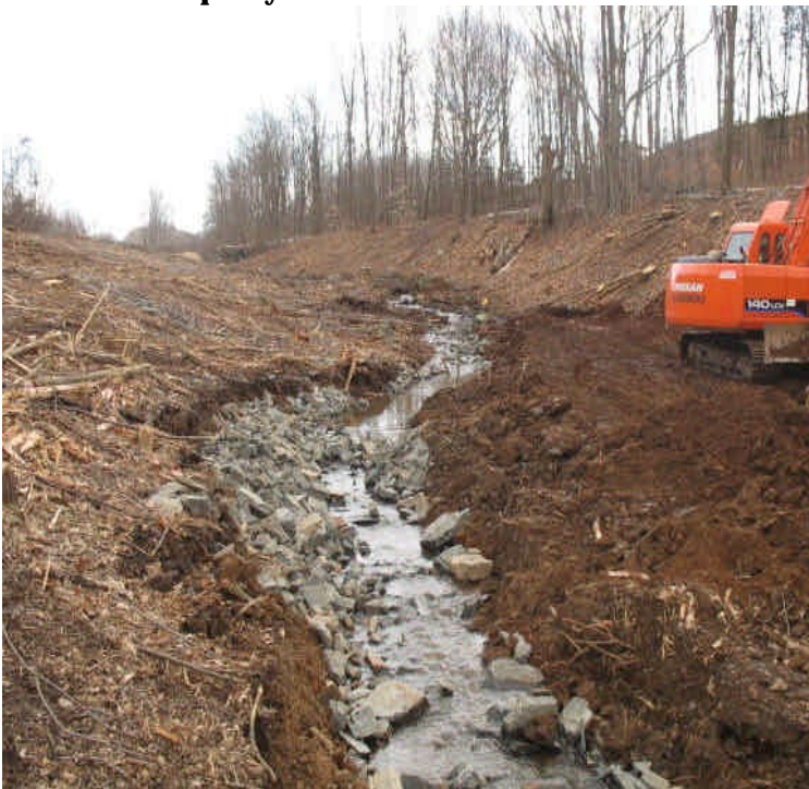
A streambed has been diverted through a riprap channel since pad workspace was necessary adjacent to the existing stream course in several locations between E. Meriden SS to Black Pond. Water in the channel was mainly clear with some suspended sediment.
