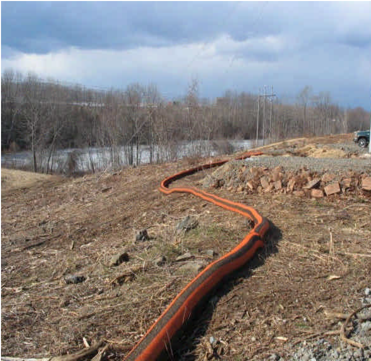
Controls installed along the access road north of Beseck SS to E. Meriden SS. Continue to monitor to confirm filter socks will filter run-off adequately.
