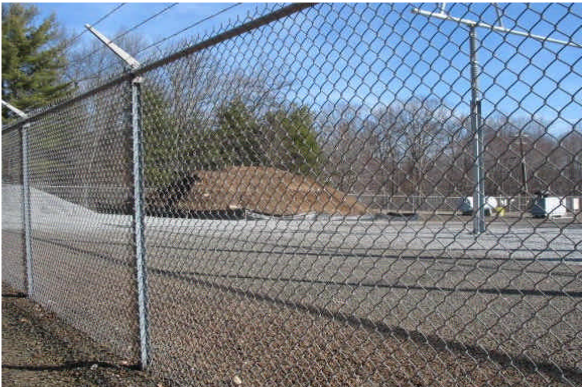
Soil stockpile to be removed. Controls are intact and sediment issues have not been observed.
