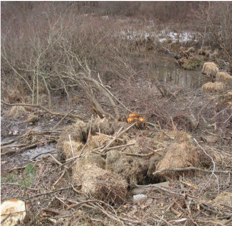
Storm drain outlet across Carpenter Lane has clear water flowing through the haybales. Trees have been cleared in the wetland for Segment 2a work.
