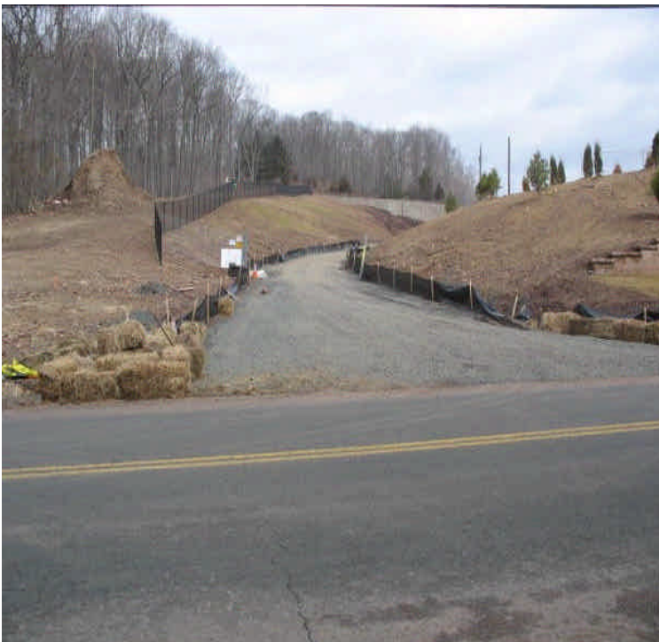
Haybales remain along the edges of the site entrance (west side) in an effort to reduce turbid run-off from the site.
