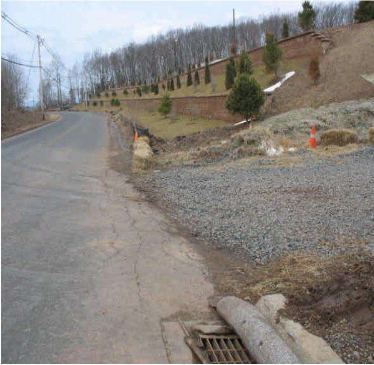
Site exit off Carpenter Lane is at final grade; haybales at the exit have been replaced. Minor amounts of fine sediment tracking are still noted but good efforts are made to keep the area controlled.
