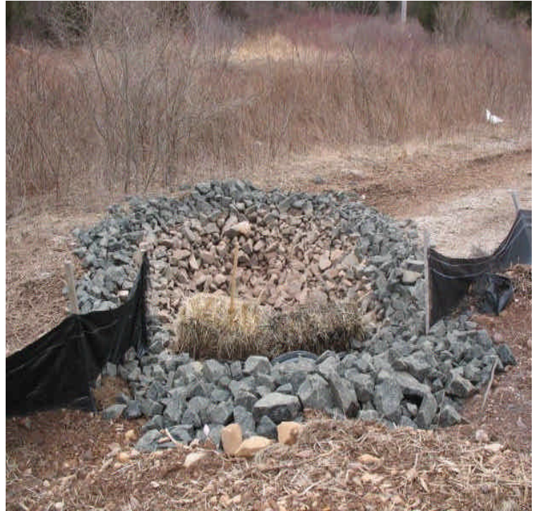
View of the culvert and sediment trap under the access road to the ROW. Sediment appears to be contained.
