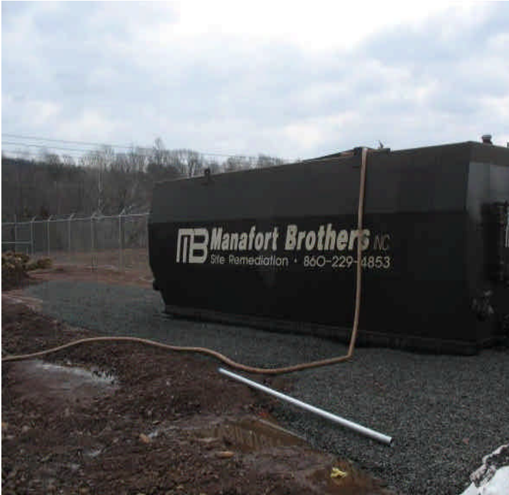
View of settling tank. Foundation pits were filled with rainwater and were being dewatered appropriately to the tank.
