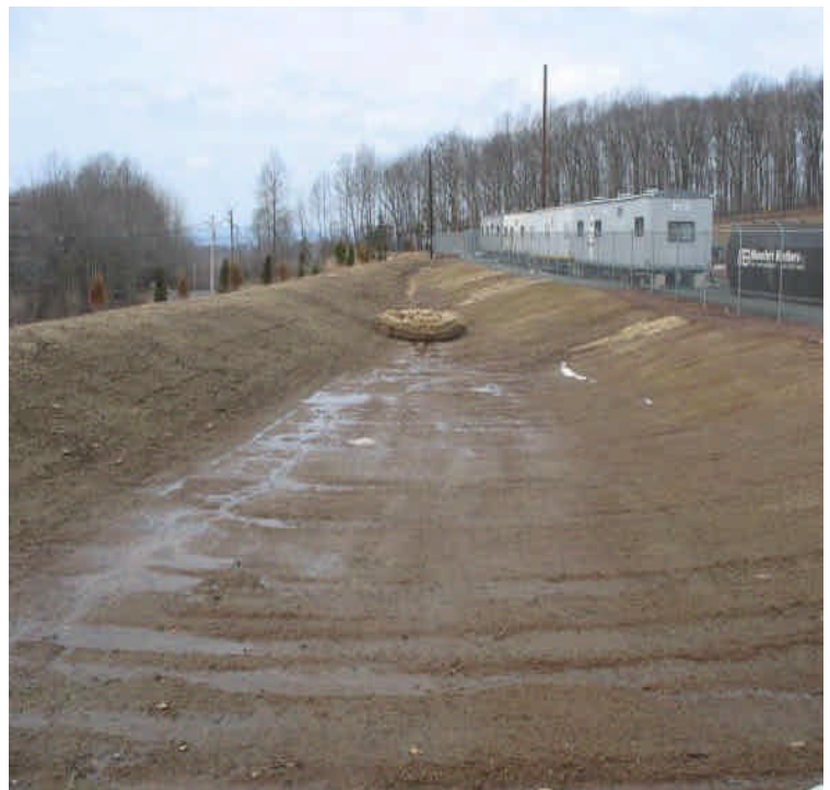
Haybales and controls remain in place at the inlet of the detention basin. Sediment from run-off was contained effectively the last few weeks.
