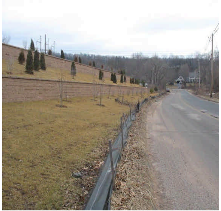
View of Carpenter Lane and retaining walls. Some slight sedimentation (as well as sand from town sanders) was noted along the gutters. Catch basins controls could use maintenance.
