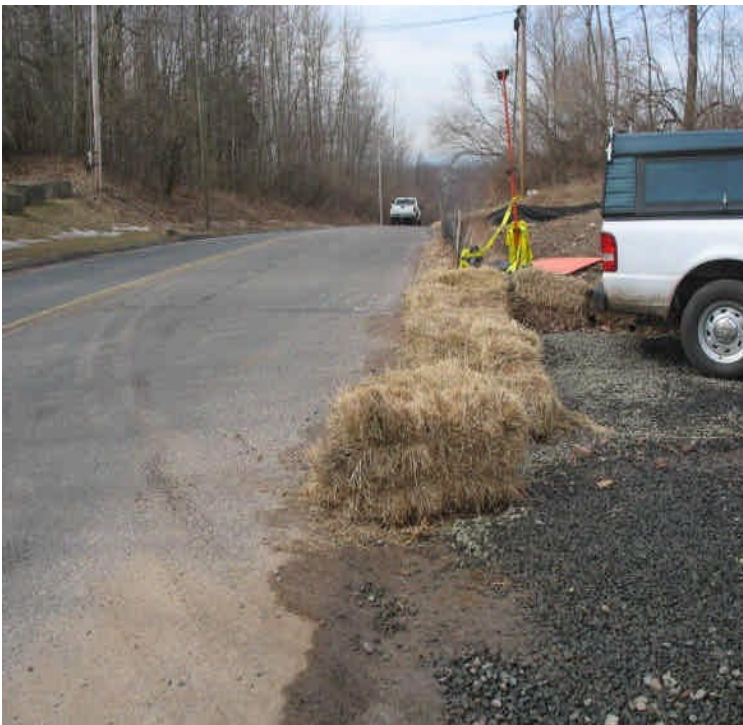
Haybales were placed across the site entrance (west side) in an effort to reduce turbid run-off from the site. Some sediment accumulation was noted at the edge of the entrance.
