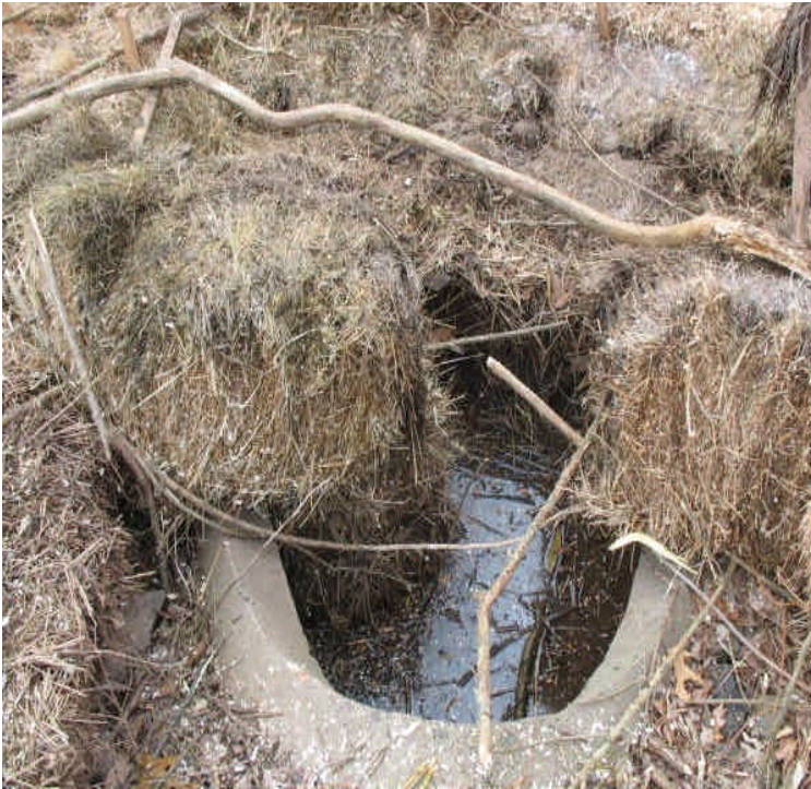
Storm drain outlet across Carpenter Lane has clear water flowing through the haybales. The ice cover in the culvert and wetlands has melted. Efforts on site appear to have retained sediment.
