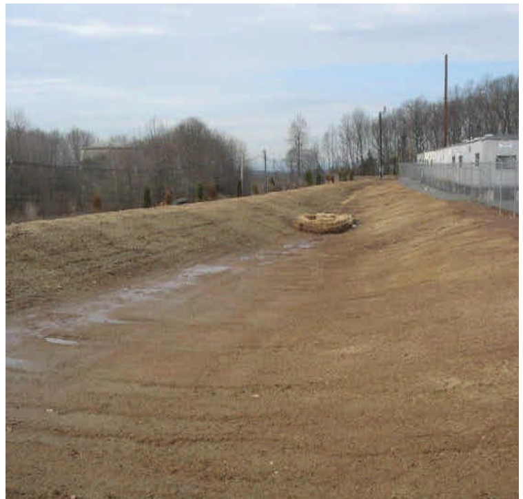
Haybales and controls remain in place at the inlet of the detention basin. Sediment from run-off appears to be contained effectively.
