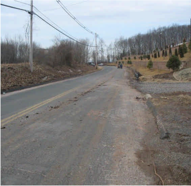
Site entrance/exit off Carpenter Lane is at final grade; haybales at the exit are degraded and should be replaced. This was going to occur shortly. No run-off was noted at the time. Tracking on the roadway was a result of Segment 2A, ROW clearing crews.
