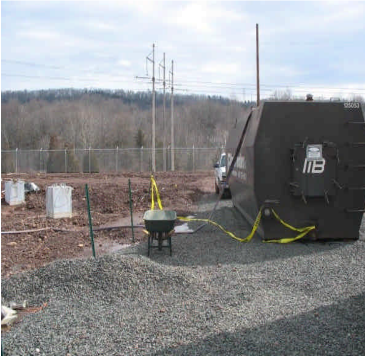
View of dewatering into a settling tank. All water from site is well contained at this time.
