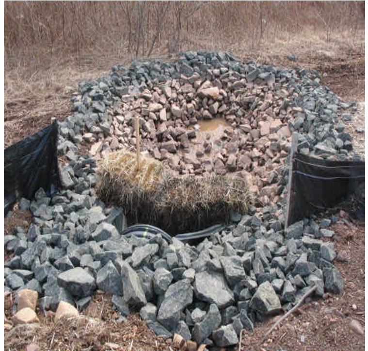
View of the culvert under the new access road. Turbid water has mostly filtered out of the trap and sediment appears contained.
