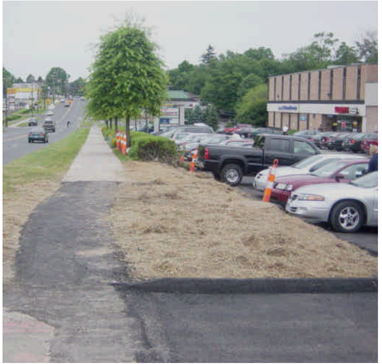
Exposed soils at vault #7 have been stabilized with hay mulch. The sidewalk was repaved and the curbing was restored.
