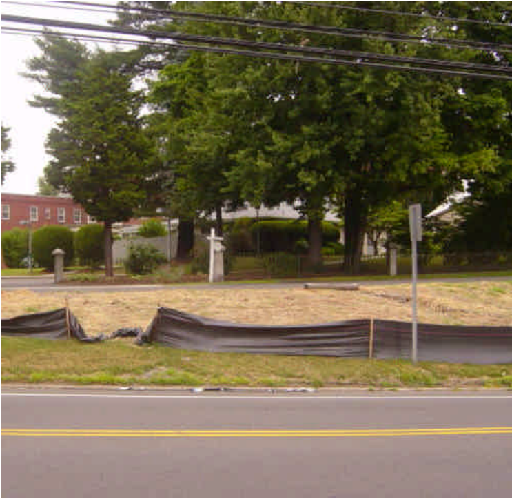
A gully had previously formed near vault #5. A silt sock has been placed at the top of the slope to minimize further erosion. The silt fence was also repaired, but a new section now needs attention. Stabilize as soon as feasible.
