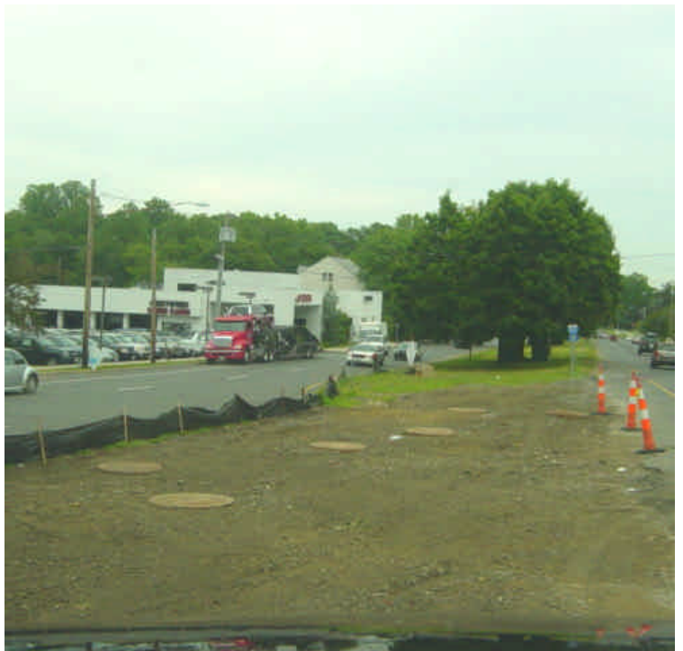
Hard-pack soil is in place near vault #19 to temporarily stabilize the exposed area. Silt fence remains along the down gradient side of slope.
