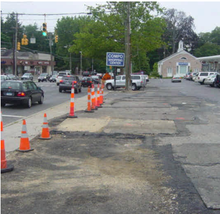
Steel plates are temporarily in place near vault #17. This area is scheduled to be paved later this week.
