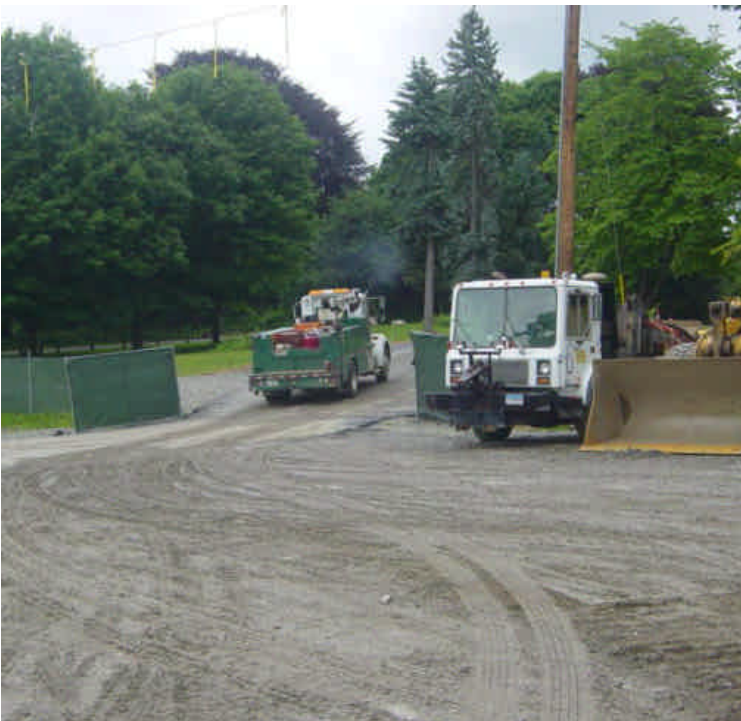
Some tracking was noted from the Sherwood Island lay-down yard. However, the entire access way has been paved, aiding in reducing tracking to the main roadway.
