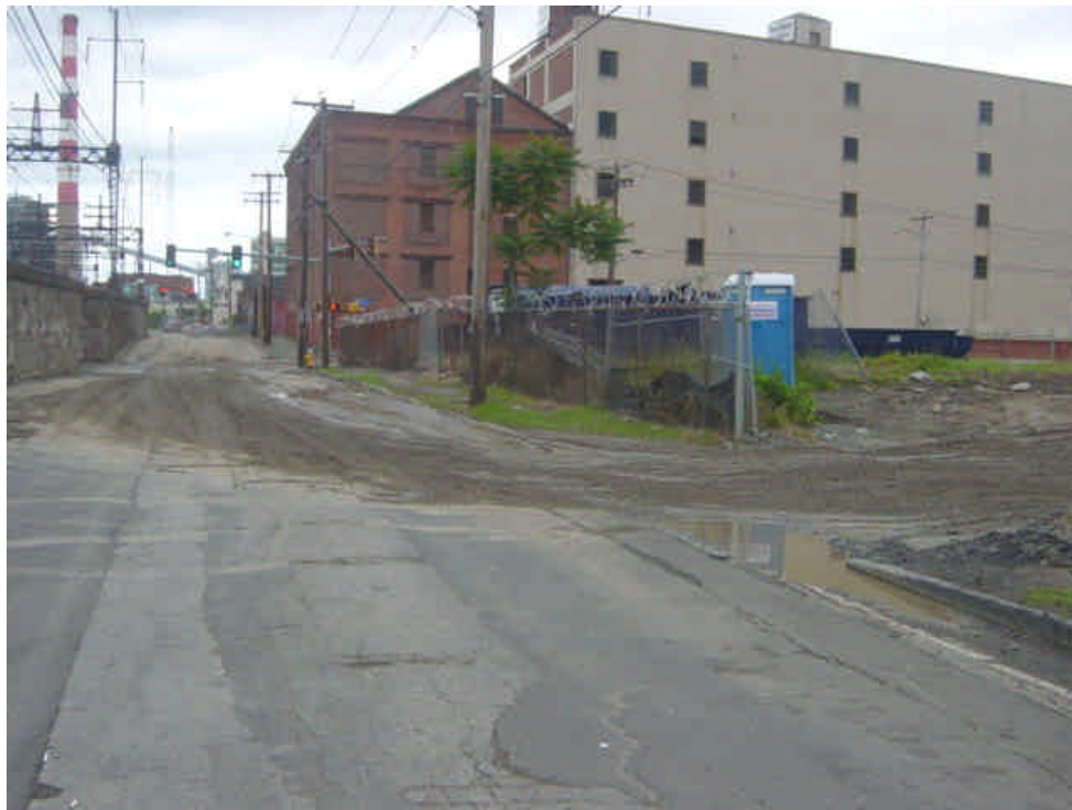
Heavy tracking was noted this week at Railroad Ave. near its intersection with Myrtle Ave. The tracks were originating from a stockpile yard that is not associated with this project. Catch basins in this area remain overwhelmed with sediment.
