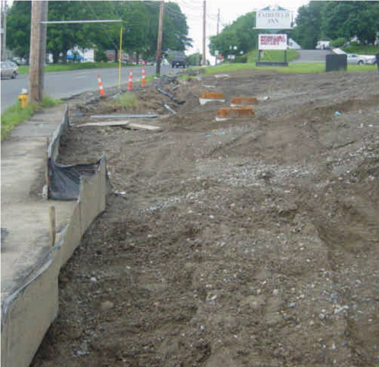
Photograph of controls near sta. #612 that appear to have been driven over earlier that morning by a motorist (not project-related).
