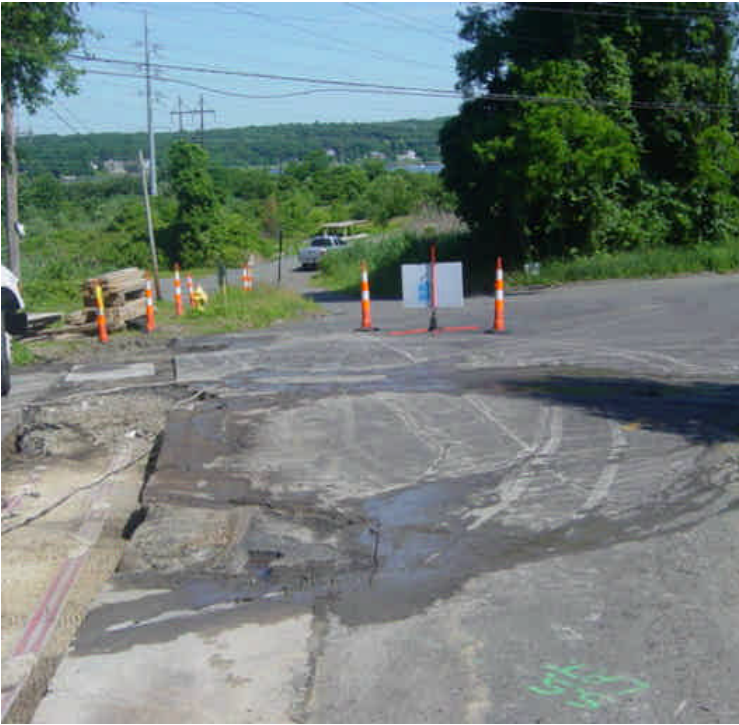
Trenching and saw cutting work near sta. #1049 to #1050 was ongoing at the time of the inspection. A minor amount of slurry was migrating along the roadway which has the potential to enter catch basins. Continue to provide good efforts to sweep roadways.
