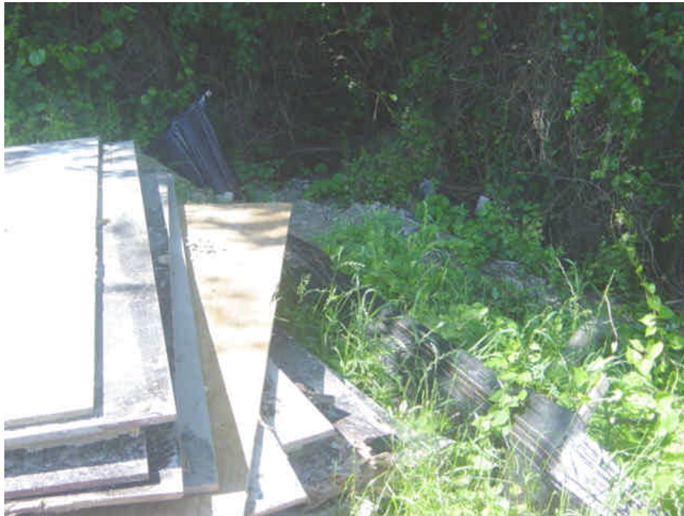
Steel plates were stockpiled close to a section of silt fence near sta. #1050. The damaged section of silt fence should be restored and the plates should be pulled back.
