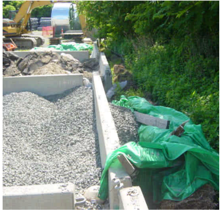
Materials being stored in the Milford lay-down yard remain over the jersey barrier containment area. The materials are stable and remain at the boundary of the silt fence and will be addressed as part of final restoration once the yard is closed/demobilized.
