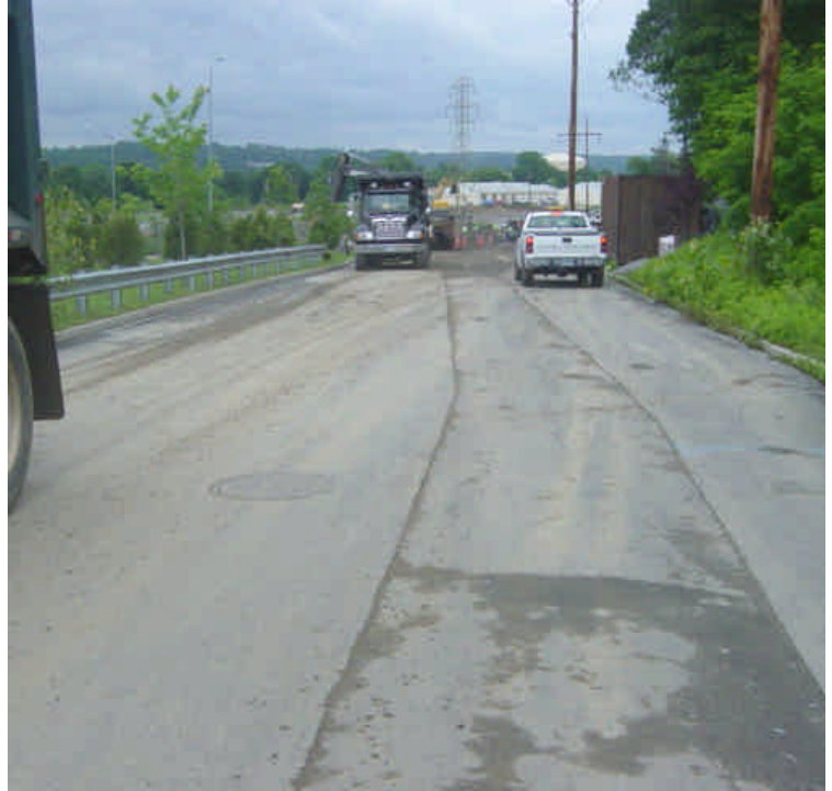
Tracking was noted onto the paved portion of Shelland St. This appears to be largely contributed to trucks entering and exiting the East Devon substation construction site. Coordinate with other contractors to keep this roadway clean if appropriate.
