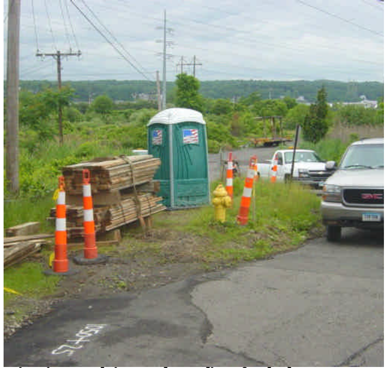
A sani-can was being stored upgradient of wetlands near sta. #1050. These facilities should be stored greater than 100-feet from wetland areas whenever feasible.
