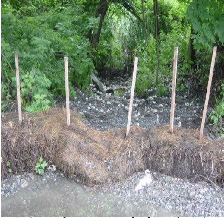
Erosion controls near sta. #1015 and vault #1 are functioning. Continue to control sediment and run-off associated with stormwater.
