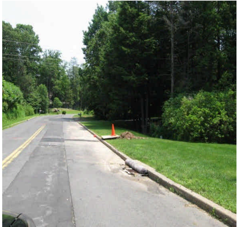
Some minor dust/sediment remains in the roadway after patch work was completed along Old Farms Rd. Sweep as needed.
