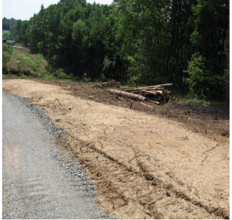
New access road being installed of Tuttle Ave. Ruts noted last week were graded, and hay mulch and seed were applied for stabilization.
