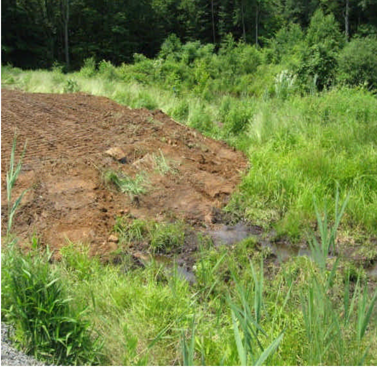
New pad in the wetland, within the apple orchard. Add controls as to protect the undisturbed portion of the wetlands. Avoid storing equipment on the pad within the wetlands
