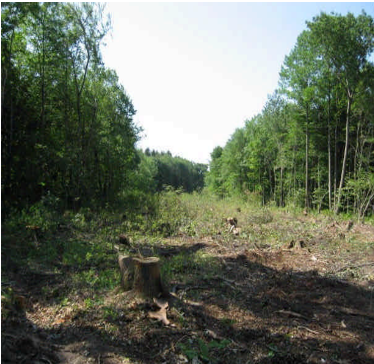
Clearing via helicopter completed within a sensitive area in the Watershed protection area. Stumps and low growing vegetation remain in place to stabilize soils.
