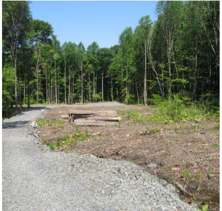
Site entrance within the receiving yard. Timber mats were stockpiled adjacent to a wetland area and should be relocated
