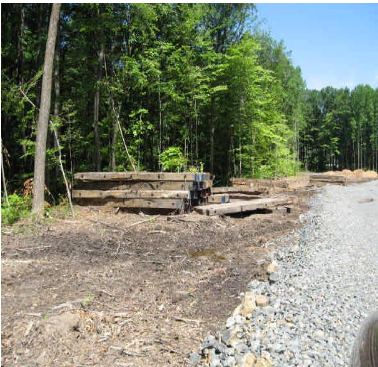
Stack timber mats or relocate to reduce impacts to vegetation regrowth. (e.g. place in a new upland pad site to be impacted by equipment).
