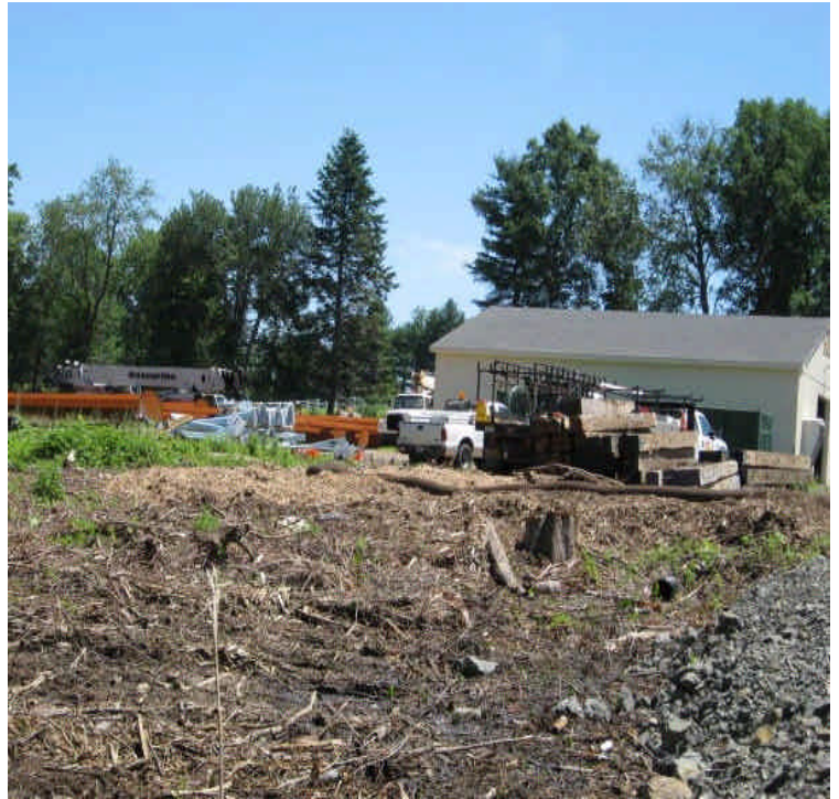
Site entrance within the receiving yard. Mulch was applied along the disturbed soils here.
