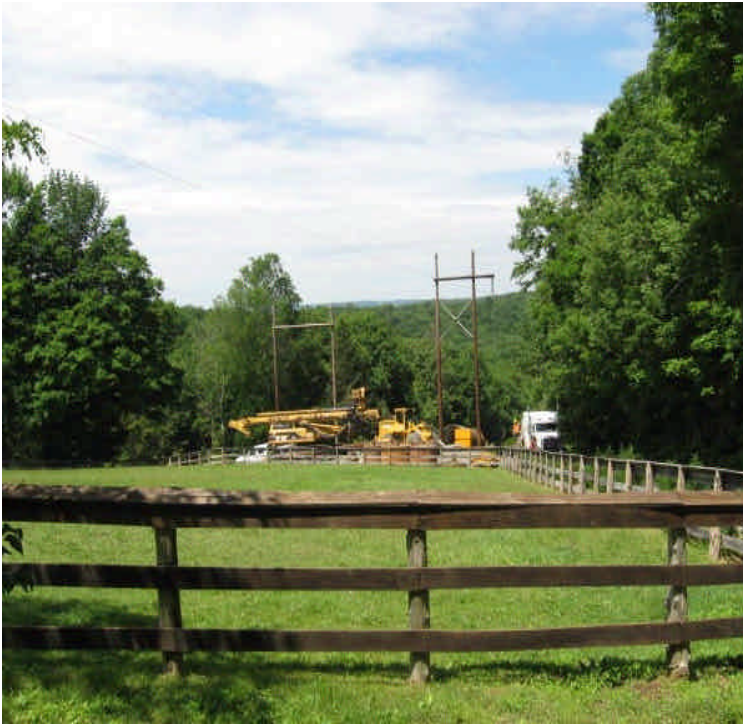
View looking toward Foot Hills Rd and Johnson Ln. Crews were preparing to start drilling off Foot Hills Rd.
