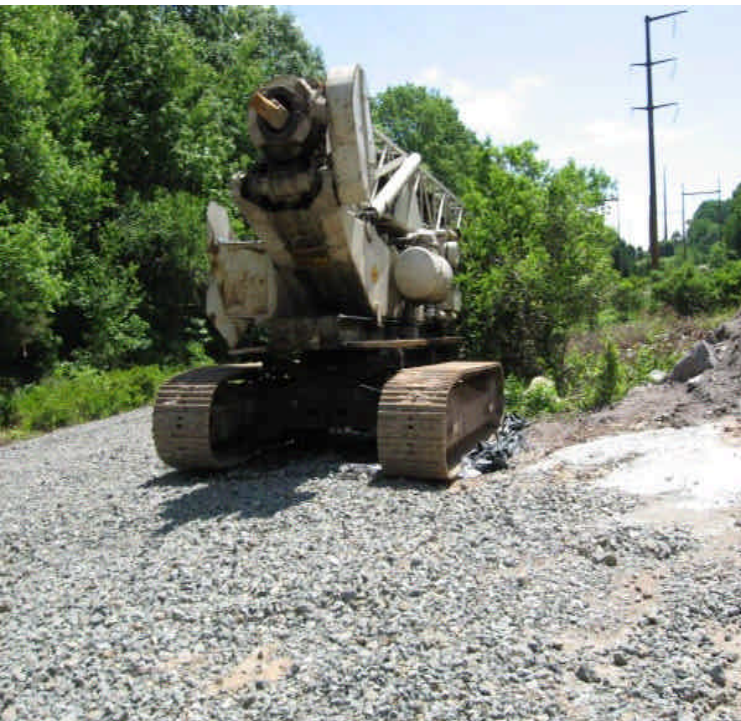
Broken equipment was relocated closer to the adjacent wetlands. It should be repaired as soon as possible. Ensure controls fully contain the leak.
