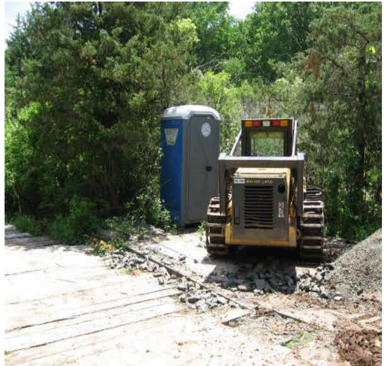
Portable sanitary facility located immediately adjacent to the wetlands off Durham Road. It should be relocated to an appropriate location in case of a spill.
