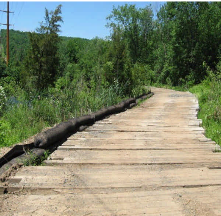
View of well installed haybales and fiber rolls at the timber mat crossing off Powder Hill Rd. Sediment is filtered from the run-off before it flows off-site in this area. Some turbid water is retained here.
