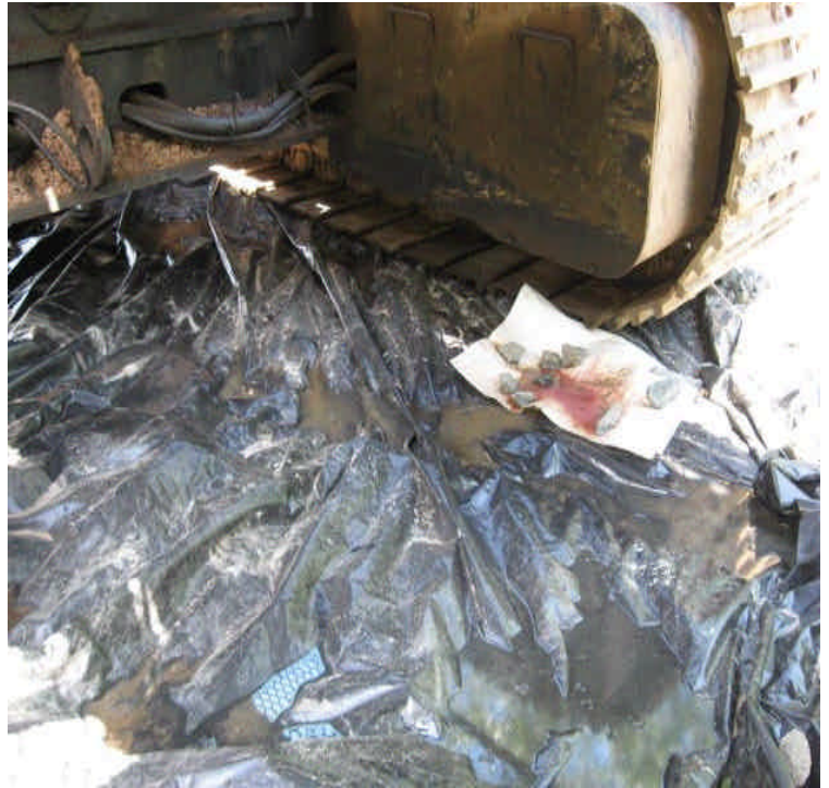
Fluid was still leaking from a drill rig off Haddam Quarter Road but increased controls have been placed here to contain the drips.
