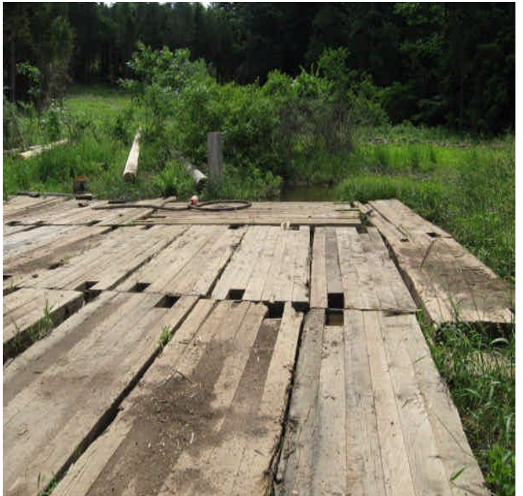
Timber mat crossing located east of Beseck SS. Controls need to be reinforced/extended.
