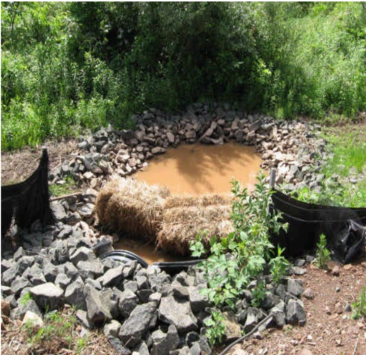
Sediment trap east of Beseck SS. Turbid water was contained within the basin but capacity is not adequate for larger storm events.
