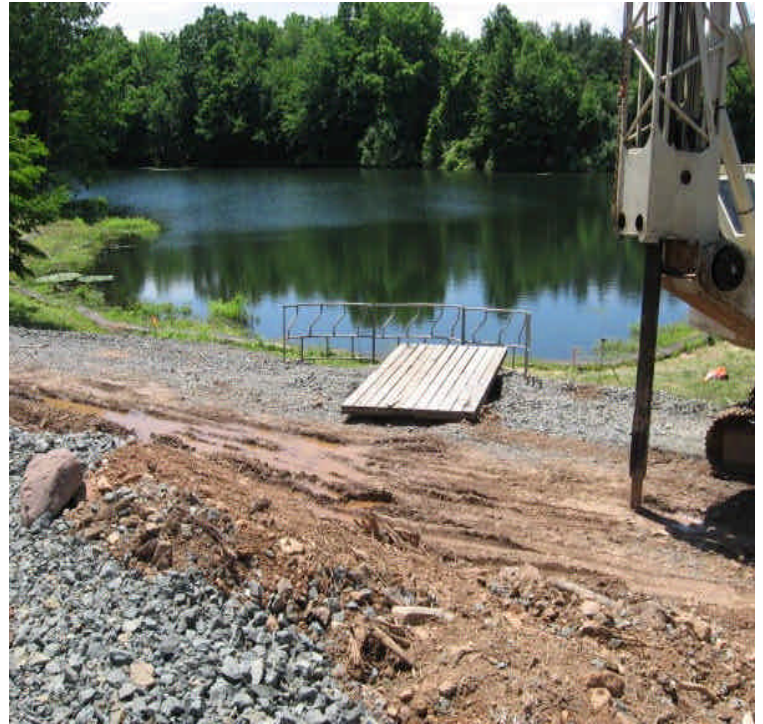
Foundation drilled north of E. Meriden SS. Controls are in place at the edge of the pond but more may be needed to control run-off.
