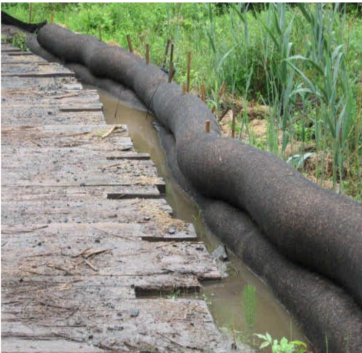
View of well installed haybales and fiber rolls at the timber mat crossing off Powder Hill Rd. Sediment is filtered from the run-off before it flows off-site in this area. Some turbid water is retained here.
