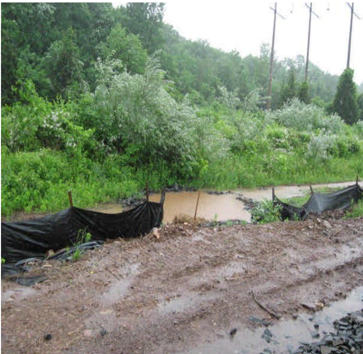
Turbid water was overflowing the sediment trap east of Beseck SS and flowing directly into the wetlands here during a heavy rain event. Work with Beseck contractors to provide adequate capacity during larger storms.
