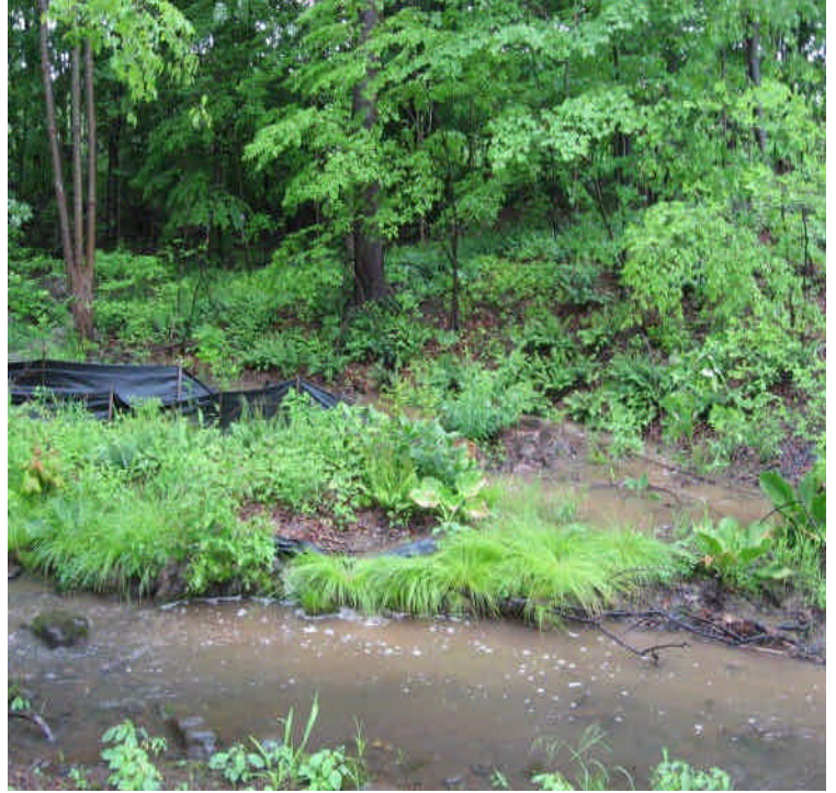
Turbid water entering stream from off site ball fields, south of High Hill Road. Repair/extend project controls as feasible.
