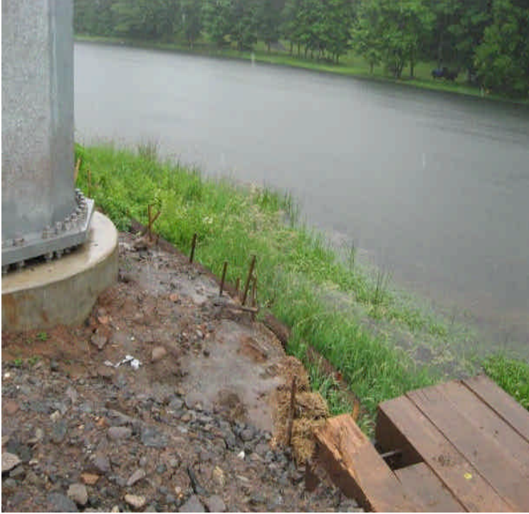
View along the pond north of Beseck SS to E Meriden SS off Fleming Rd where pole installation is complete where sediment has filled controls to capacity immediately adjacent to the pond. A filter sock has been added as another layer of control but sediment should still be removed.
