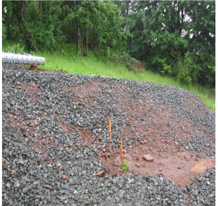
View of the pads installed north of East Main Street. Structures were delivered for installation.
