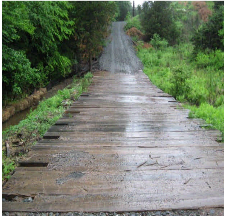
Timber mat crossing off Johnson Ln. Monitor turbidity carefully here as the adjacent area provides amphibian breeding habitat.
