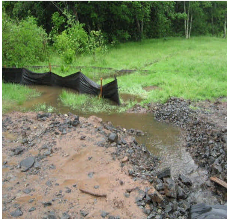
Run-off at the Little Lane wetland crossing. Silt fence check dams were filtering most before it left site.
