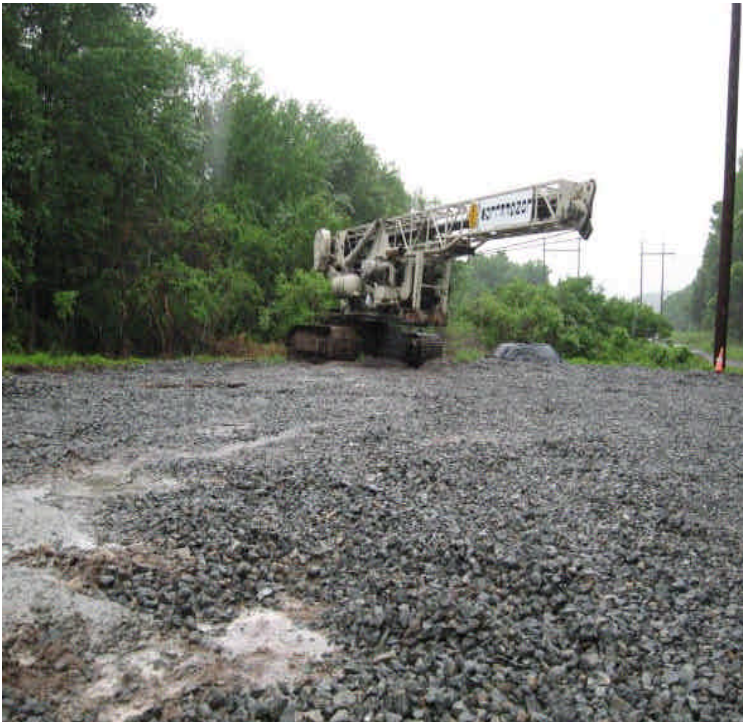
Broken equipment was relocated closer to the adjacent wetlands. It should be removed as soon as possible; more controls are needed.
