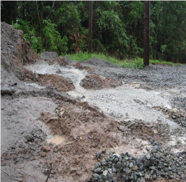
Concrete containment area overflowing onto a pad site upgradient of a wetland off Haddam Quarter Road. Provide adequate capacity and remove concrete material.
