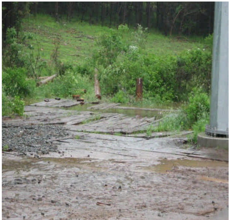
Timber mat crossing remaining east of Beseck SS had turbid run-off. Controls need to be reinforced/extended.
