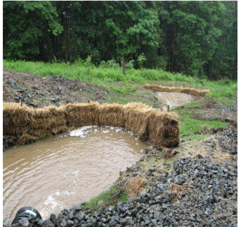
Controls/check dams along the slope of Beseck Mt. Good efforts to control run-off were noted but stormwater volumes were high during the heavy rain.
