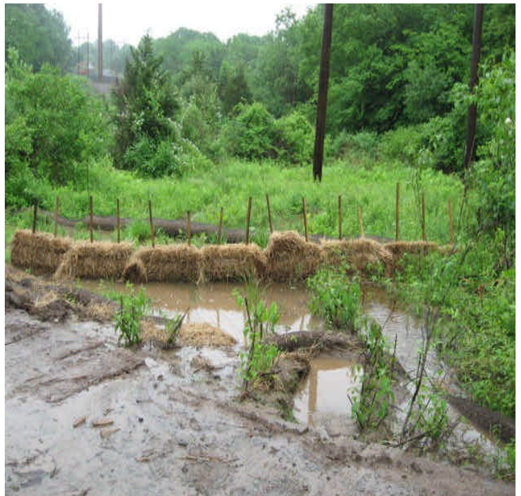
Fiber rolls and haybales west of Powder Hill Rd are filtering turbid water before it enters the pond. Remove any accumulated sediment from wetlands when water recedes and when sediment is deeper than 2".
