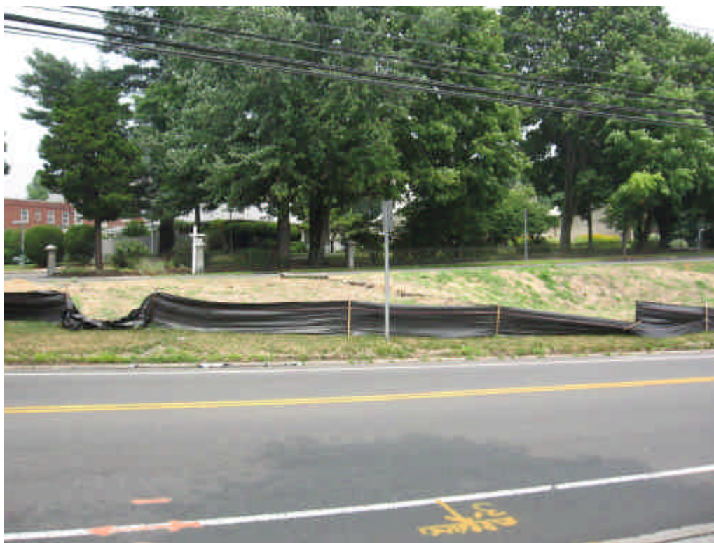
Photo of erosion controls at vault #5, a section of silt fence remains in need of repair. No evidence of additional erosion at the site and some vegetative cover was starting to establish.
