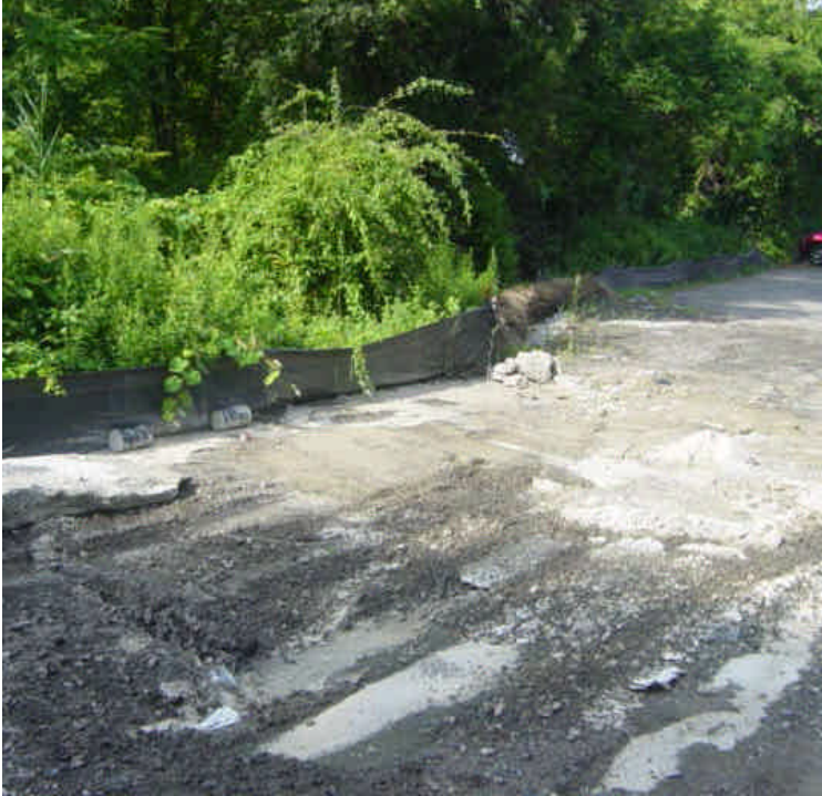
Concrete slurry appears to have been deposited near the backfilled area of vault 1, (potentially by other contractors on a separate project). Concrete washouts should be performed in a contained area. Multiple sections of silt fence are in need of repair between sta. #1015 to #1020.
