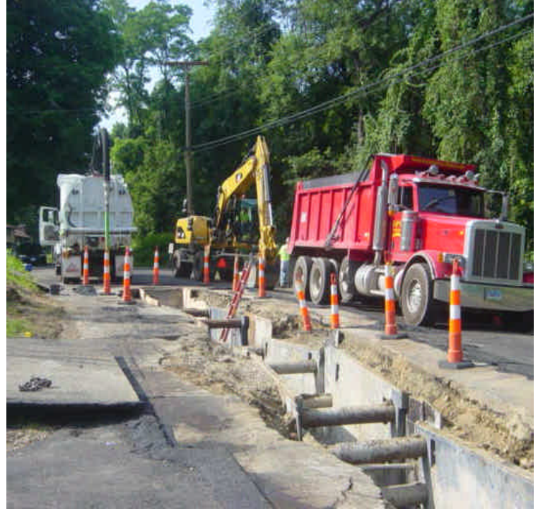
Trench excavation activities continue at sta. #1048. The exposed soil along the slope on the left side of the photo should be contained/stabilized to prevent erosion.
