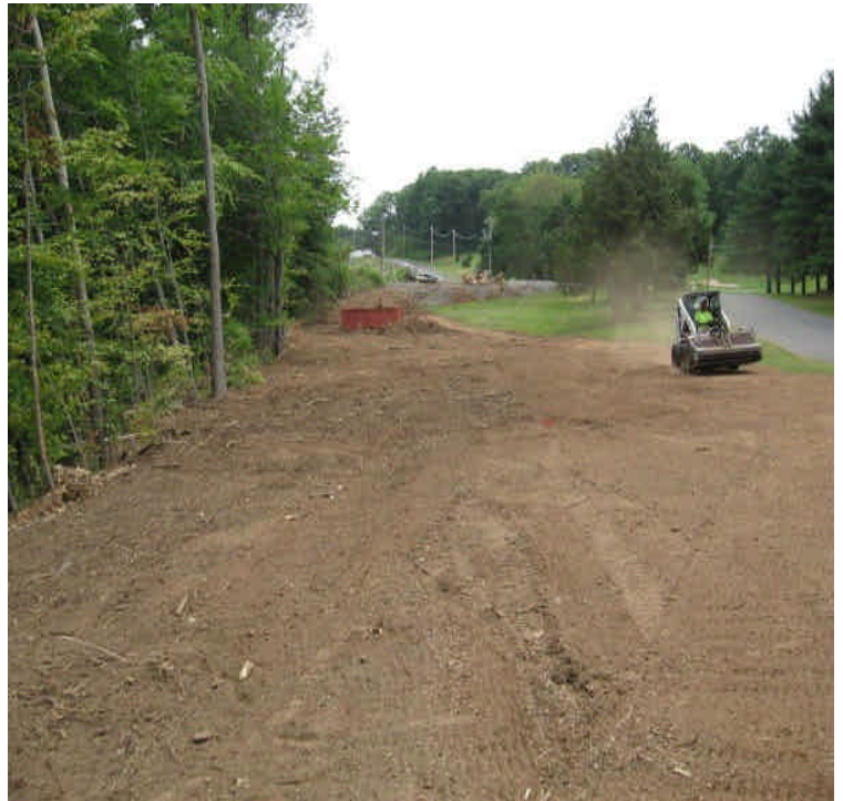
Grading noted off Harrison Rd. as the area is being prepared for hydroseeding.
