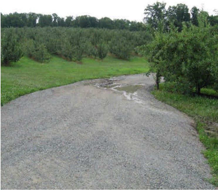
A drainage channel was dug within the apple orchard off Mansion Rd. A culvert appears to be necessary to reduce sedimentation
