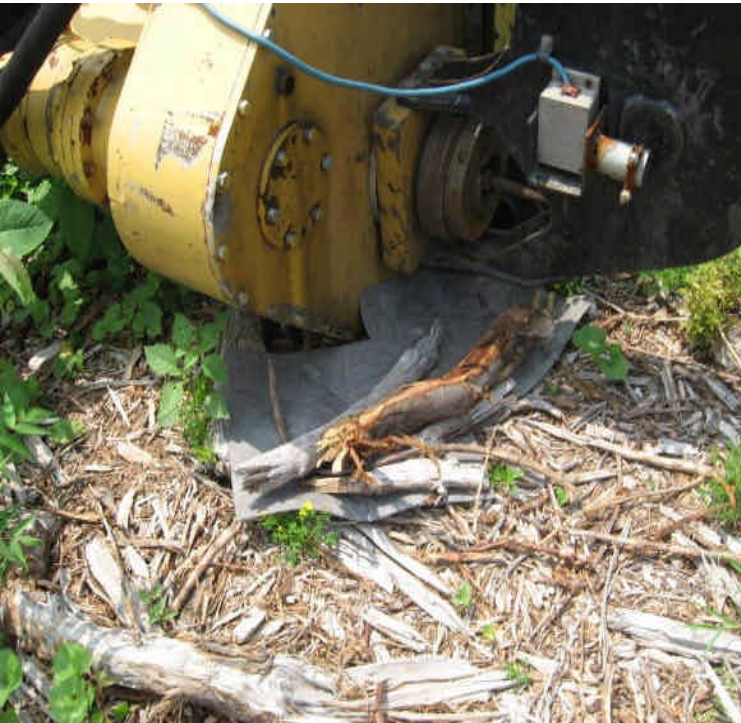
Hydraulic fluid dripping from equipment parked off Carpenter Ln. Some controls were placed but additional attention is needed to clean the affected area.
