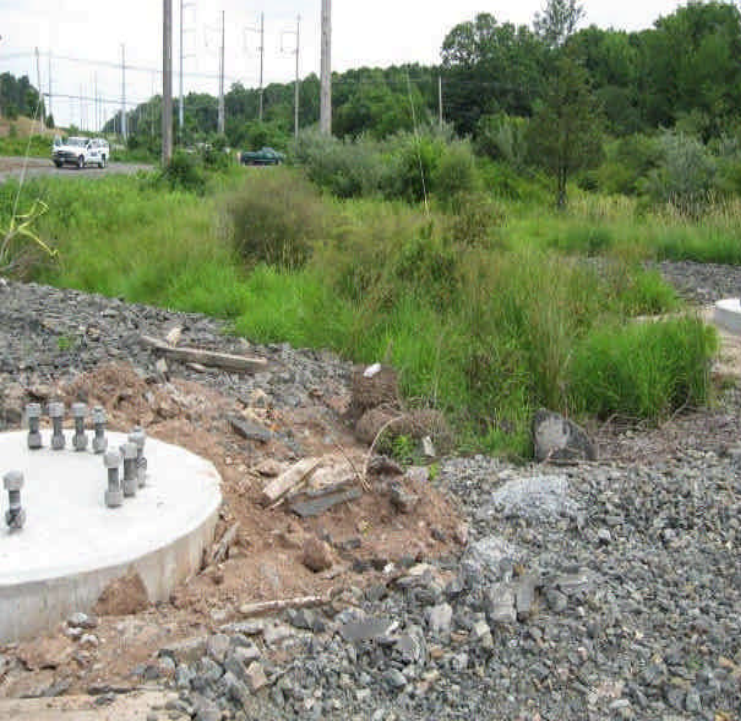
Foundation was placed in a small stream channel off Carpenter Lane. Create a new channel/or provide stream restoration to re-establish the hydrology.
