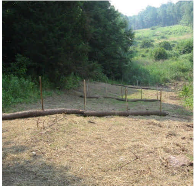
Mulch and filter socks are in place along recently cleared slopes in the Tuttle Ave area.
