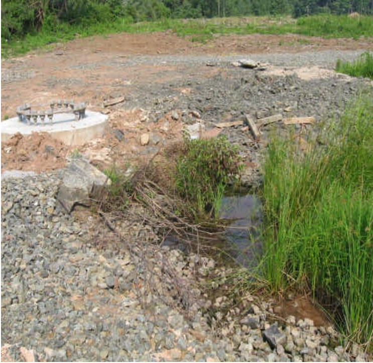
Foundation was placed in a small stream channel off Carpenter Lane. Create a new channel/or provide stream restoration to re-establish the hydrology.
