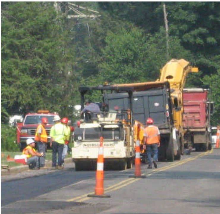
The roadway and trench patch along Old Farms Rd. was being repaved.
