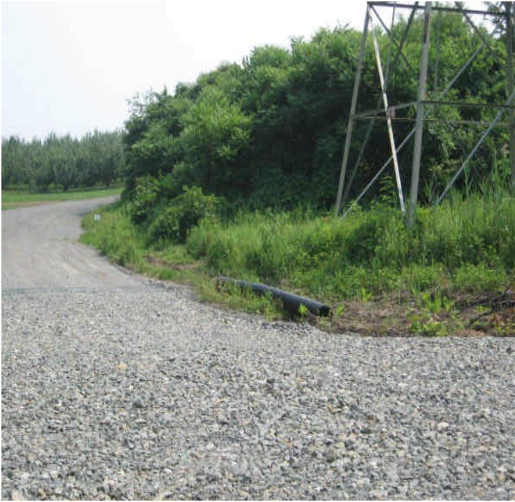
A drainage channel was dug within the apple orchard off Mansion Rd. A culvert appears to be necessary to reduce sedimentation
