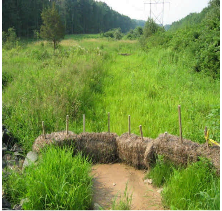
Sediment/turbid run-off was appropriately filtered by a haybale check-dam within wetlands off Carpenter Lane. Remove sediment when feasible to restore capacity.
