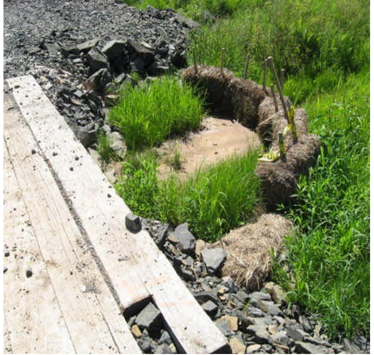
Sediment/turbid run-off was appropriately filtered by a haybale check-dam within wetlands off Carpenter Lane. Remove sediment when feasible to restore capacity.
