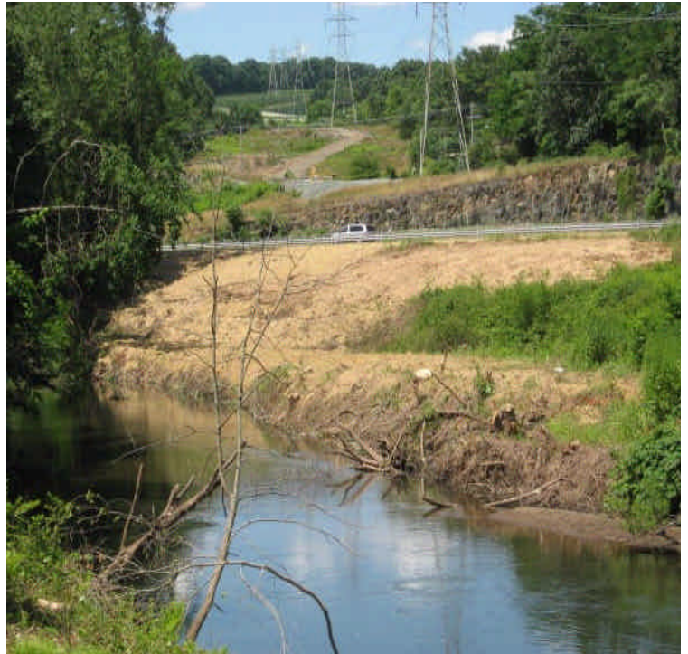
Mulch in place on the slope off Merritt Parkway, adjacent to the river. Monitor carefully for any erosion and install erosion control mats if necessary. Root systems remain in place.
