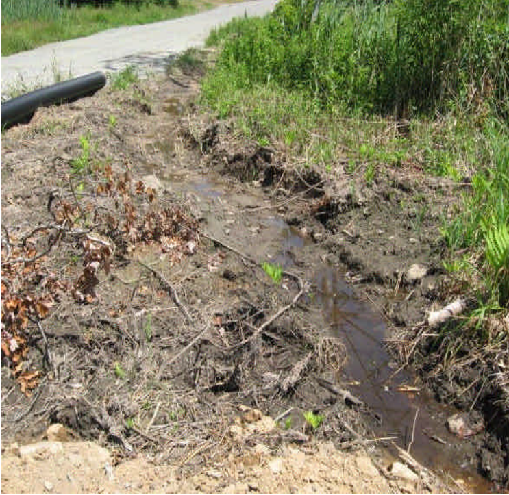
A drainage channel was dug within the apple orchard off Mansion Rd. A culvert appears to be necessary to reduce sedimentation
