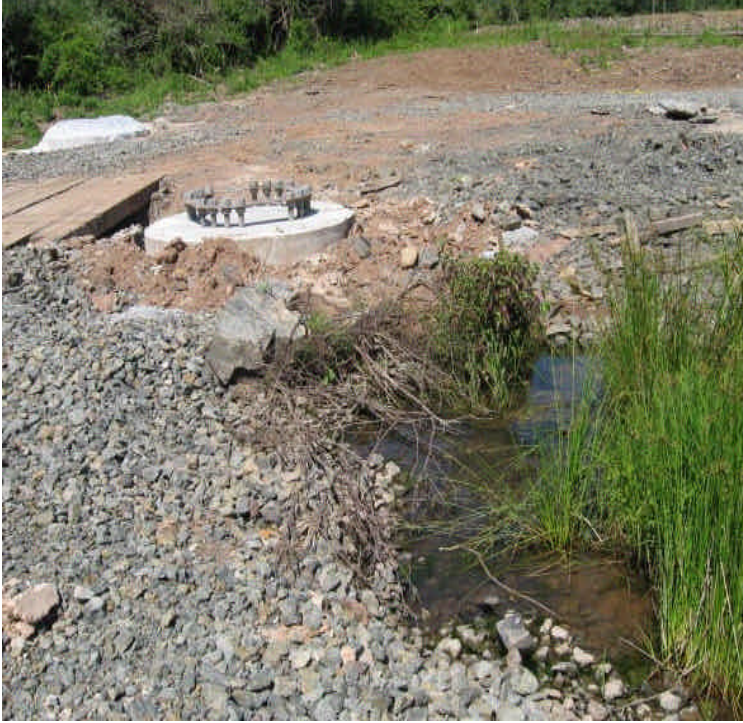
Foundation was placed in a small stream channel off Carpenter Lane. Create a new channel/or provide stream restoration to re-establish the hydrology.
