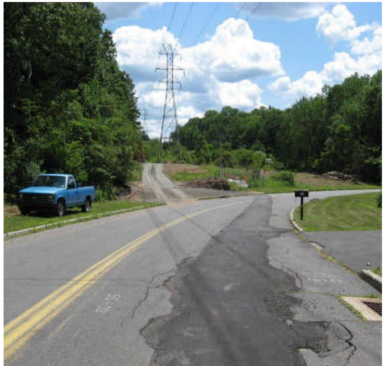
The trench patch along Old Farms Rd. still needs repair in some locations. A new pad site was being constructed.
