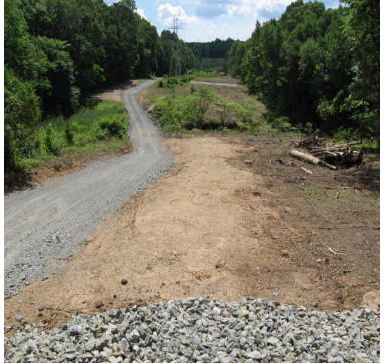
Access road has been installed off of Tuttle Ave. Filter socks, hay mulch and seed remain in place for control and stabilization
