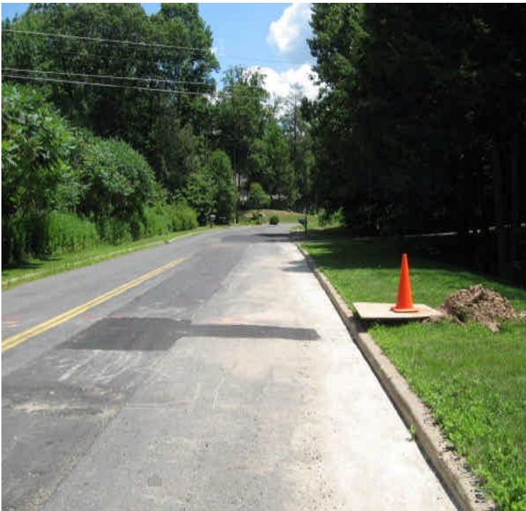
Sediment accumulation was noted in the gutter along the roadway on Old Farms Rd.
