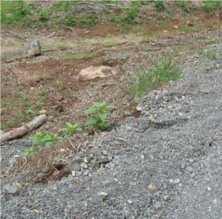
Ruts/washouts are occurring along a steep slope in the access road off Black Walnut Drive.
