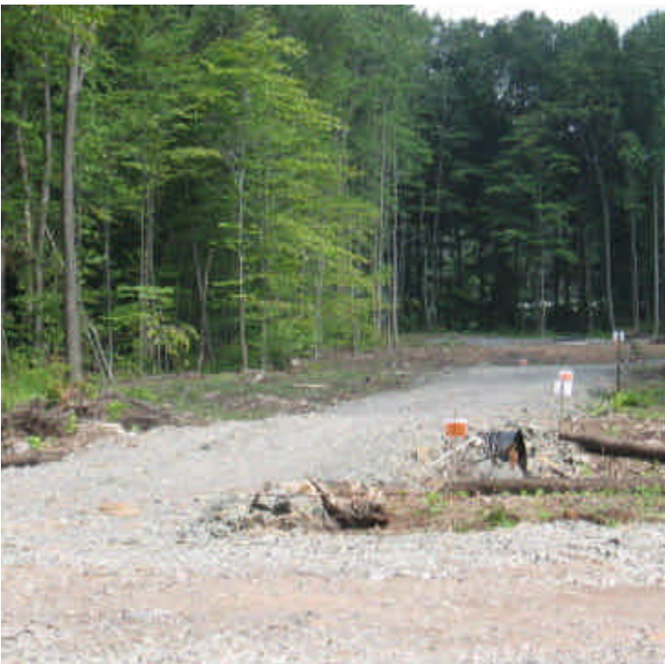
Environmental controls are in place at the wetland crossing and along the access road near the contract shipping/receiving yard. Monitor flow from the culvert for turbidity and adjust controls as needed.
