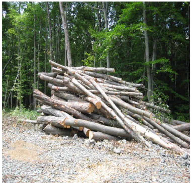
View of the remaining timber stockpile to be removed from the site.
