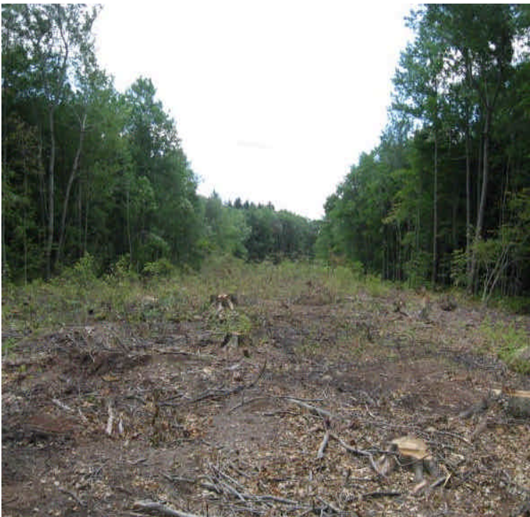
View of the sensitive crossing in the ROW that was recently cleared via helicopter and low impact techniques. Stumps and low growing vegetation were retained to stabilize soils.
