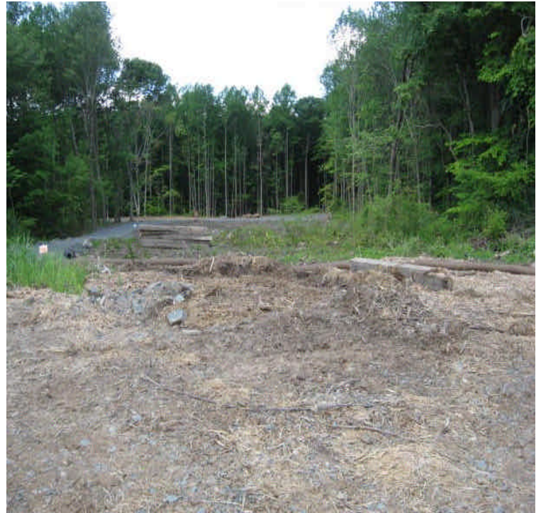
Site entrance within the receiving yard. Timber mats were stockpiled in/adjacent to a wetland area and should be relocated
