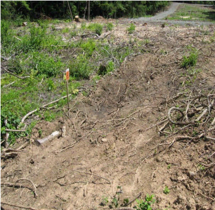
Water was no longer flowing into the pond from the equipment ruts created between Rte 17 and Black Walnut Drive. Controls are still needed. Also, confirm that the “entering wetland” sign is actually at the boundary and not within the wetland.
