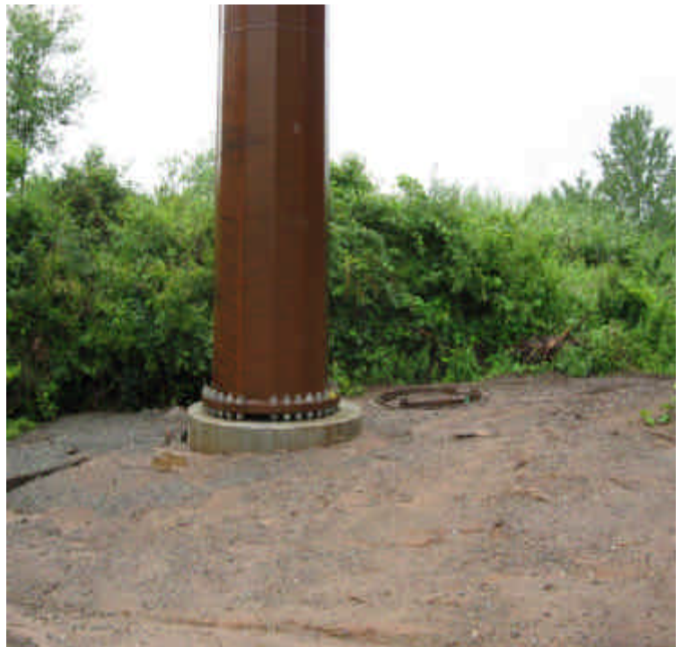
Pole installed off Durham Road. Sediment accumulation was noted on timber mats in the wetlands. Remove sediment to the extent feasible and install controls where needed.
