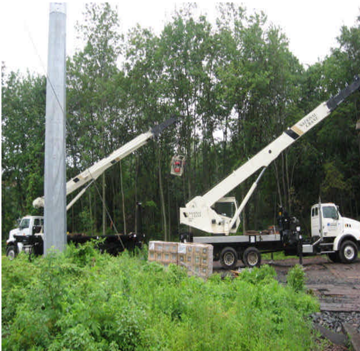
Two pieces of equipment were parked on mats within wetlands off High Hill Road. Avoid equipment storage in wetlands, even if it is temporary
