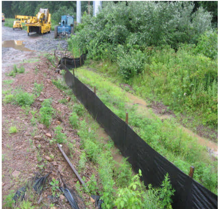
Turbid water flowing from the access road, through controls, and off site to the sediment trap/basin east of Beseck SS.
