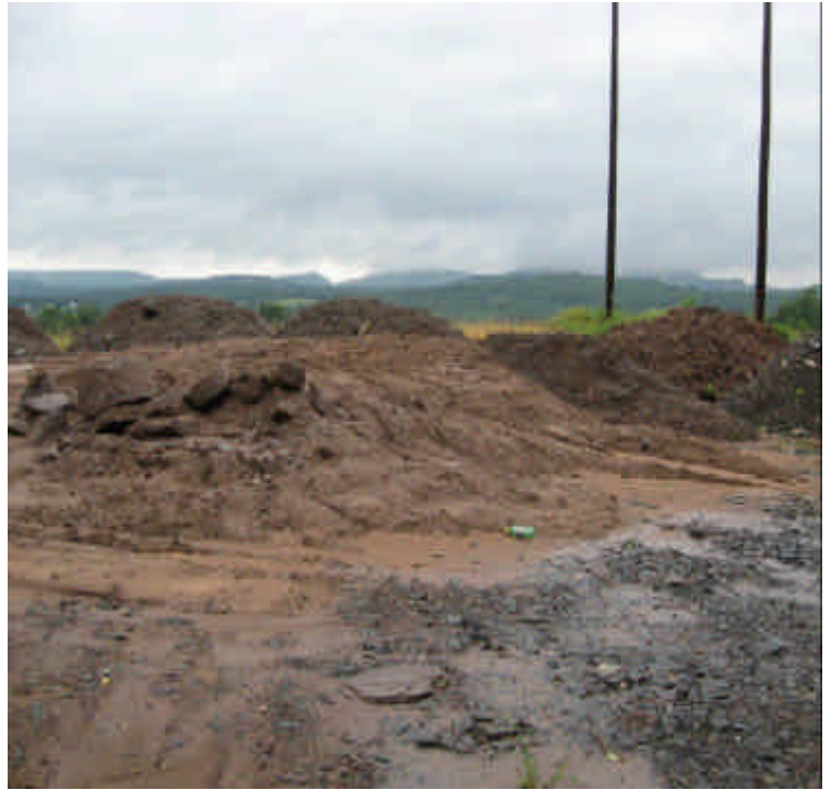
View of soil stockpiles resulting from foundation drilling between Little Lane and the Durham Transfer Station off Cherry Hill Road. Ensure that soil is contained appropriately.
