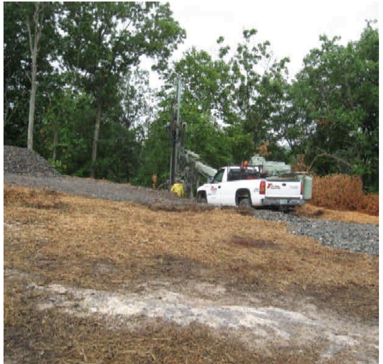
Crews have been spreading mulch along previously disturbed areas west of Scovill SS off Rte 9. Photo also shows a view of foundation drilling occurring in the area.
