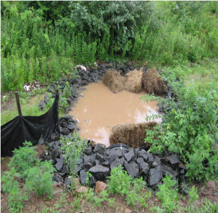
View of the sediment trap east of Beseck SS. The trap is also receiving turbid water from the switching station and does not have the capacity during larger rain events.
