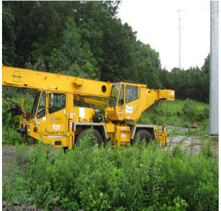
Equipment was parked on mats within wetlands north of Beseck SS. Equipment was moved the next day and used for line puling in this area. Avoid equipment storage in wetlands, even if it is temporary.
