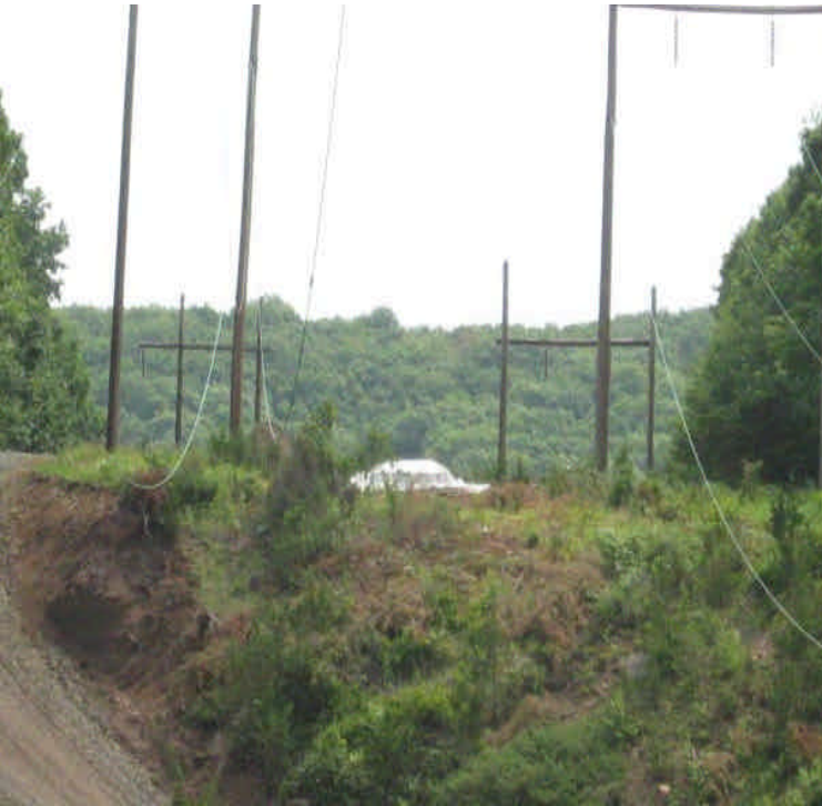
The foundation was installed off Black Walnut Drive, upgradient from Ball Brook.
