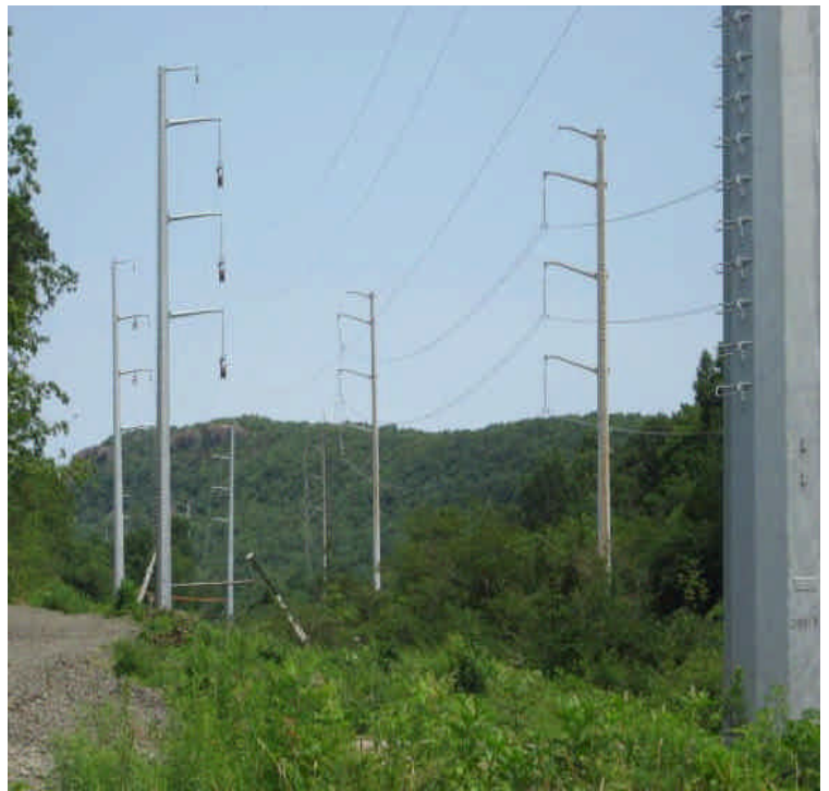
View of line pulling work on recently installed poles off High Hill Rd.
