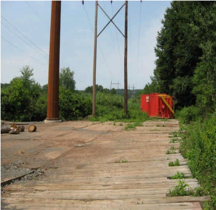
Timber mats remain within wetlands off Durham Rd. A settling tank is also in place here.
