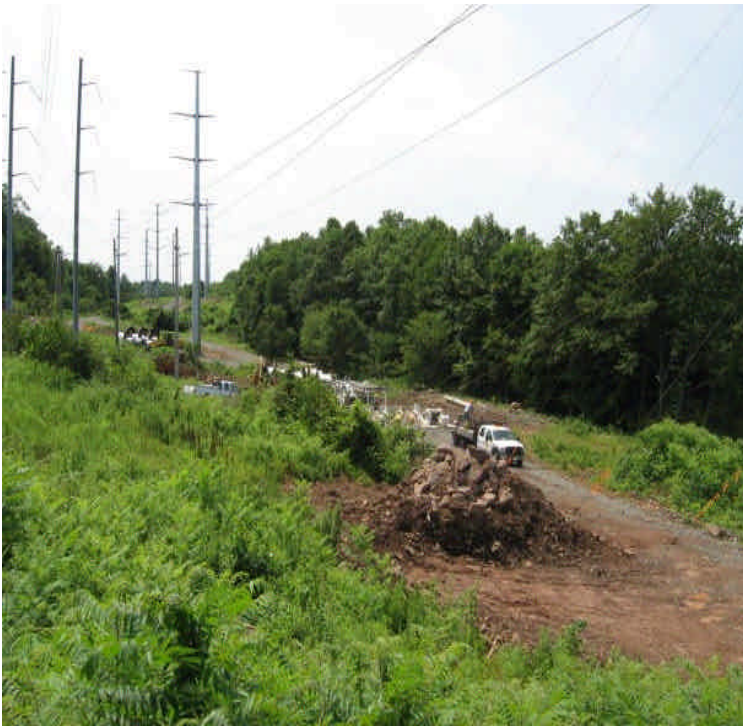
Line pulling was occurring in the ROW west of East Meriden SS.
