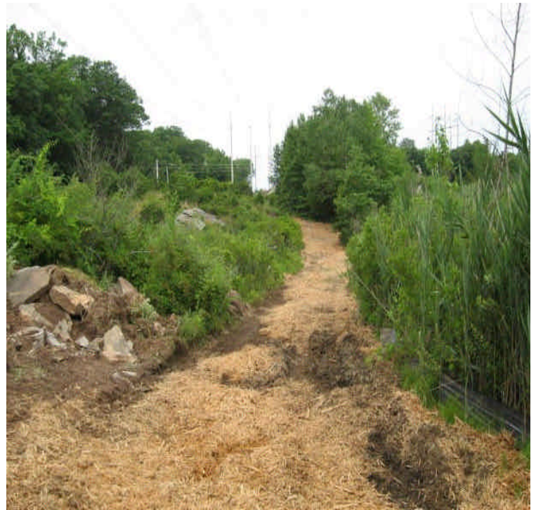
Crews have been spreading mulch along previously disturbed areas west of Scovill SS off Rte 9.
