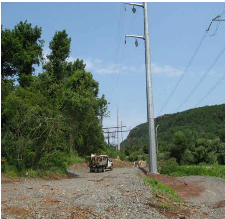
View of the pad site with the new pole off East Main Street.
