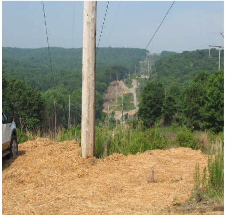
Crews were spreading mulch along exposed soil areas west of Scovill SS off Rte 9.
