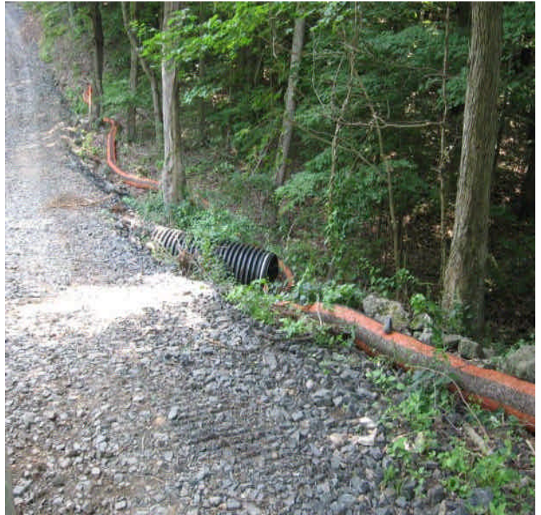
View of the wetland crossing off Black Walnut Drive. Filter socks remain in place.
