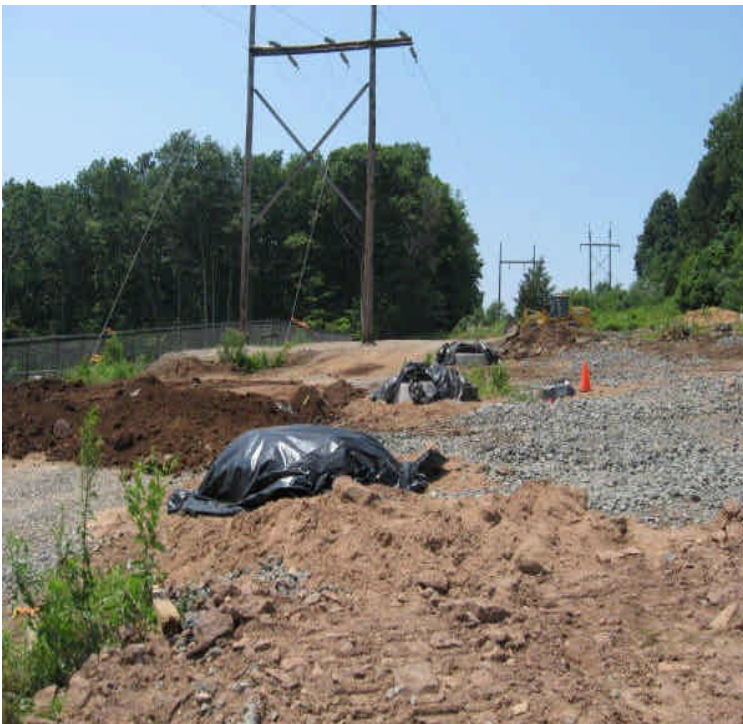
View of pad and road grading and foundation installation north of Beseck SS.
