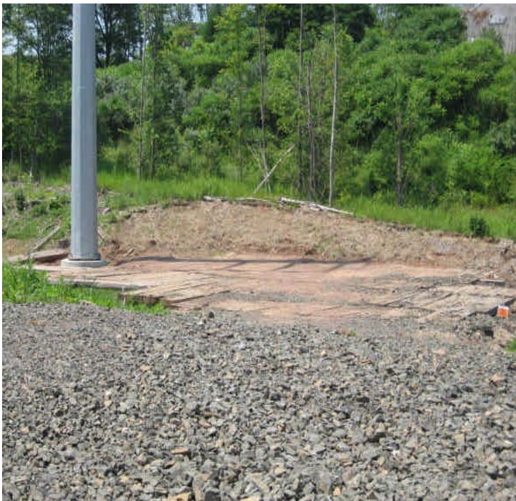
Timber mats and controls at pole within wetlands off High Hill Road. Grass growth was noted on slope.
