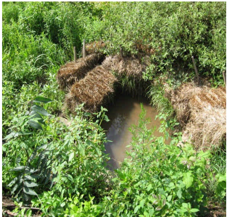
Turbid water was observed within the culvert. Clear water was observed entering the wetlands. The haybales help to filter out the sediment. Evaluate whether the amount of sediment accumulation justifies the disturbance needed to remove it, once the water subsides.
