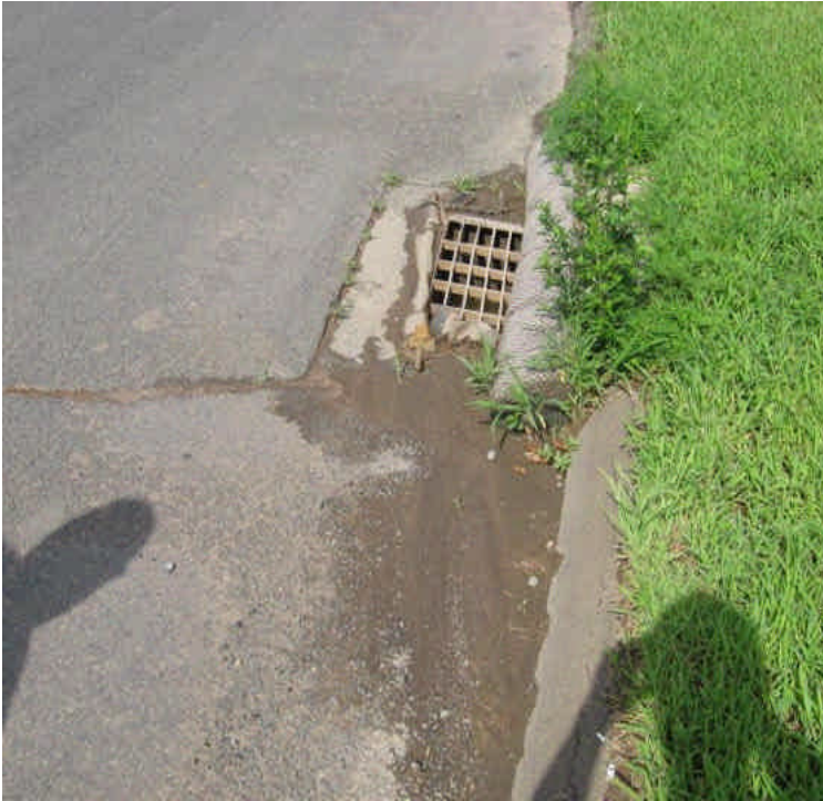
Sediment accumulation was noted in the gutters along Carpenter Lane as a result of heavy rains. Remove sediment from roadway on a regular basis.
