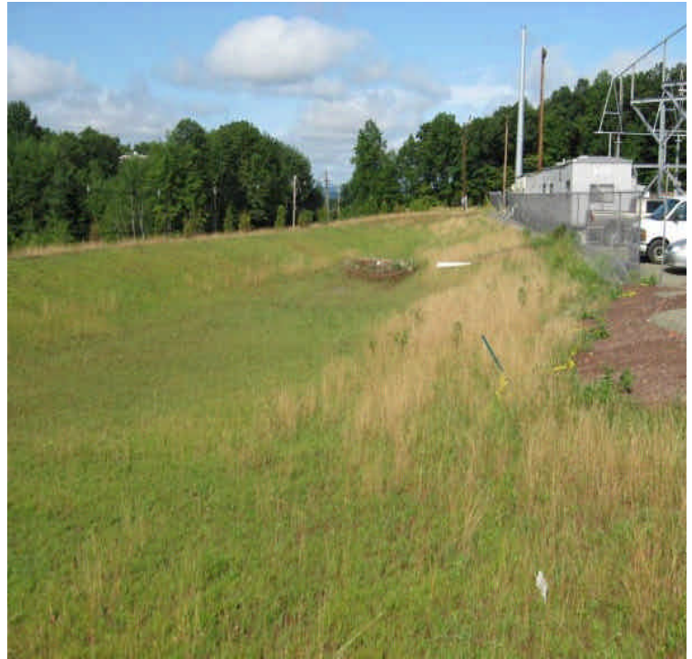
Haybales and controls remain in place at the inlet of the detention basin. Grass cover continues to establish well in hydroseeded areas. The basin appears to have 75% vegetative cover and is stable.
