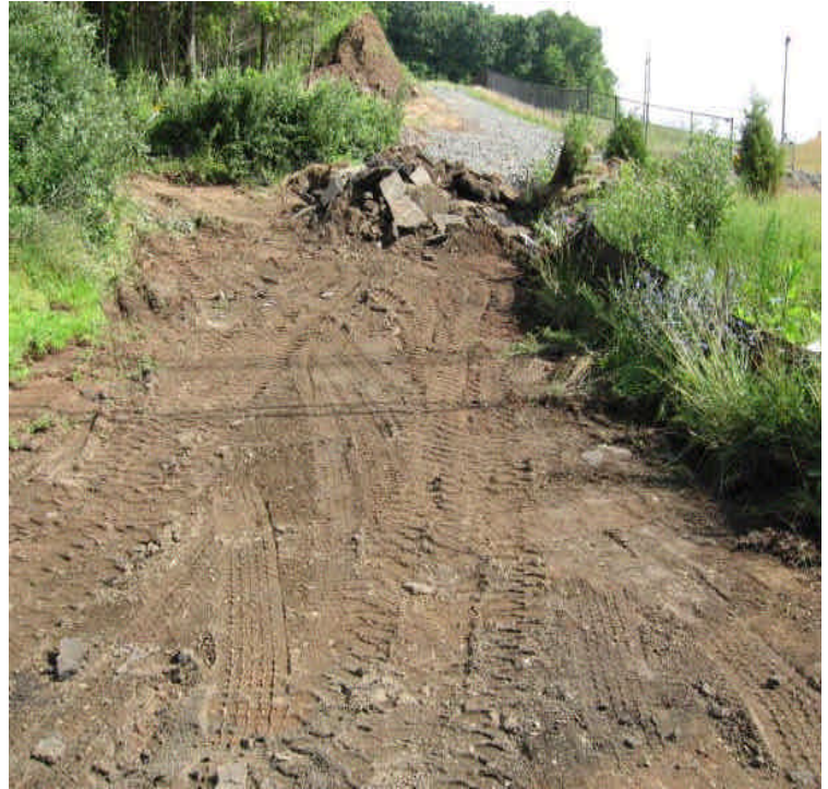
Pavement being removed from original driveway entrance. Add controls upon completion of grading. Stabilize exposed soil when feasible.
