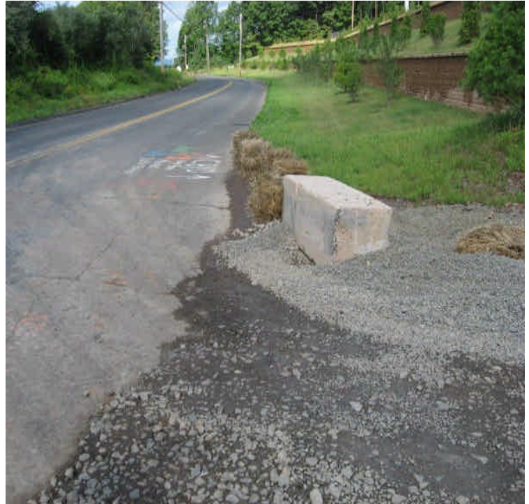
View of the eastern site exit at Carpenter Lane. Haybales, a concrete block, and additional stone were in place at the corner of the drive, in an effort to contain run-off.
