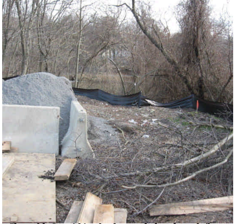
Photo of the Imperial Ave. lay-down yard where the stockpile of crushed stone is starting to overflow its containment area. Material is still contained to site at this time but prevent migration to adjacent resource areas.
