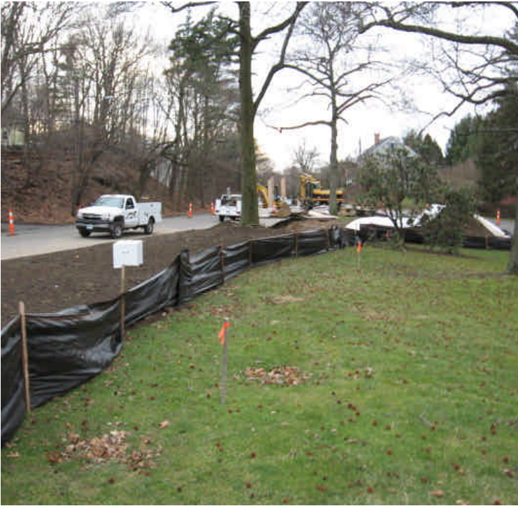
Photo of trenching activities along Pequot Ave. A portion of the trench has been backfilled and loam applied. Area remains to be and are stabilized.
