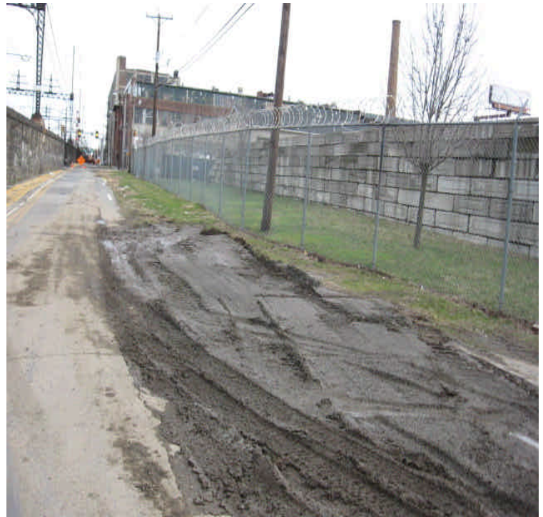
Photo of an area that has been re-graded along the shoulder of Railroad Ave. Exposed soils should be stabilized.
