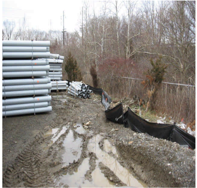
Photo of the perimeter erosion controls in the King's Highway lay-down yard. Sections of the fence have been compromised and are in need of repair.
