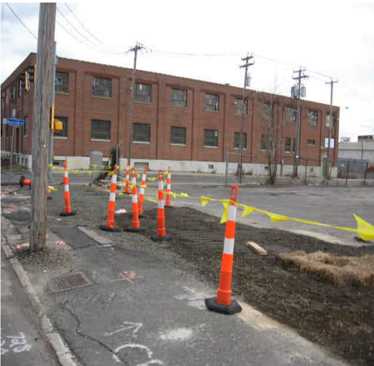
Photo of a completed section of trench along Railroad Ave. near the intersection with Bostwick Ave.
