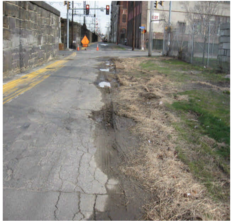
Some soil from the shoulder of Railroad Ave. is migrating into the roadway and is being tracked by vehicles.
