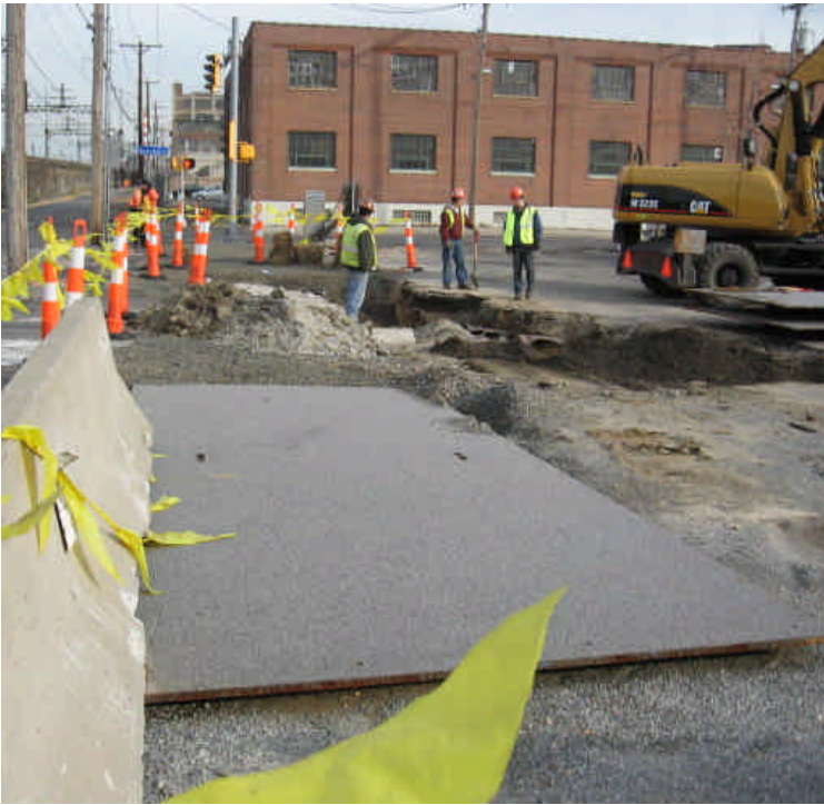
Trenching activities along the shoulder of Railroad Ave. near its intersection with Bostwick Ave.
