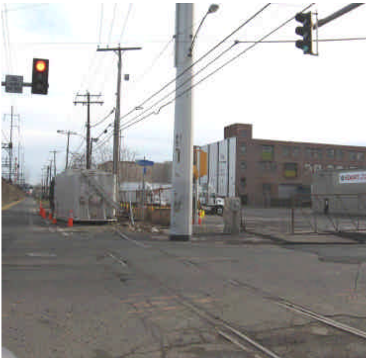
Photograph of trenching activities and frac tanks stored on Railroad Ave. at its intersection with Howard Ave.
