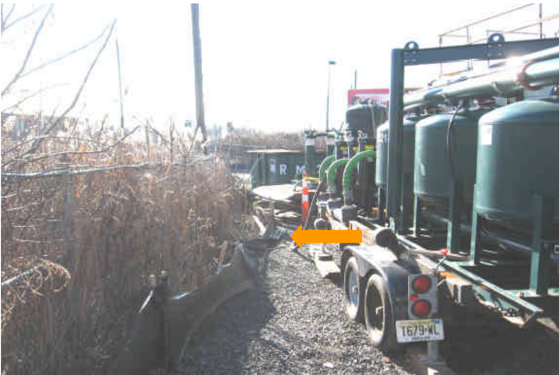
Photo of a small section of the perimeter silt fence that is in disrepair along the side of the yard that is adjacent to the resource area.
