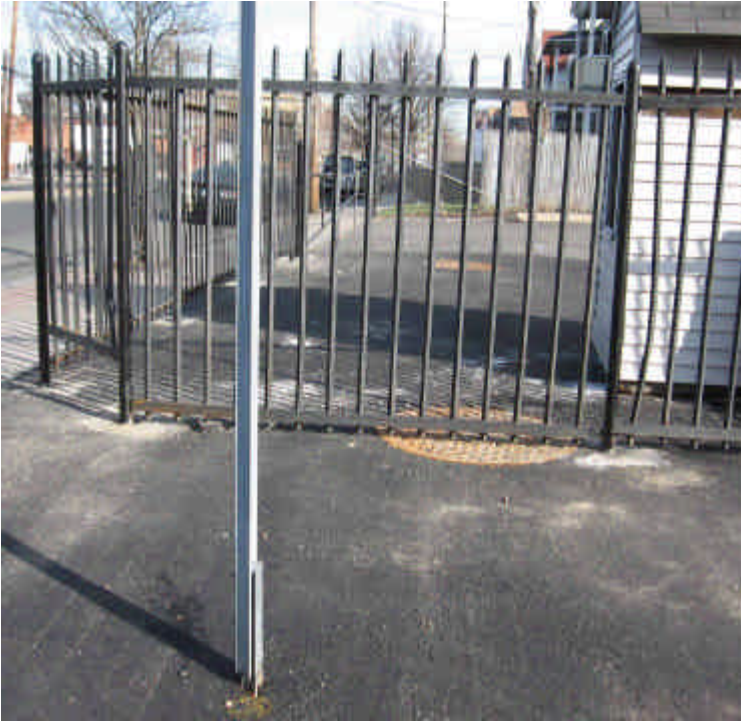
Photograph of Vault #41. Installation is complete and the area has been restored.
