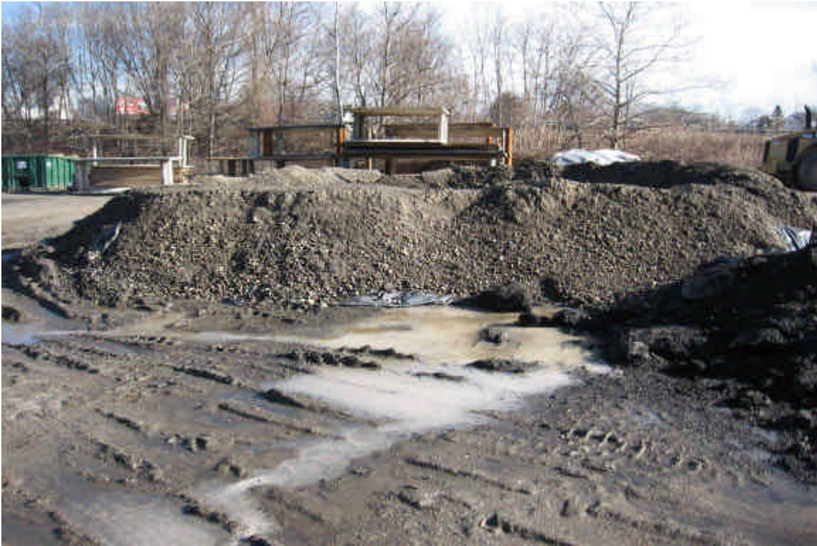
Photo of the concrete washout basin where washout was not fully contained. Repair as feasible.
