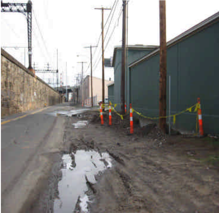
Photograph taken on Railroad Ave. between Wordin Ave. and Iranistan Ave. of soils that have been exposed by construction activities. Temporary stabilization (mulch) is recommended.
