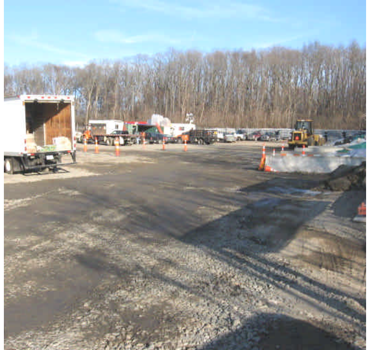
The Milford lay-down yard is being used to divert traffic around Vault #6 installation activities.
