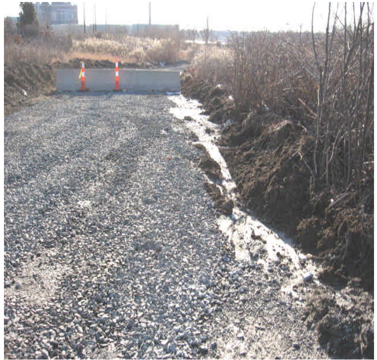
Photo of an uncontained concrete washout released along the access road near station #1055. The concrete should be removed and properly disposed of. Remind drivers to use appropriate locations.
