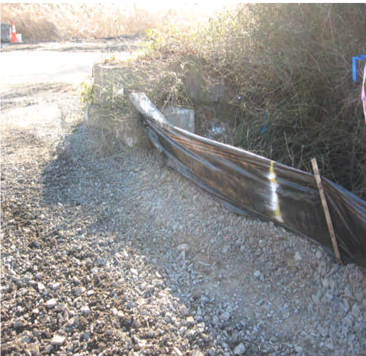
The silt fence west of station #1052, immediately adjacent to construction entrance and resource area. Ensure that the fence is toed-in and provide maintenance as necessary.
