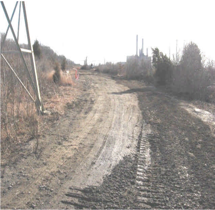
Photo taken near station #1058. A mixed aggregate base was applied as cover on the trench to stabilize the existing access road
