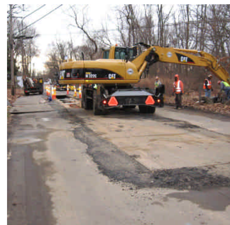
Photograph of trenching activities from station #1033 to 1039. No issues were noted at the time of inspection.
