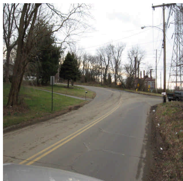
Sediment is being tracked onto Nungateck Ave. from the cross-country roads. Sweep roadway as necessary, and prevent further tracking as feasible.
