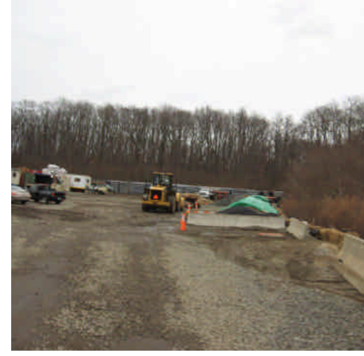
Overview photo of the Millfield lay-down yard. No issues were noted at the time of inspection. Erosion controls remain at the perimeter of the yard.
