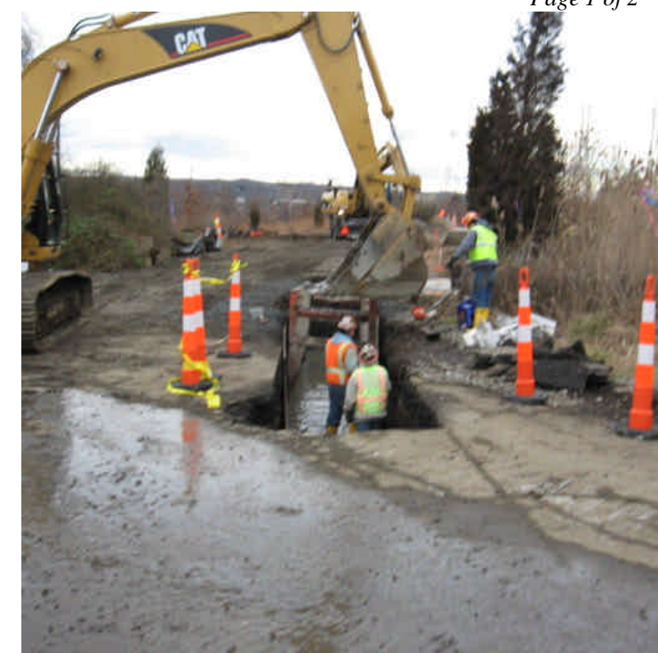
Photograph of trenching activities at station #1055. Water in the trench is not being pumped at this time.
