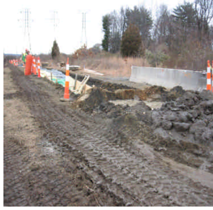
Photograph of trenching activities from station # 1054 to 1050. A basin has been constructed to receive/contain concrete washout.
