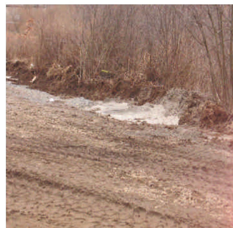
An uncontained concrete washout was noted along the ROW. This concrete should be removed and properly disposed of. Rental drivers to continue using designated, contained area.
