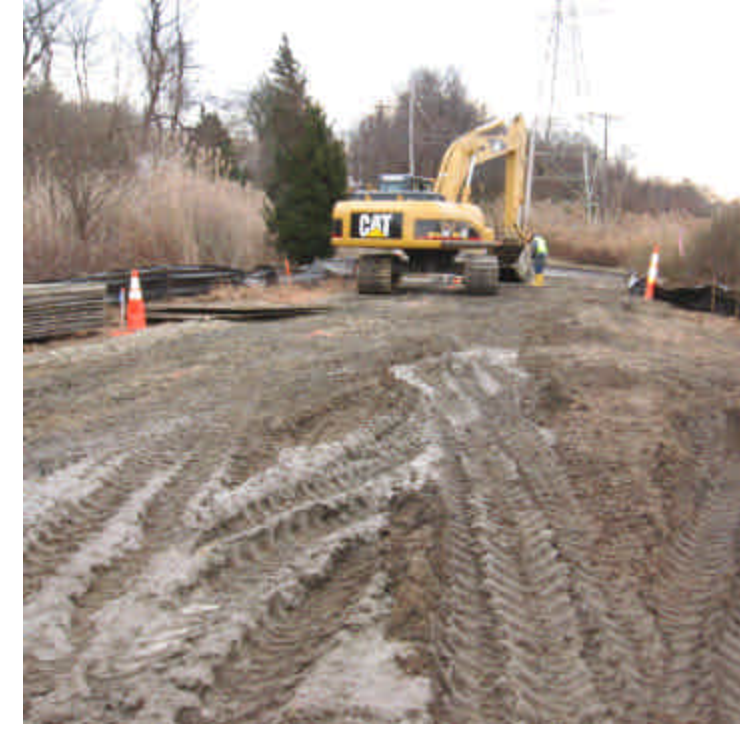
Erosion controls (silt fence) have been installed to protect wetland areas on either side of access road.
