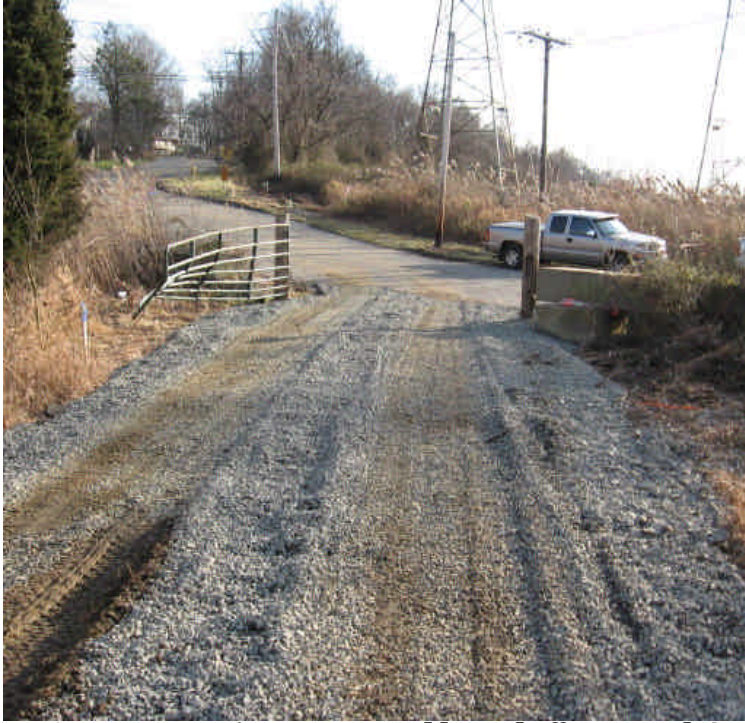
Stone construction entrance pad located off Naugatuck Ave. to access station 1050 to 1058.
