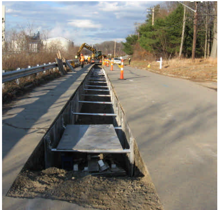
Trenching activities from station 1089 to 1097. All catch basins near construction activities are protected.
