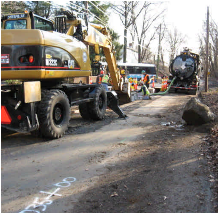
Trenching activities from station 1033 to 1037. Vac truck is dewatering groundwater from trench. Roadway should be swept of sediment at the close of the workday and as sawcut slurry is created.
