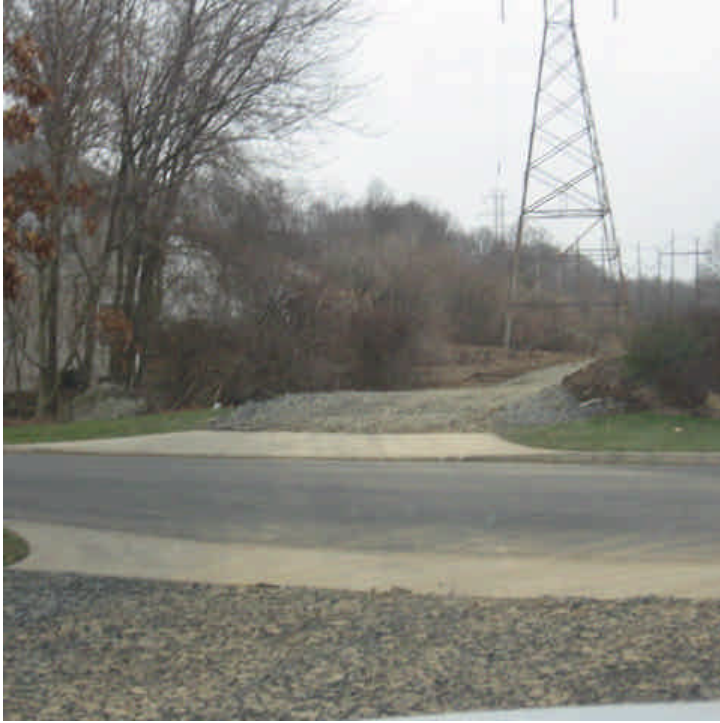
Access road construction appears to be complete off Lexington Lane and the road remains free of major sediment tracking.
