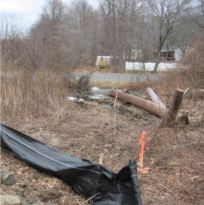
The first wooden structure has been dismantled within the ROW off Pine Tree Dr. Pieces were being stored in the small wetland area here. Remove and place in a more appropriate location.
