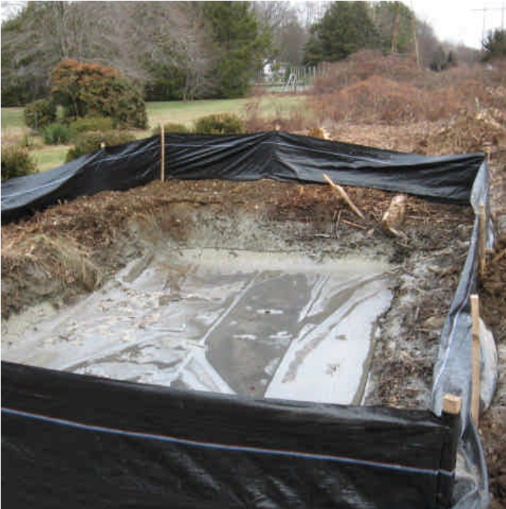
View of one of the dewatering basins constructed within the ROW off Treat Lane. All sediment is contained here.
