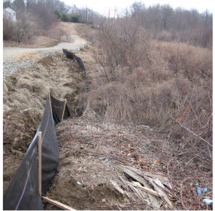
Silt fence was installed adjacent to the wetland located to the south of the access road off Lexington Lane (east).
