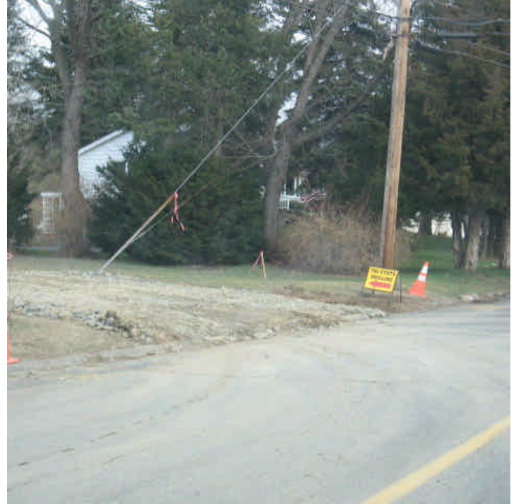
Minor sediment tracking was noted off Treat Lane this week. It does not appear to have reached any nearby catch basins. Sweep as necessary
