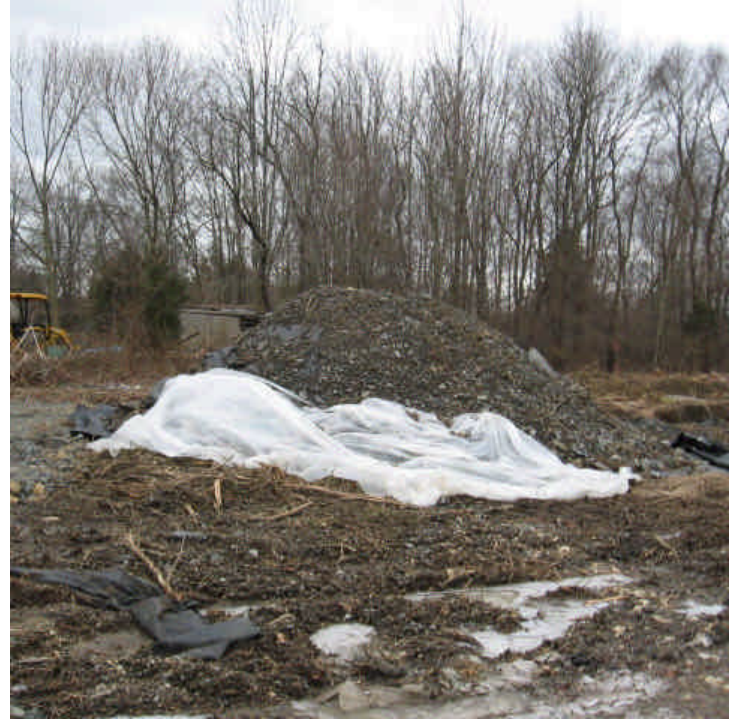
The plastic covering needs to be adjusted on some spoil piles off Sunset Dr.
