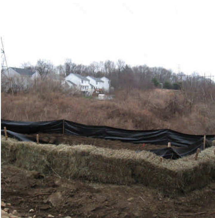
View of one of the dewatering basins constructed proactively within the ROW off Lexington Lane.
