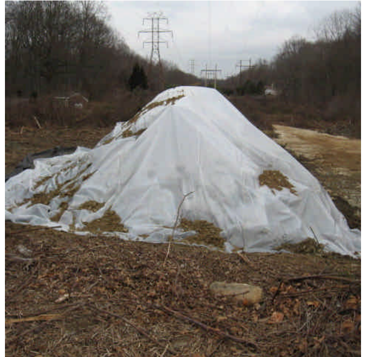
Spoil piles were covered in plastic within the ROW off Treat Lane when drilling was complete.
