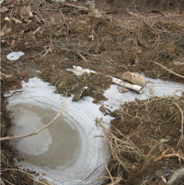
View of the non-project related activities occurring within the ROW off Sunset Drive. A trench was dug and a pipe installed near the first structure foundation.
