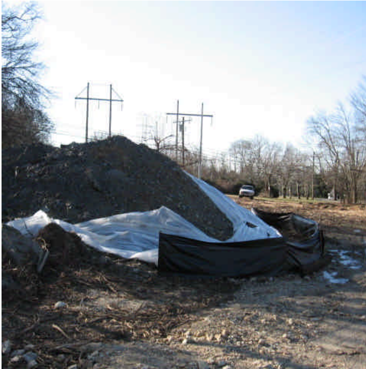
Plastic has slipped from some of the spoil piles off Russell Ave but silt fence remains intact where necessary.
