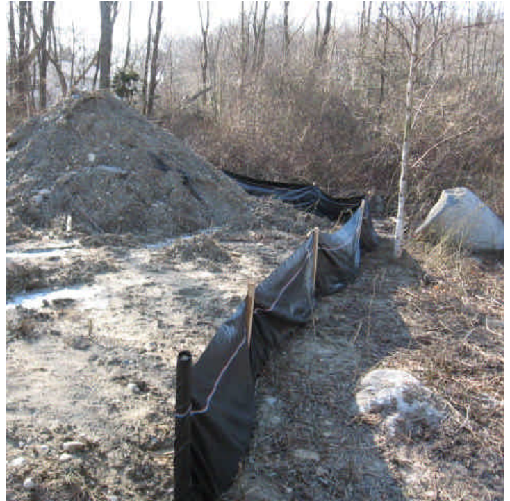
Silt fence remains intact around the spoil pile near the wetland off Overland Drive (west).
