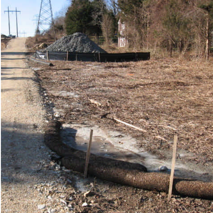
View of the sediment that had breached the controls off Overland Dr. (east). Filter sock check dams have prevented the sediment from migrating further downgradient.
