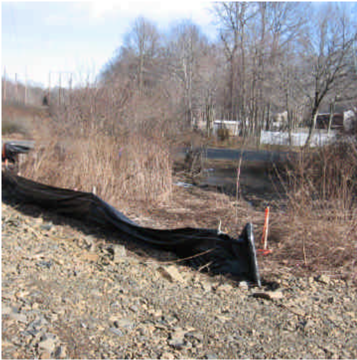
Silt fence remains intact at the small wetland pocket within the ROW off Pine Tree Dr (west).
