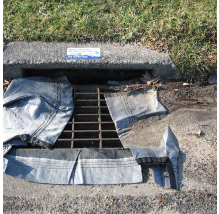
Accumulated sediment was noted around the catch basin on the western side of Overland Dr. Sweep the gutter and roadway as needed.
