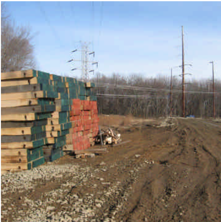
View of the access road within the ROW off Pease Rd in Woodbridge. Timber mats are being stored here for future access.
