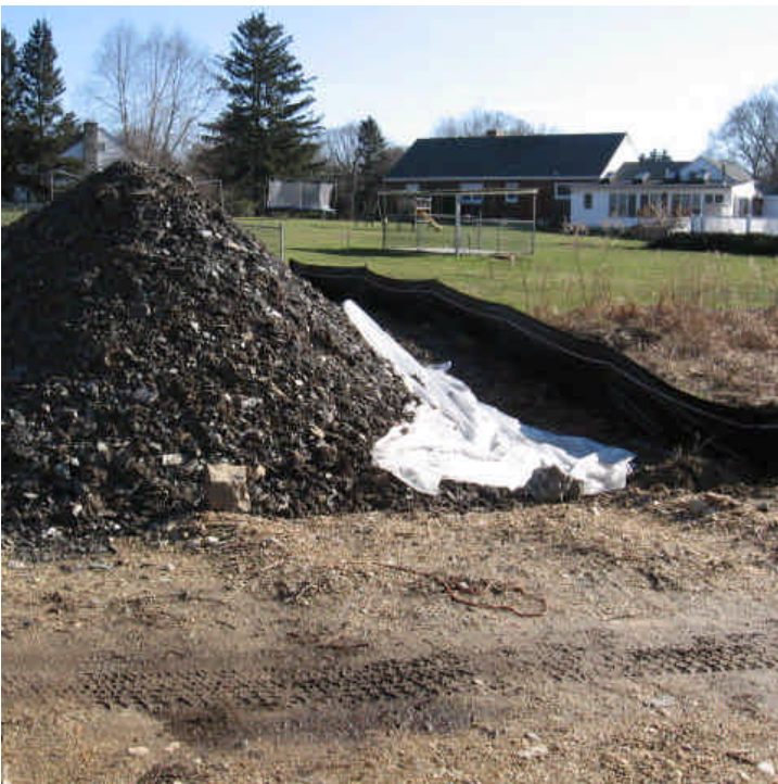
Silt fence remains intact at the spoil pile near the wetland off Sunset Dr. The pile appears contained, but silt fence may need to be extended toward the road.
