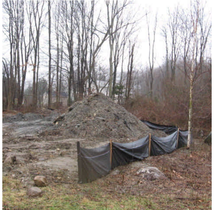
Silt fence was installed at the spoil pile located near the wetland off Overland Drive (west).
