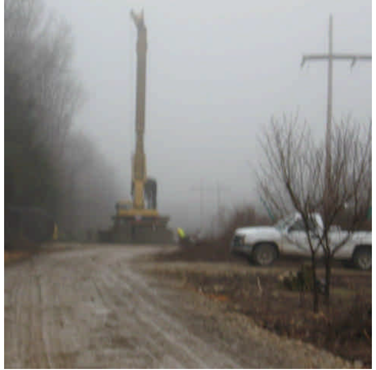
View of the foundation drilling within the ROW located off Route 152 (west).
