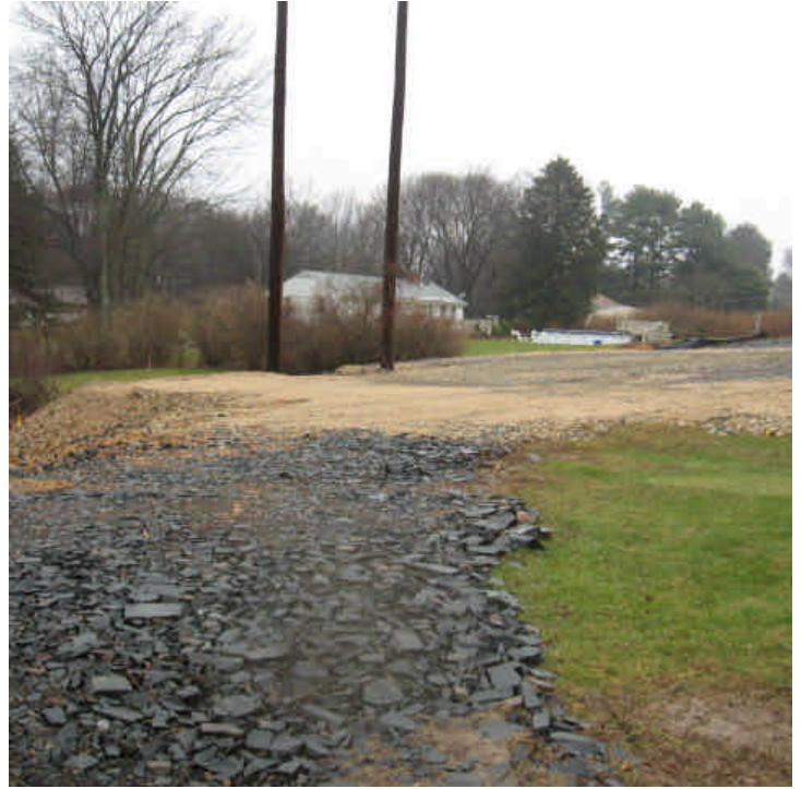
Overall view of the work area within the ROW located off Hunting Hill Place.
