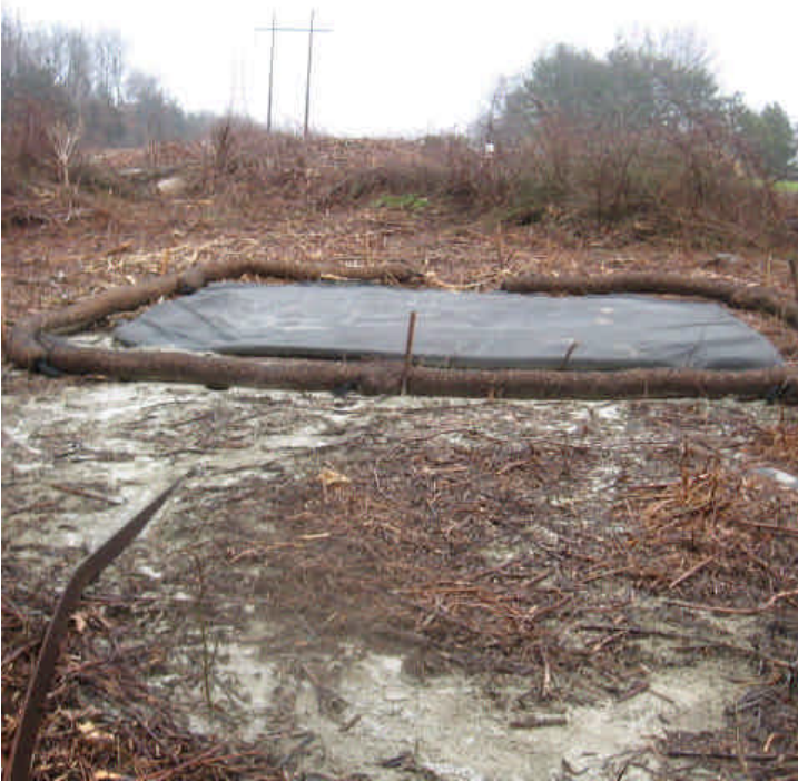
Sediment/slurry remains outside of the controls within the ROW Off Overland Drive (west). It is unlikely that sediment will affect the wetland located downgradient but this should be avoided.
