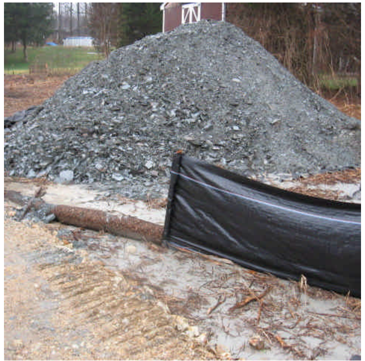
Some sediment/slurry has breached the dewatering controls off Overland Drive (east).
