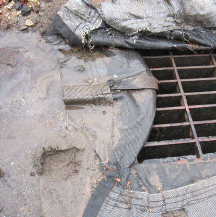
Sediment has built up around the catch basin on Sunset Dr. The Silt-Sak still appears to be functioning properly here. Clear as necessary.
