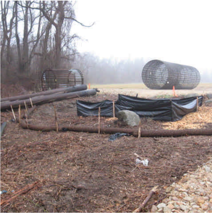
View of a dewatering basin and filter sock check dam within the ROW off Route 152 (east). Continue to ensure controls are adequate to contain slurry.
