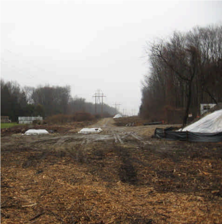
View of the foundation work and spoil piles in the ROW off Russell Ave.
