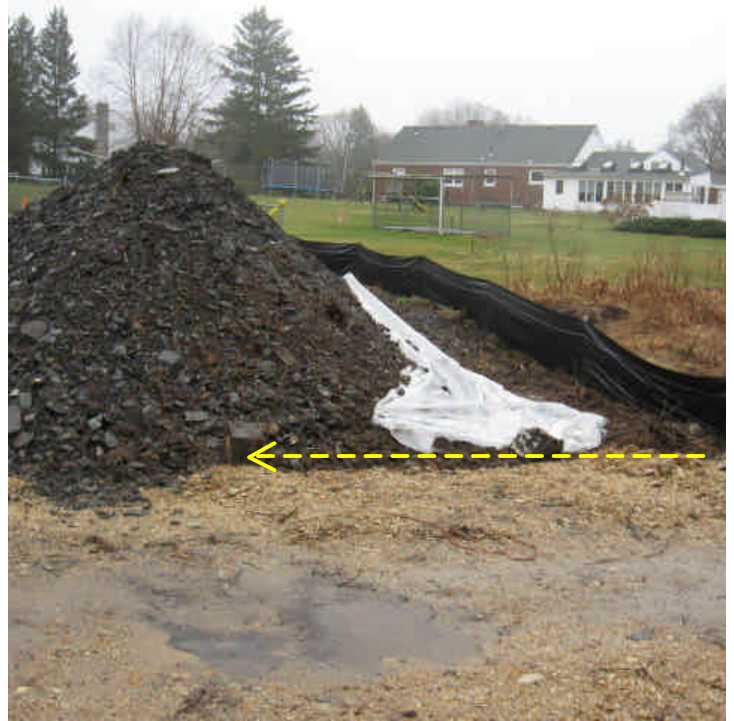
Silt fence was installed between the stockpile and wetland within the ROW off Sunset Ave. The silt fence may need to be extended toward the road here.
