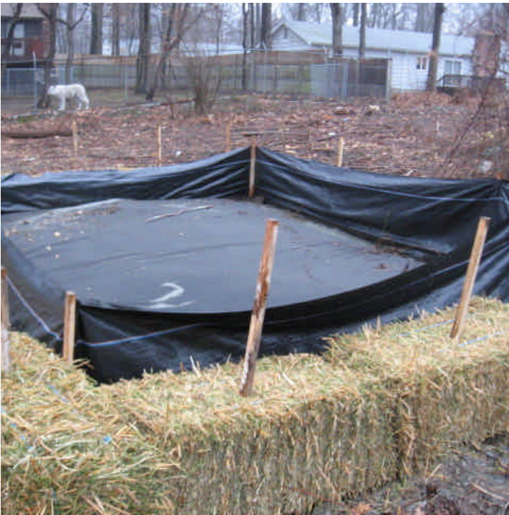
View of one of the many dewatering basins located within the ROW off Route 152 (west).
