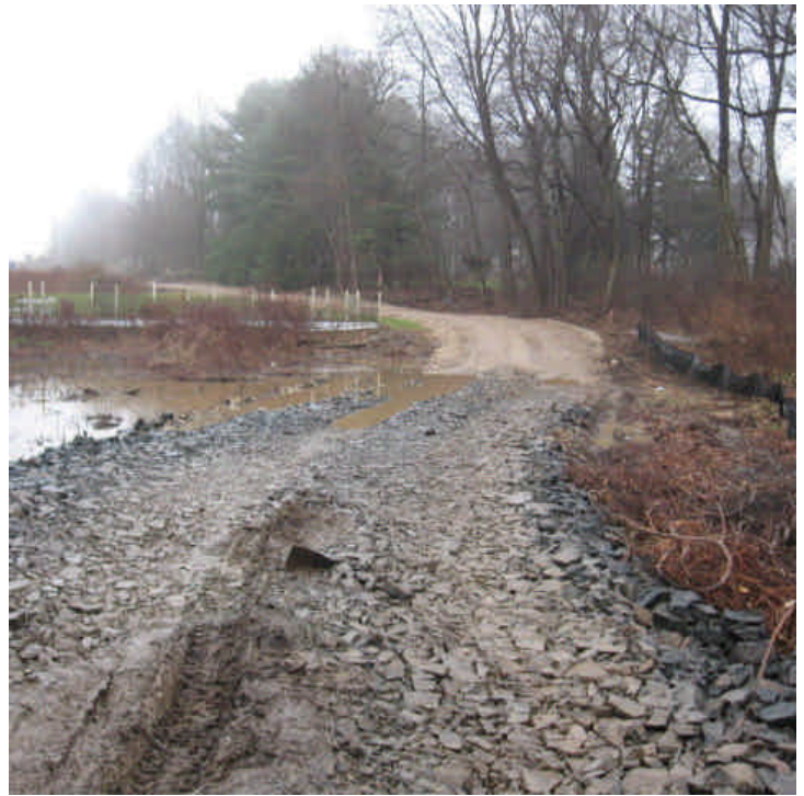
View of the water pooling at the access road located across from the wetland area off Route 152 (west). Additional stone may be needed in the access road here to reduce turbidity.
