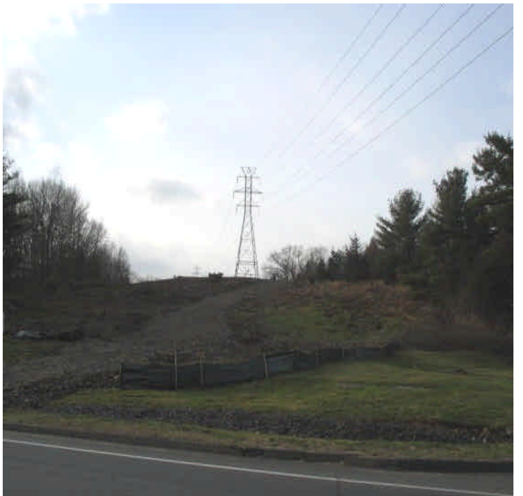
Section of silt fence is in slight disrepair along South Turnpike, however no immediate issues were noted. Continue to monitor slope for erosion.
