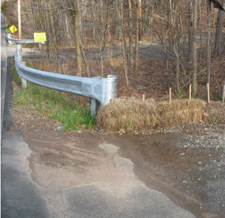
Sediment accumulation should be removed from the haybales at the ROW entrance off Mansion Rd when feasible although no immediate issues were noted.
