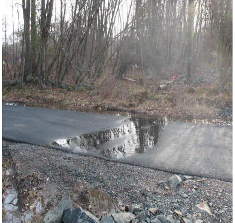
Continue to monitor run-off and sheet flow seeping from non-federally jurisdictional wetland crossings off Old Farms Rd. Some turbid water has been observed reaching the roadway. Also, evaluate past and current hydrology here as water was pooling across some driveways.
