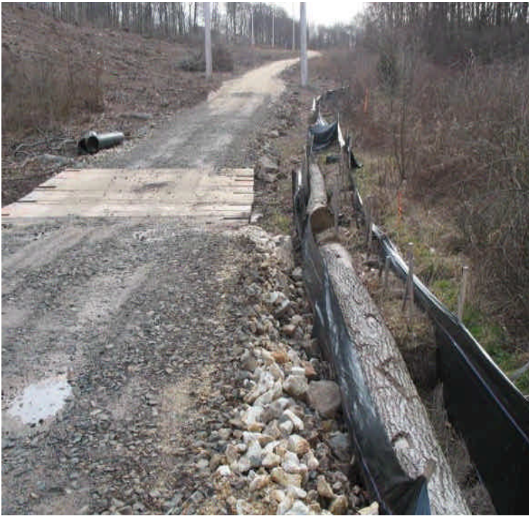
Access road, timber mats, and erosion controls off High Hill Road at a non-federally jurisdictional wetland crossing
