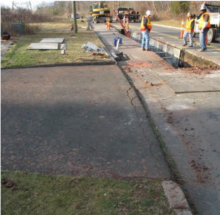
View of trenching on Old Farms Road for underground work. Minor sediment was noted on adjacent driveway. Adjacent wetlands showed signs of sedimentation. Continue to sweep roadway or driveways as needed, especially as soon as sawcut slurry is created.
