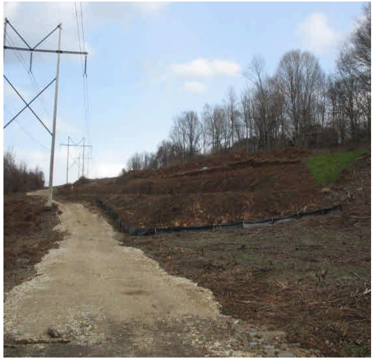
New staging areas prepared for pole construction. Temporary stabilization measures (mulch) are in place. Grading was performed to repair washouts.
