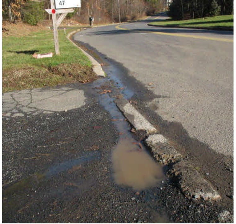
Continue to monitor run-off seeping from non-federally jurisdictional wetland crossing off Old Farms Rd. Some turbid water has been observed reaching the roadways.
