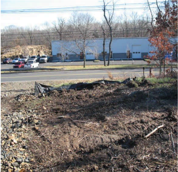
Section of silt fence is in slight disrepair along South Turnpike. Continue to monitor slope for erosion.
