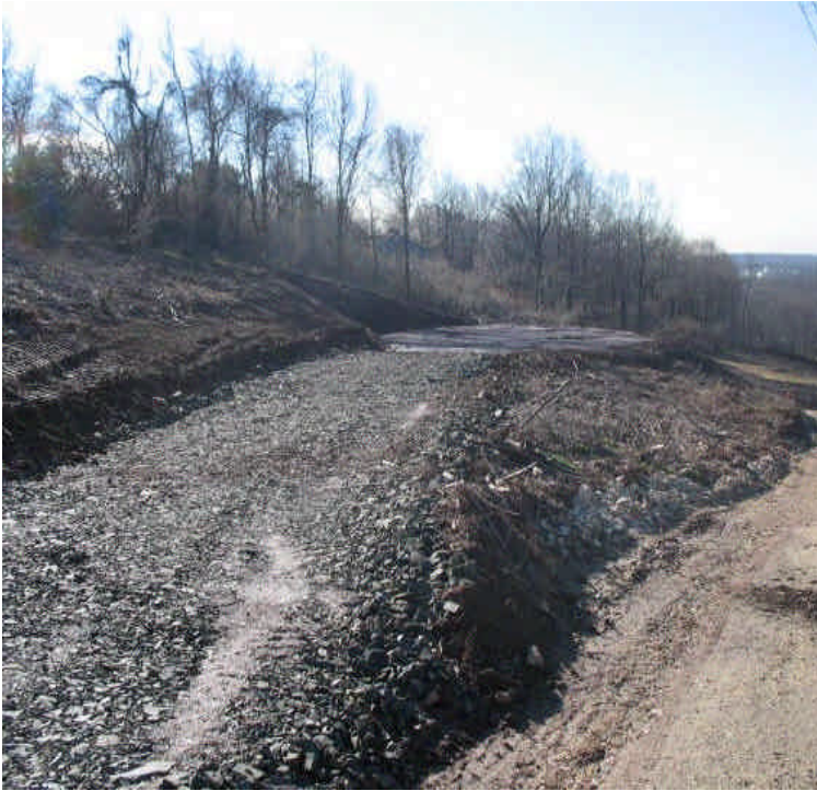
New staging areas prepared for pole construction. Temporary stabilization measures (mulch) are in place.
