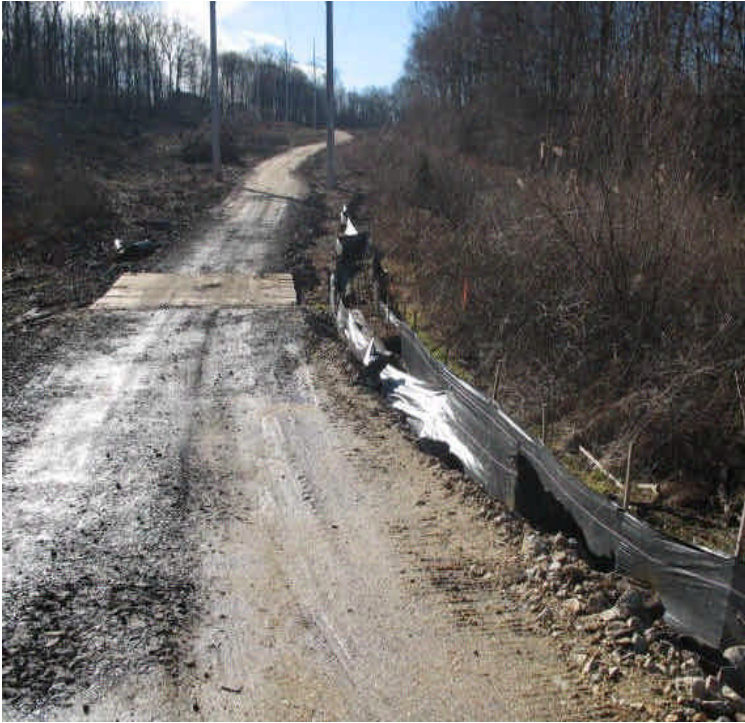
Access road, timber mats, and erosion controls off High Hill Road at a non-federally jurisdictional wetland crossing
