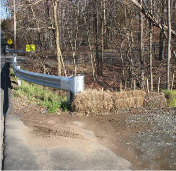
Sediment accumulation should be removed from the haybales at the ROW entrance off Mansion Rd.
