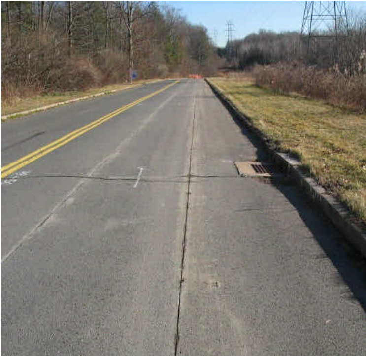
Old Farms Road sawcut in preparation for underground work. One catch basin still needs protection. Adjacent wetlands showed no signs of sedimentation. Continue to sweep roadway as needed, especially as soon as sawcut slurry is created.
