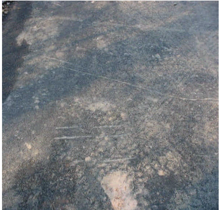
Plywood was used to protect driveways from equipment crossing on the ROW off Old Farms Rd. Only minor tracks were noted on a few driveways.
