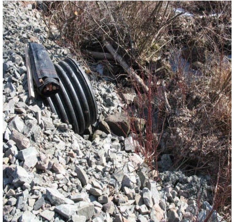
Stone and culvert used to cross a small stream off Powder Hill Rd. No sediment was observed leaving the site. Original conditions will need to be restored when work is complete.
