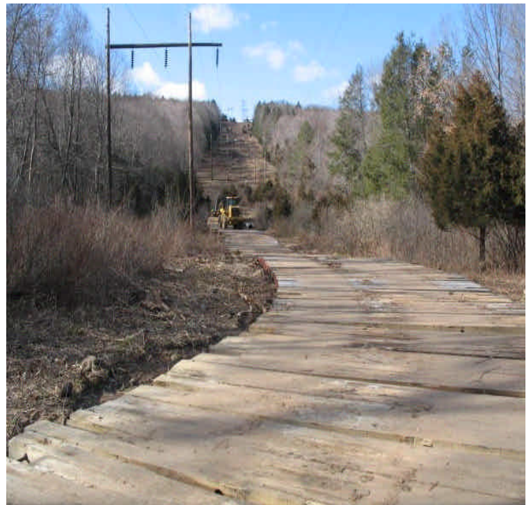
Timber mat installation for access west of Powder Hill Rd. The mats traverse wetlands, uplands, and small streams.
