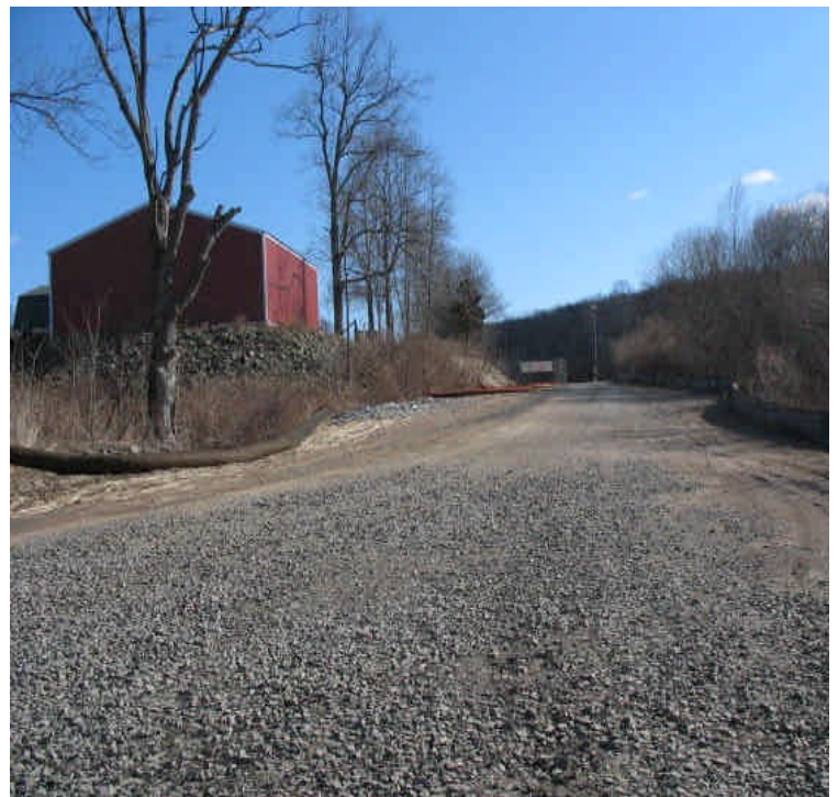
Silt fence, fiber rolls, and hay mulch have been added as a buffer around the perimeter of the contractor receiving yard.
