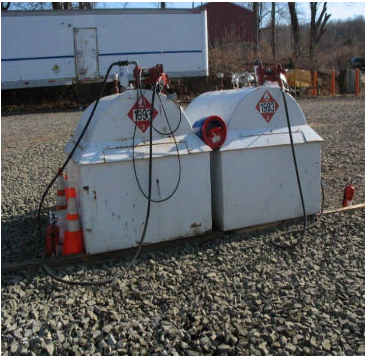
The fuel storage tanks remain in place on the new spill pad and nozzles are contained. Small drip stains were noted and are contained to the stone.
