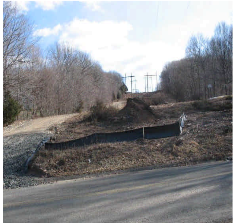
Access road and ROW off Arbutus Street. No run-off noted during the inspection.
