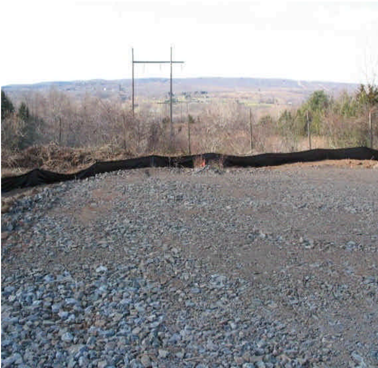
New silt fence installed and staging area in place along the ROW off Little Ln. (to the west).
