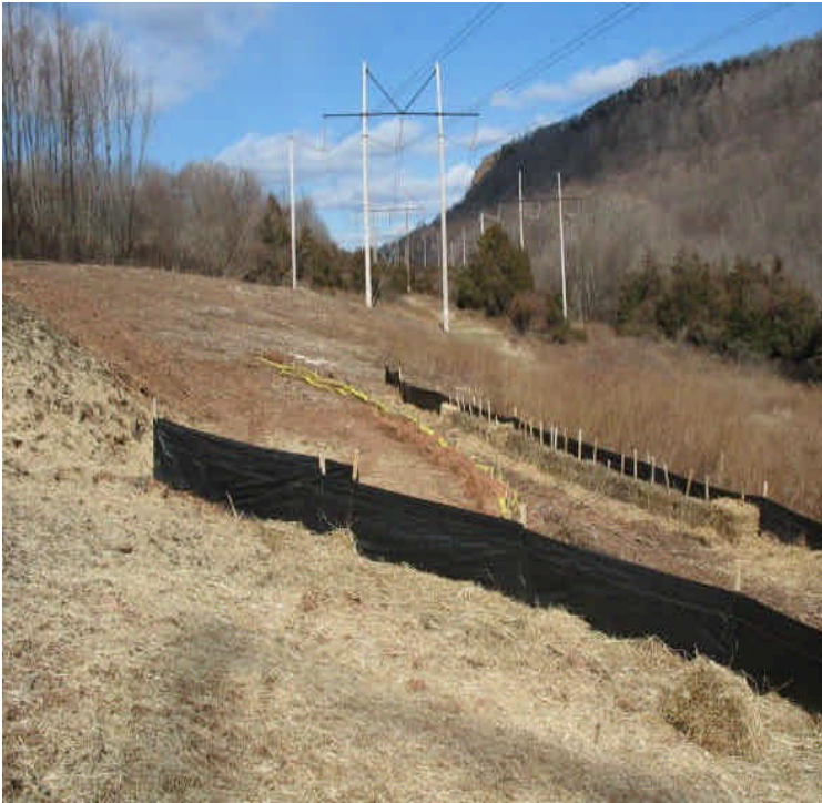
Overview of the haybales, silt fence, and filter socks at Black Pond. Mulch remains in place around the site for increased stabilization.
