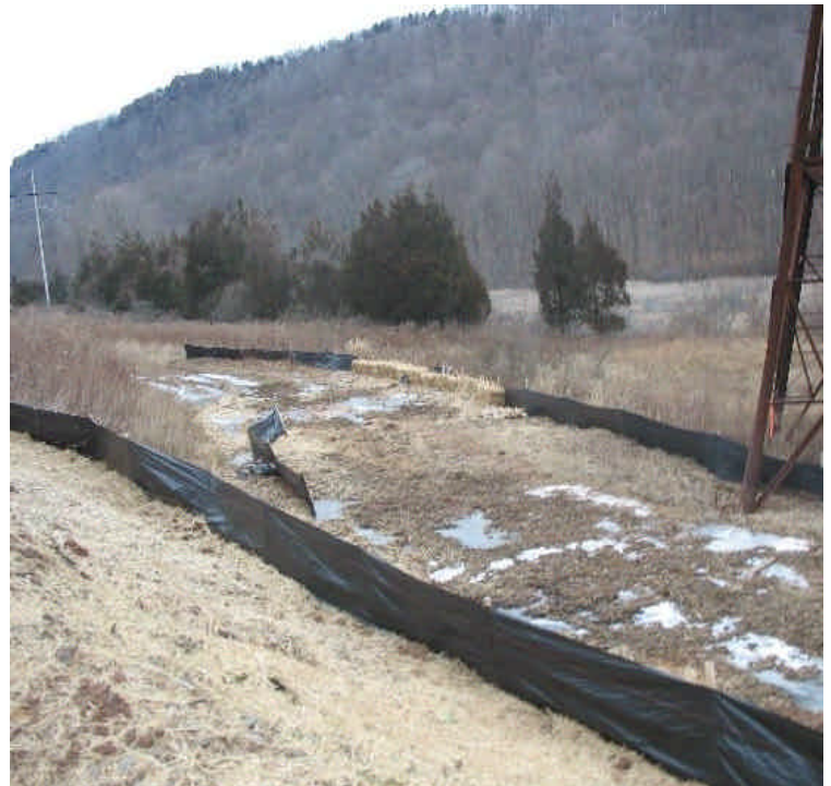
Silt fence and haybales are in place upgradient of wetlands at Black Pond.
