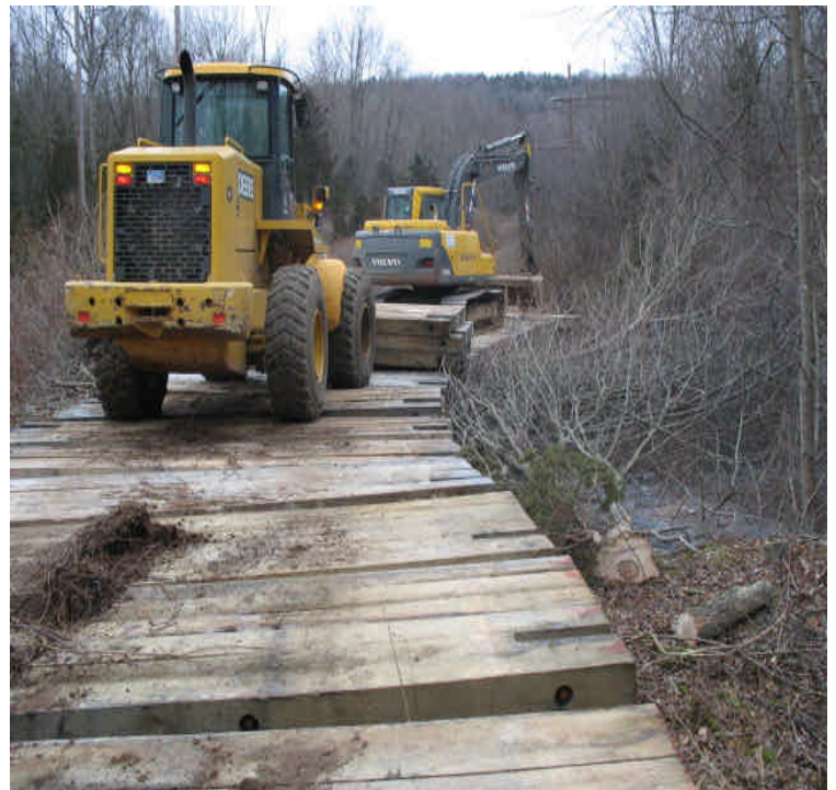
Wetland crossing construction continues west of Powder Hill Rd. The stream will be crossed later in week. Monitor for sedimentation and adjust controls as needed.
