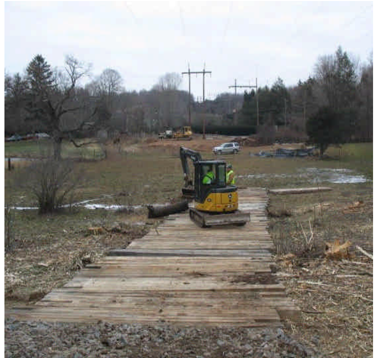
ROW extension connecting Rt. 17 with Little Lane. Timber mats and a culvert are being used to cross the wetland and a stream.
