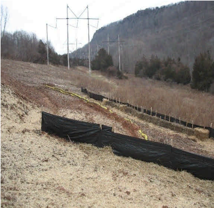
Overview of the haybales, silt fence, and filter socks at Black Pond. Mulch remains in place around the site for increased stabilization.
