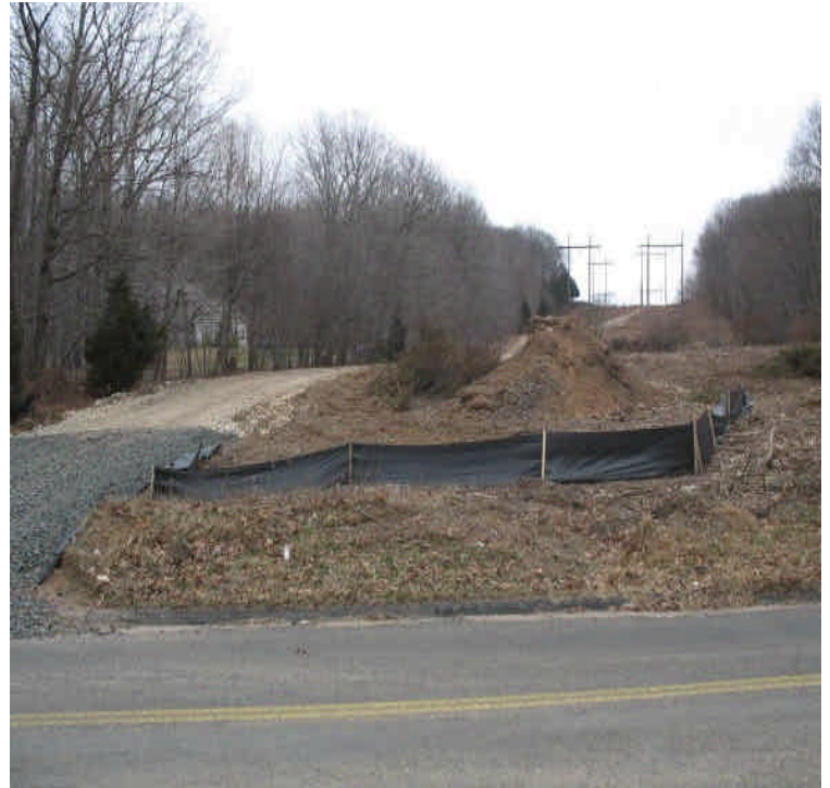
Access road and ROW off Arbutus Street. No run-off was noted during the inspection.
