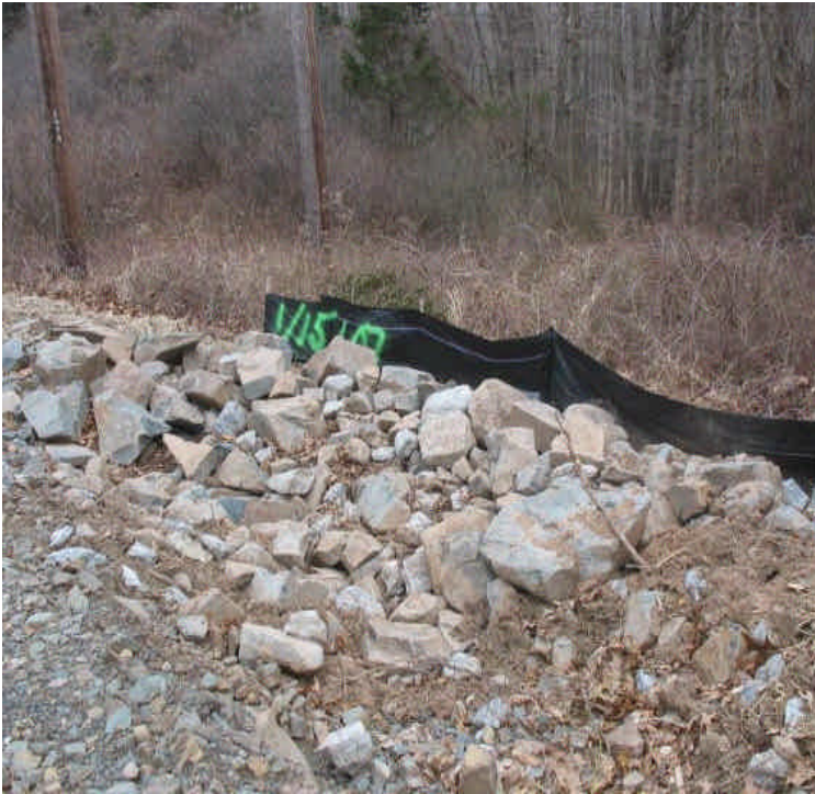
Riprap sediment trap and silt fence along the access road off Black Walnut Drive remains clear of sediment and controls are intact.
