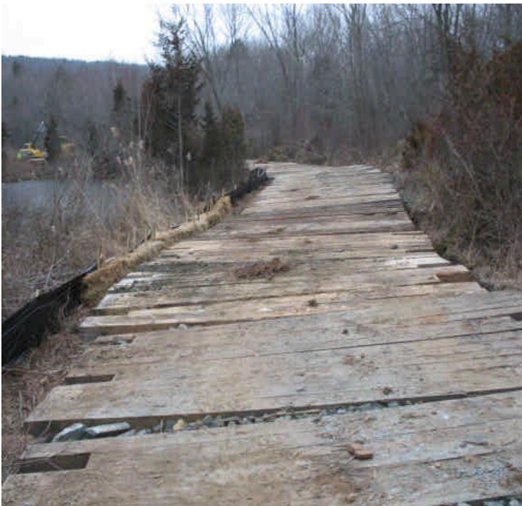
View of a low, saturated spot at the timber mats crossing in the wetlands located west of Powder Hill Rd. Haybales are in place for further control and timber mats have added support. Minor sedimentation was noted leaving the site in this area.
