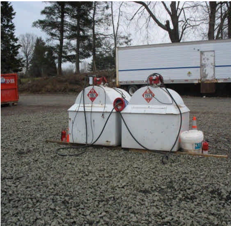
New location, stone spill pad, and handle containment for the fuel storage tanks at the contractor receiving yard. Spill kits and fire extinguishers were also added.
