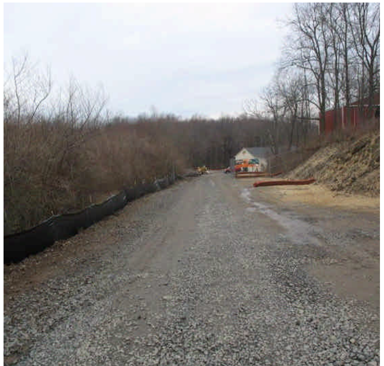
Silt fence, fiber rolls, and hay mulch have been added upgradient of wetland areas adjacent to the contractor receiving yard.
