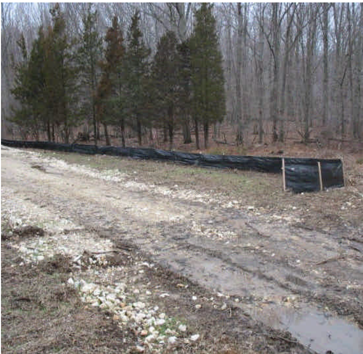
Access road off Haddam Quarter Rd. Clear water was leaving the site, filtered by existing controls.
