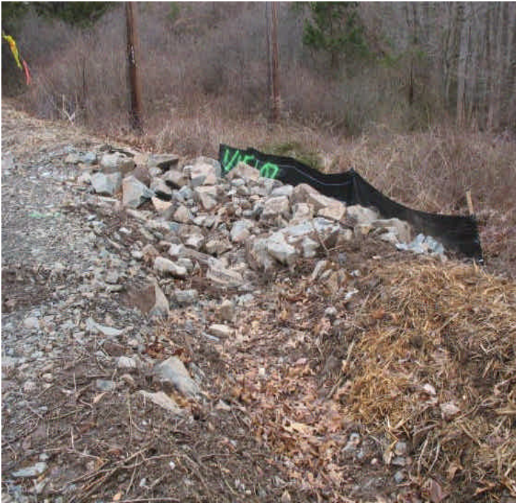
Riprap sediment trap and silt fence along the access road off Black Walnut Drive. Accumulated sediment has been removed and silt fence was repaired.
