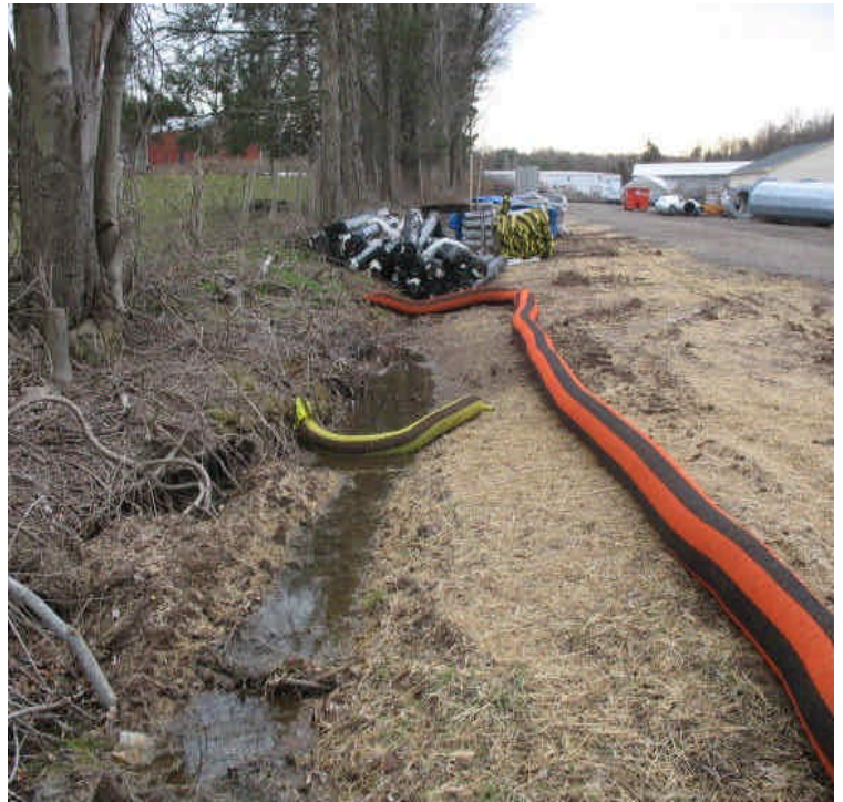
Additional controls were also added to drainage areas/swales at the contractor receiving yard.
