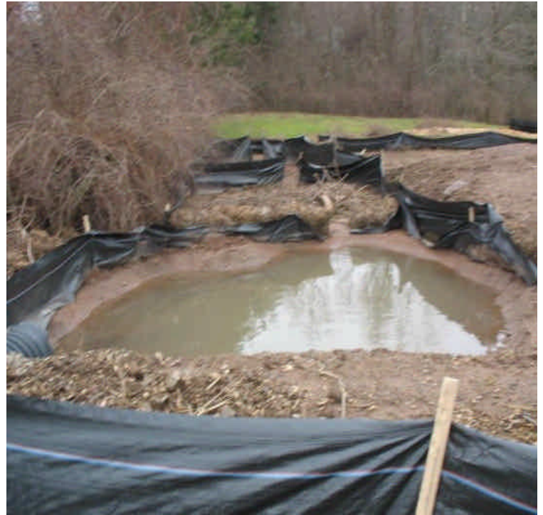
Some run-off was noted in the swale adjacent to the foundation in the ROW north of the contractor yard along Rte 17. The stormwater flows to the slurry holding areas where it remains contained.
