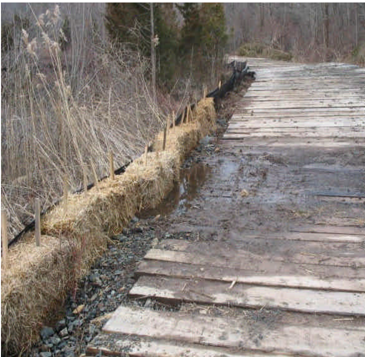
View of a low, saturated spot at the timber mats crossing in the wetlands located west of Powder Hill Rd. Haybales are in place for further control. Continue to monitor and adjust when the road is active.
